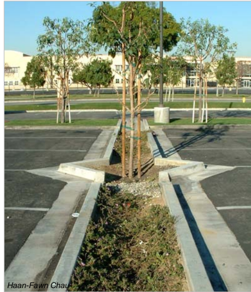
Vegetated swale with curb cuts at a shopping center. 8500 Firestone Blvd., Downey, CA.
