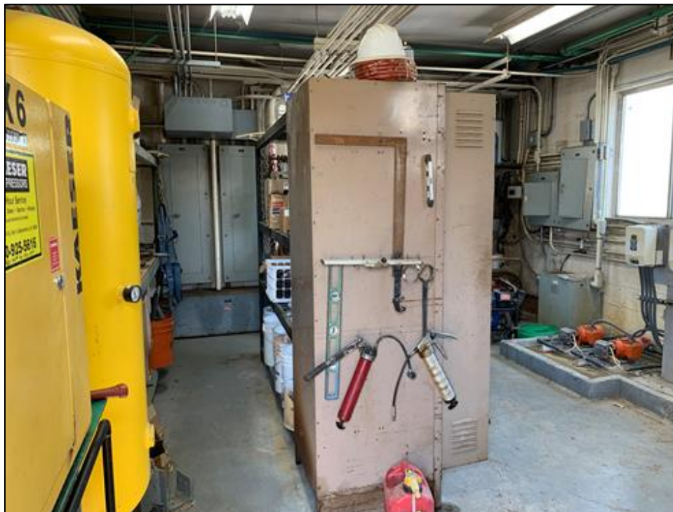
Photograph 24: Digestion control room interior, September 15, 2022.
