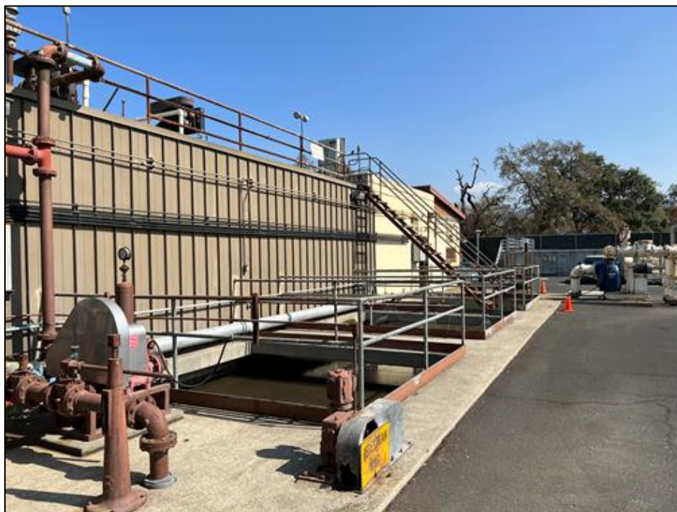
Photograph 10: Clarifier tanks in front of sludge digester, camera facing northeast, September 15, 2022.
