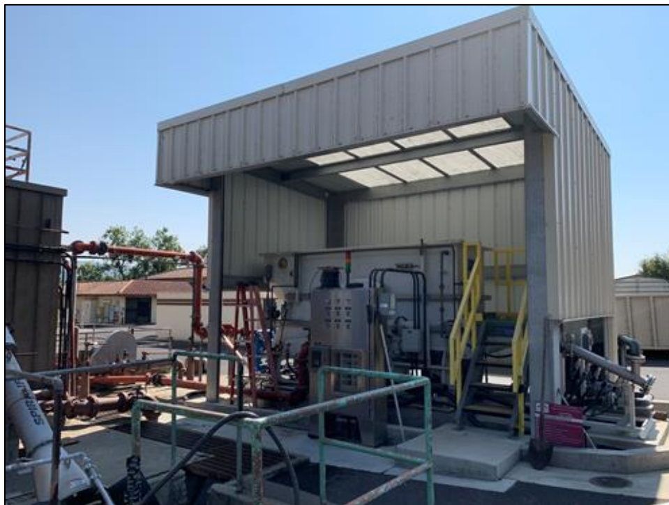
Photograph 9: Dissolved air flotation system, camera facing southeast, September 15, 2022.
