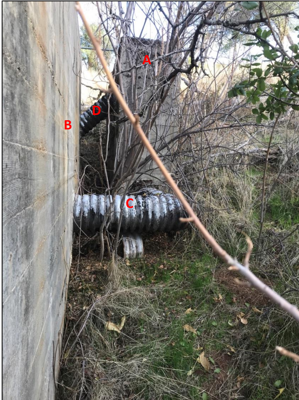
Photograph 8. Pipe connecting the Receptor Tank (A) and the Primary Processing Tank (B); heavy fraction pipe in foreground (C), light fraction pipe in background (D). View east.
