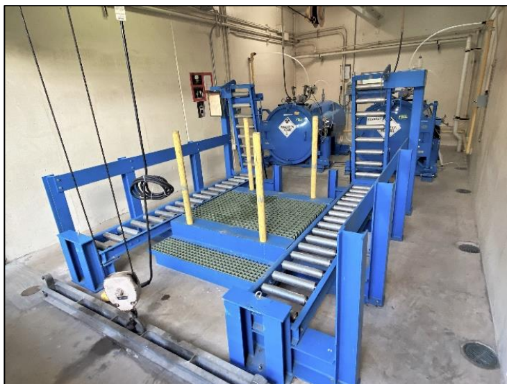
Figure 67: Two one-ton chlorine tanks within secondary containment cylinders with rolling loaders (JRP photograph, November 17, 2022).
