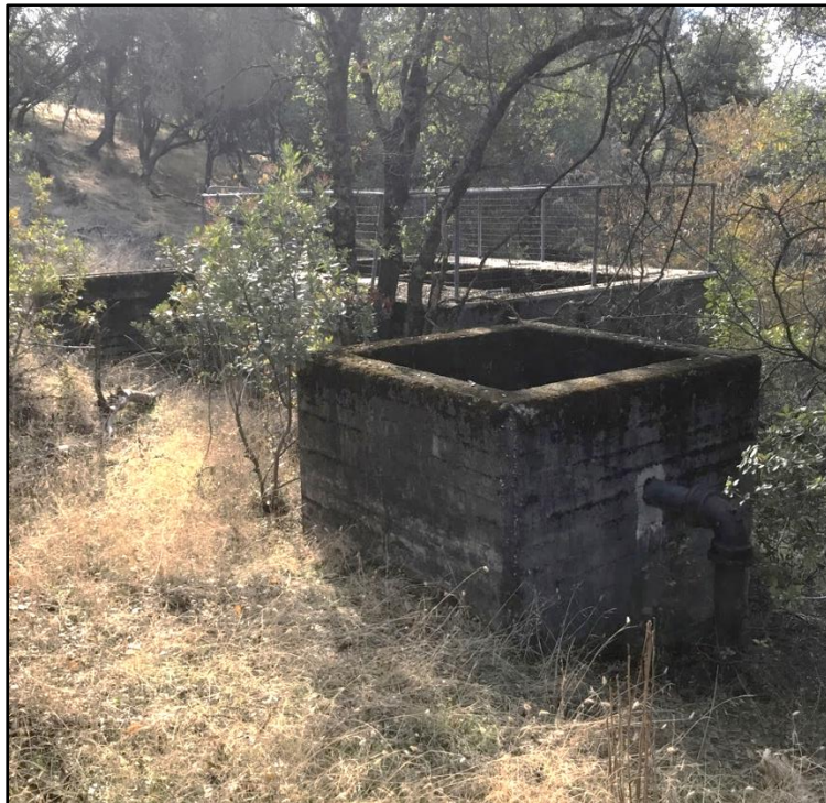
Photograph 12. Secondary Processing Tank with 6-inch diameter effluent outlet pipe exiting from north wall; Primary Processing Tank in background. View southwest.
