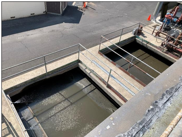
Figure 95: Primary clarifier using water spray and skimmer to separate grease layer (JRP photograph, September 15, 2022).
