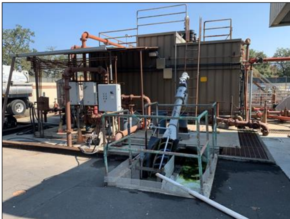
Photograph 8: Comminutor, camera facing east; September 15, 2022.
