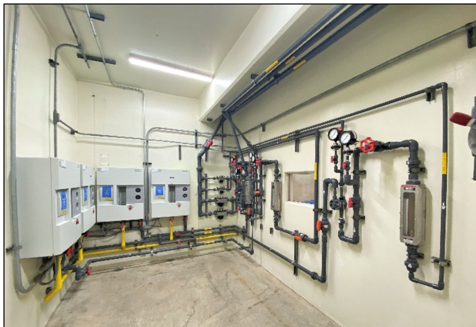
Figure 68: A chlorination feed unit with pipes and pressure gauges (JRP photograph, November 17, 2022).
