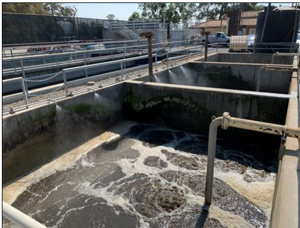
Photograph 16: Activated sludge tank, camera facing southeast, September 15, 2022.
