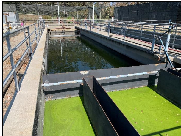
Figure 96: Final clarifier (JRP photograph, September 15, 2022).
