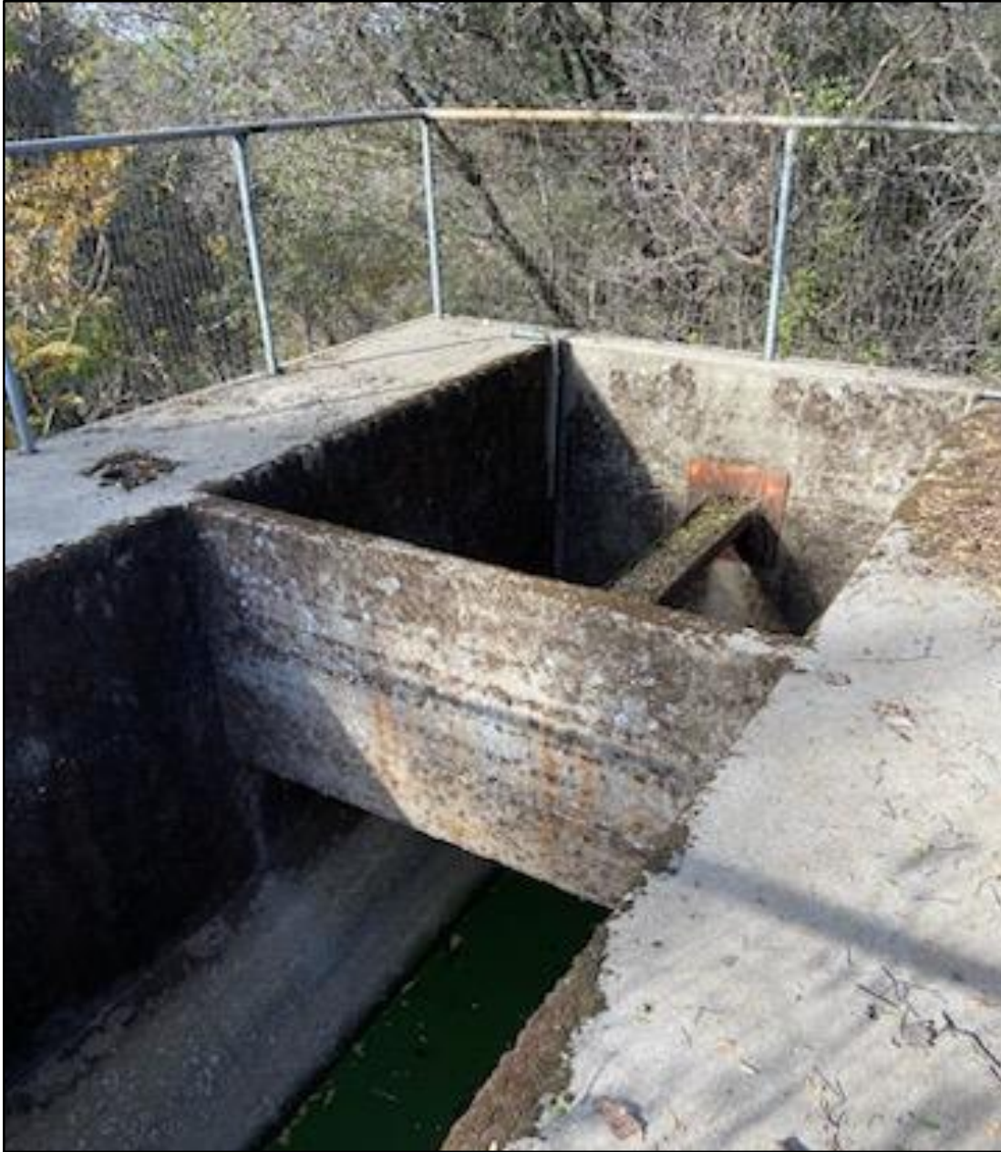
Photograph 10. Primary Processing Tank, with upper open chamber flanked by the closed lower chamber. Upper chamber has a baffle in the center and a trough extending to the wall and outlet to a Secondary Processing Tank. View northwest.
