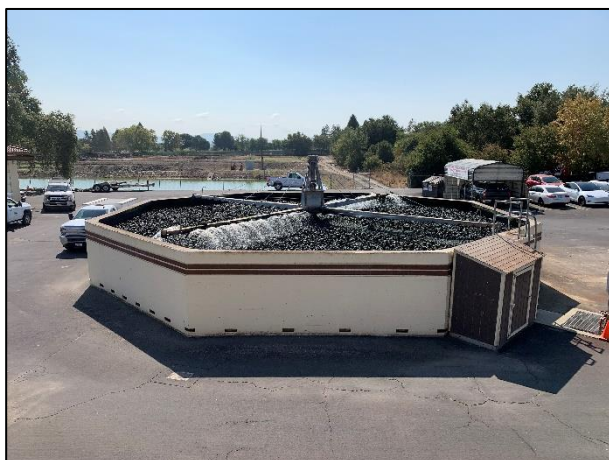
Figure 97: An octagonal trickling filter present a modest variation on the usual circular form (JRP photograph, September 15, 2022).
