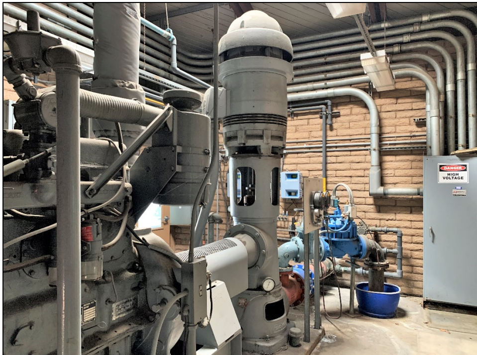
Figure 65: City of Pleasanton Well No. 6 shows a bullet-shaped motor atop the well head, a natural-gas reserve generator at left, discharge pipe right of center, and electrical supply at image right (JRP photograph, October 13, 2022).
