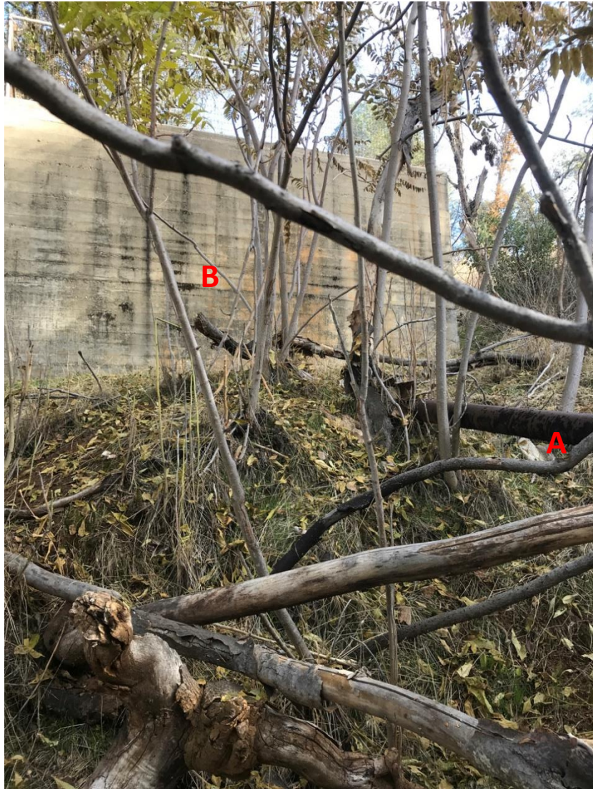
Photograph 21. Overflow Effluent Pipe (A) west of Primary Processing Tank (B). View southeast.
