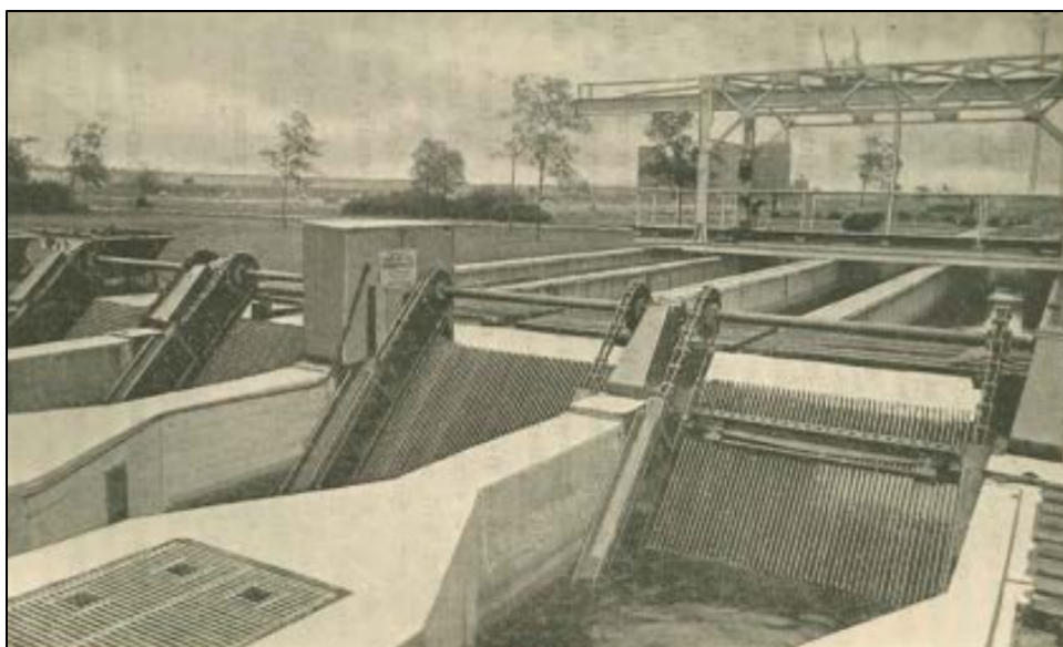
Figure 34: Mechanically cleaned bar screen at head of a typical sewage treatment plant. 212
