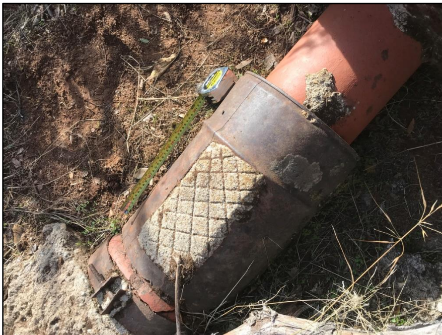
Photograph 7. Eastern intake pipe at entrance to Receptor Tank.
