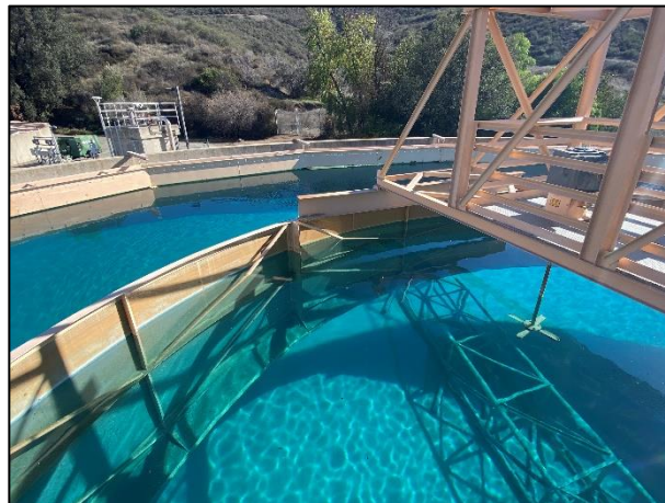
Figure 74: Interior view of clarifier shows rake arm at bottom of tank, a mechanical fan-shaped agitator, and a baffle wall for containing the agitation zone (JRP photograph, November 17, 2022).
