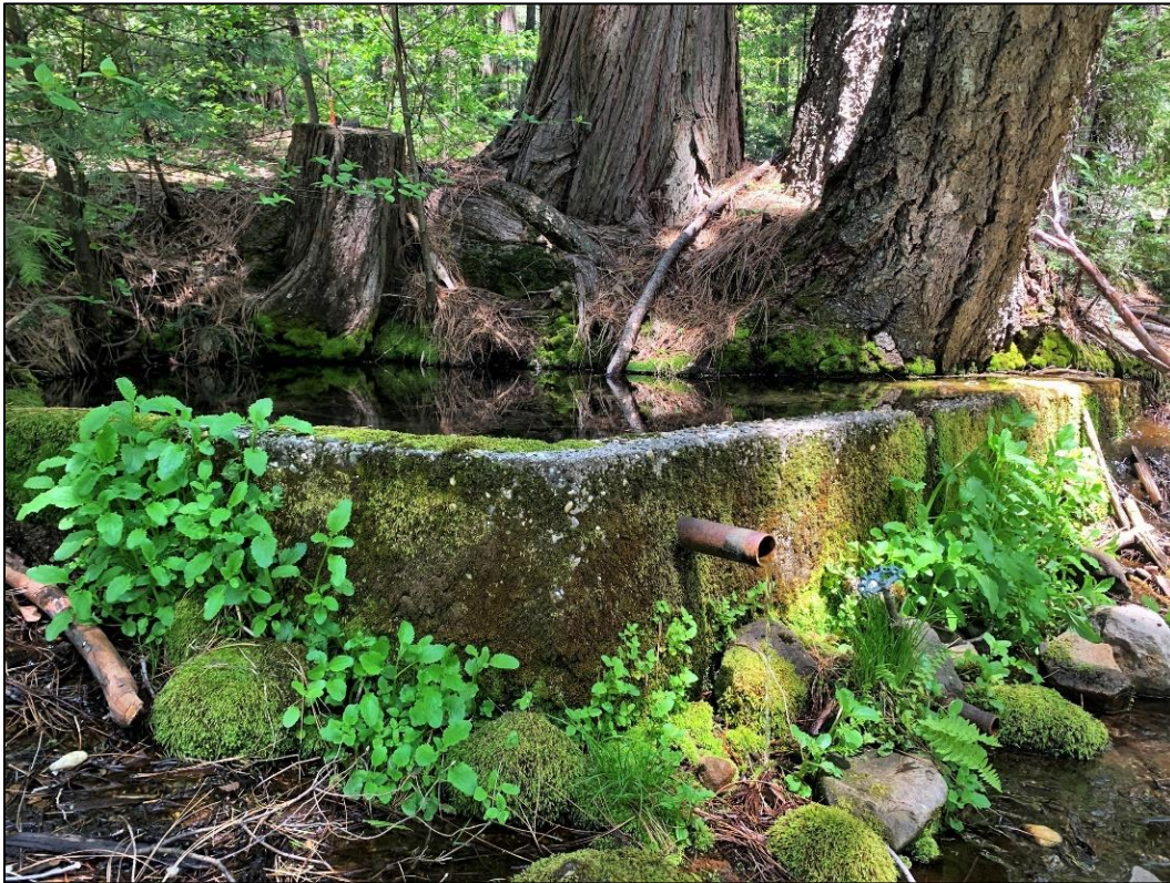
Figure 81: A 1930s-era concrete spring box captured water for a nearby labor camp in the Sierra Nevada range above Nevada City (JRP photograph May 8, 2019).
