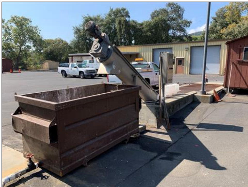
Photograph 7: Auger used grit chamber debris disposal, camera facing southwest; September 15, 2022.
