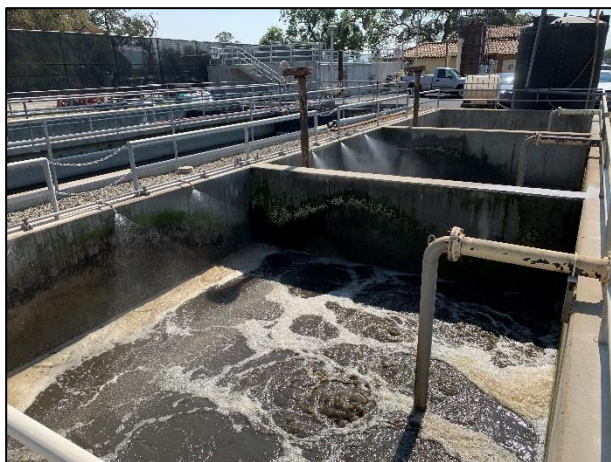
Figure 99: The typical frothy appearance of an activated sludge tank in action (JRP photograph, September 15, 2022).
