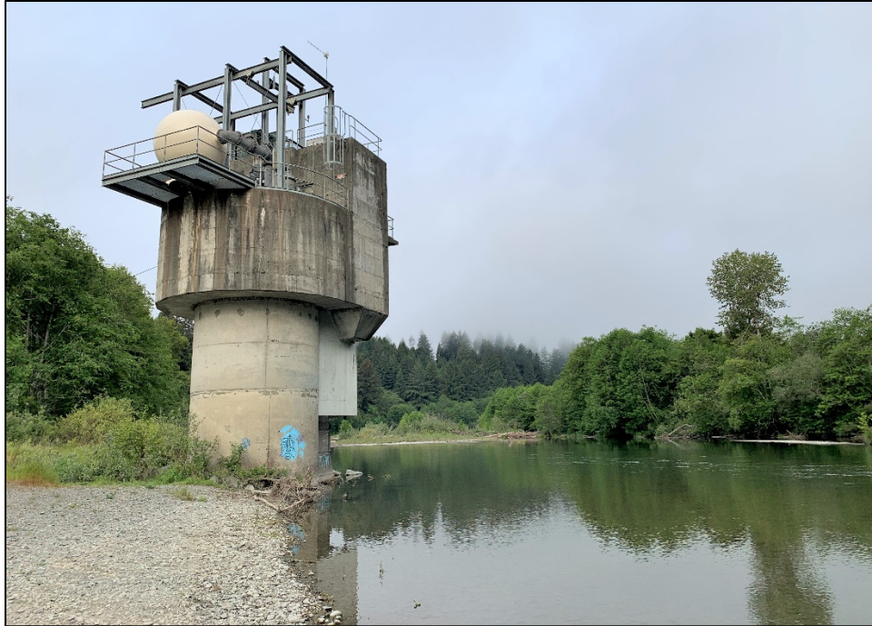
Figure 85: A pumping station for below-surface gallery collection along the Mad River in Humboldt County (JRP photograph, May 27, 2022).
