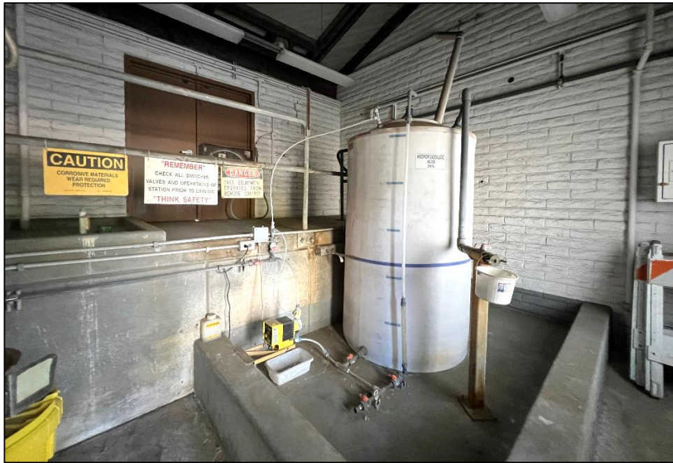
Photograph 11: Fluoridation room showing storage tank and dosing unit in front of loading dock; facing southeast, October 13, 2022.
