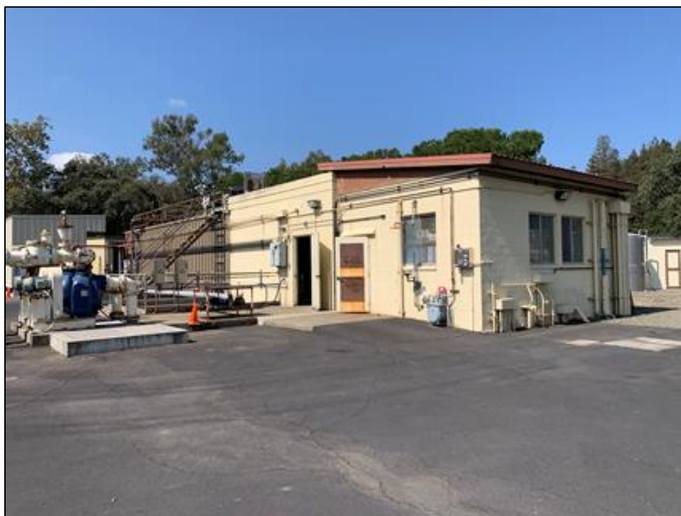
Photograph 23: Control rooms at east end of sludge digester, camera facing northwest, September 15, 2022.
