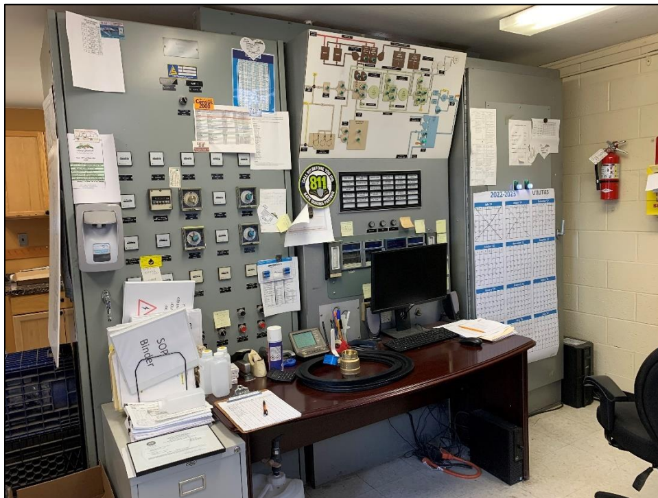
Photograph 5: Control console in office wing of control building, camera facing west, September 15, 2022.
