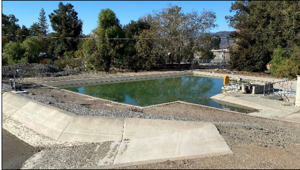
Figure 77: A sludge drying bed. Note the rampways providing access for material removal after drying (JRP photograph, November 17, 2022).
