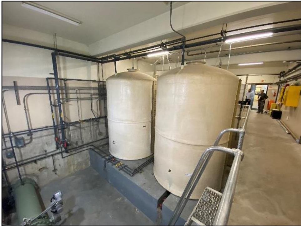
Photograph 10: Plastic storage tanks hold chemicals for injection into the raw water influent pipeline at left edge of image; November 16, 2022.
