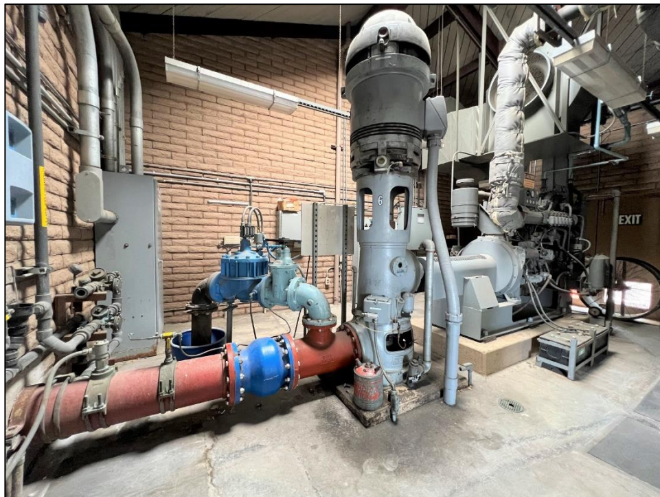
Photograph 10: Pump room with Well 6 wellhead, motor, and generator; facing northeast, October 13, 2022.
