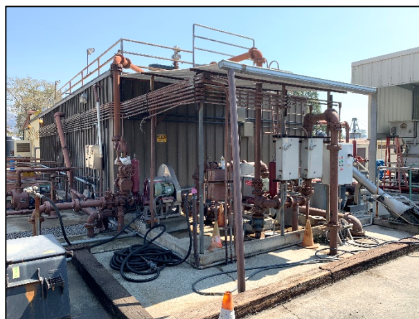
Figure 105: Rear of digestion tank showing pipe connections (JRP photograph, September 15, 2022).
