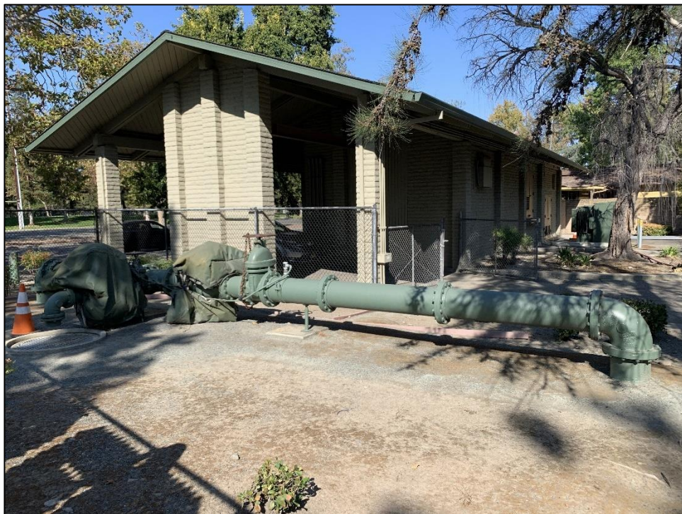
Photograph 15: Well control piping installed around 1999 south of building; facing north, October 13, 2022.
