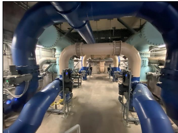
Figure 76: The pipe gallery below the filter beds has pipes labeled for backwash flow and treated water effluent (JRP photograph, November 17, 2022).
