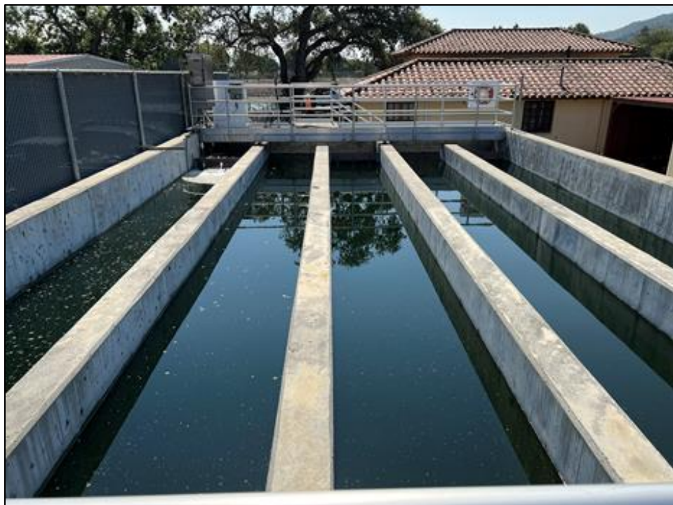
Photograph 19: Chlorine contact basin, camera facing southwest, September 15, 2022.
