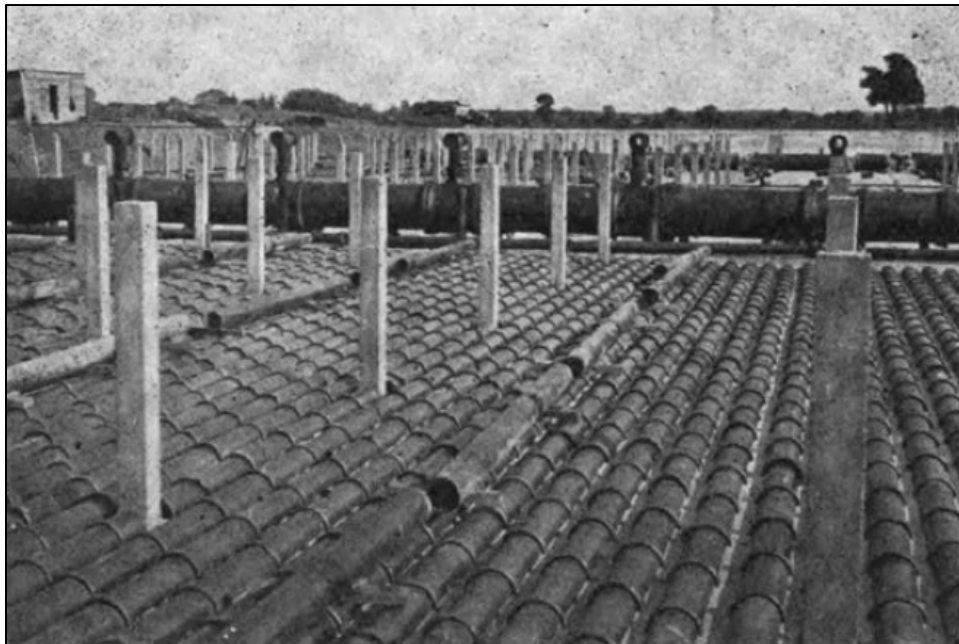
Figure 46: Trickling filter under construction, showing drainage tiles and concrete posts to hold sprinklers. Stone will later fill the bed to the top of the posts. 245
