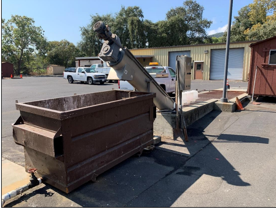
Figure 94: An auger removes materials separated by the trash rack and grit chamber, located below grade at the head of the treatment plant process (JRP photograph, September 15, 2022).
