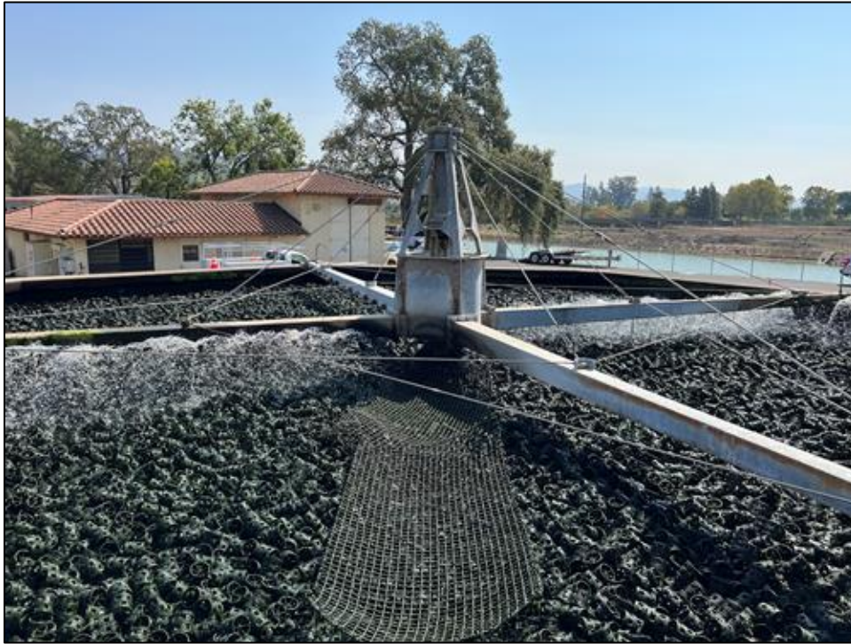
Photograph 14: Trickling filter distributor arms and plastic media, camera facing east, September 15, 2022.
