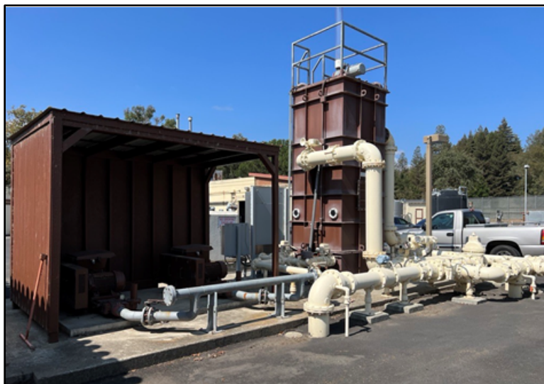
Figure 101: A pressure filter contained in a metal casing with piping for backwashing (JRP photograph, September 15, 2022).
