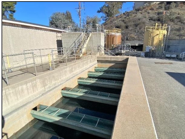
Figure 75: One of four rapid sand filter beds at the Redlands Tate plant. During normal operations, the filtering water would stand above the half-pipe troughs (JRP photograph, November 17, 2022).
