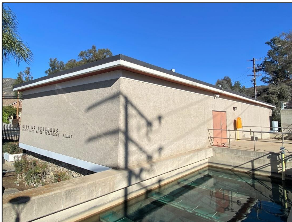
Photograph 4: Southwest control building corner with filter bed in foreground. Note the lack of column articulation on the sides and rear of building; camera facing northeast, November 16, 2022.
