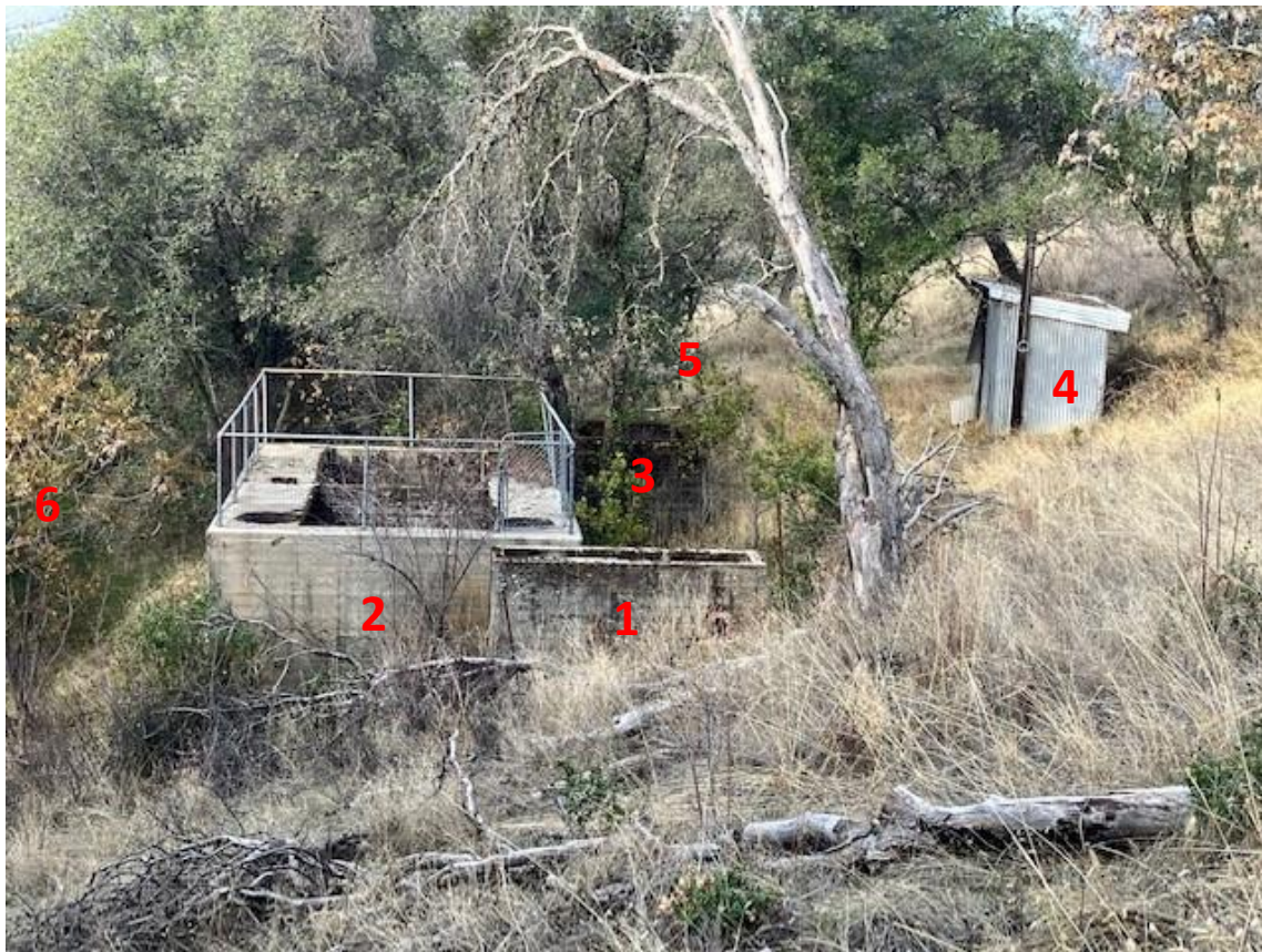
Photograph 1. Overview of treatment plant: 1) receptor tank, 2) primary processing tank, 3) square, secondary processing tank, 4) electrical shed, 5) southern end of leach field #2, 6) pond. View north.
