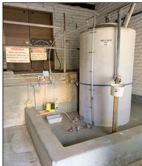
Figure 69: Fluoride in liquid hydrofluocilic form contained in a plastic storage tank and a concrete spill containment wall, with a small electric feed pump (JRP photograph, October 13, 2022).
