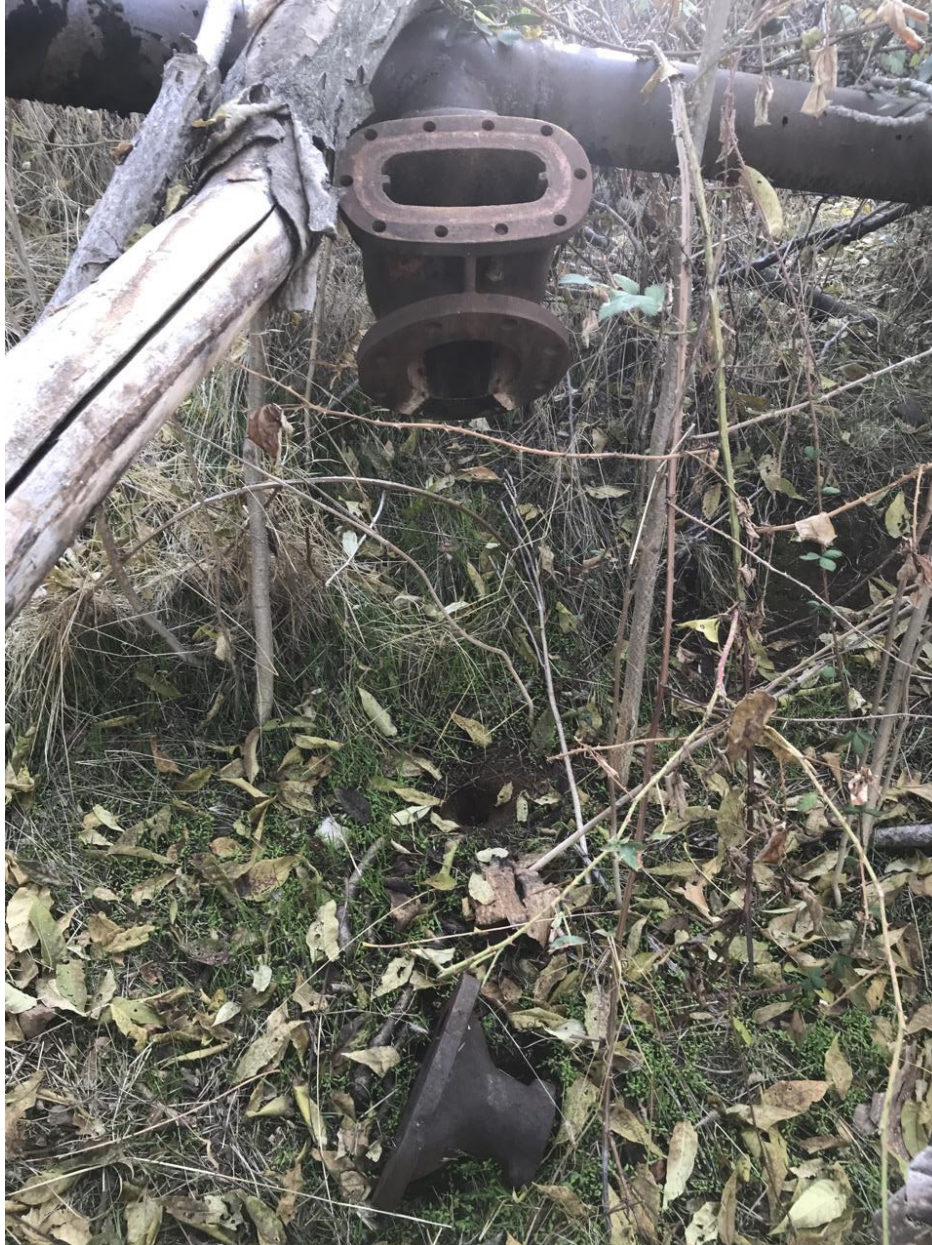
Photograph 22. Overflow pipe diffuser with reducer on ground. View south.
