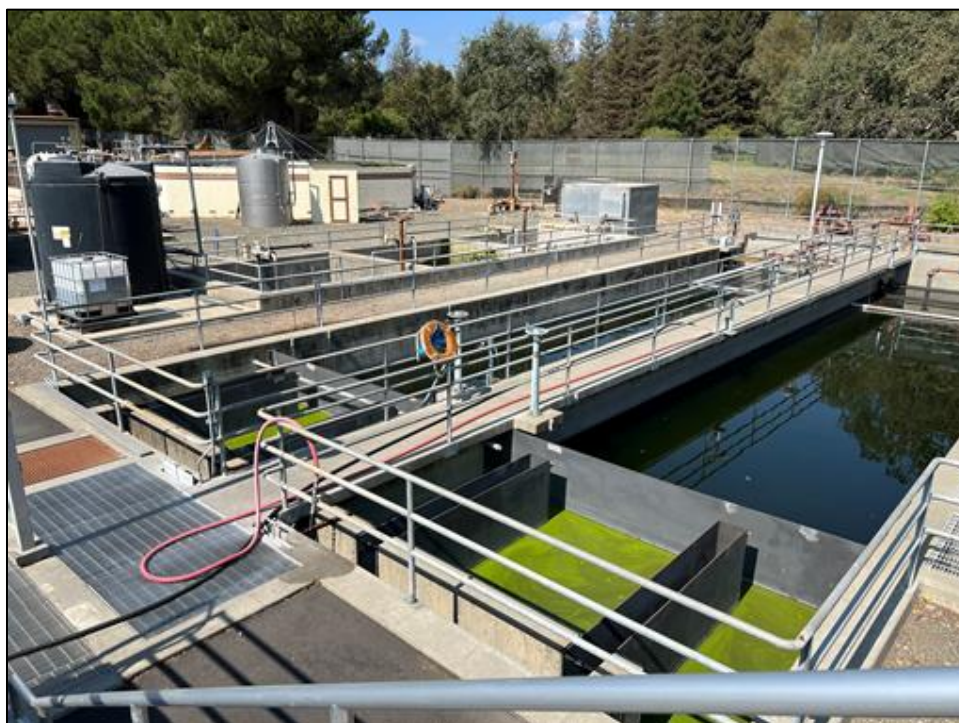
Photograph 17: Final clarifying tanks, camera facing north, September 15, 2022.
