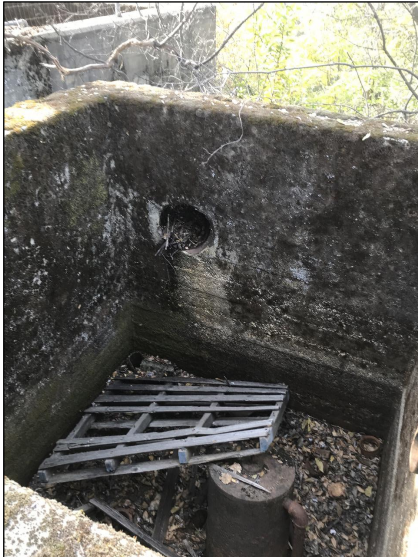
Photograph 13. Interior of Secondary Processing Tank with 12-inch diameter inlet pipe from Primary Processing Tank in west wall; pump at base of tank, along with modern pallet. View southwest.
