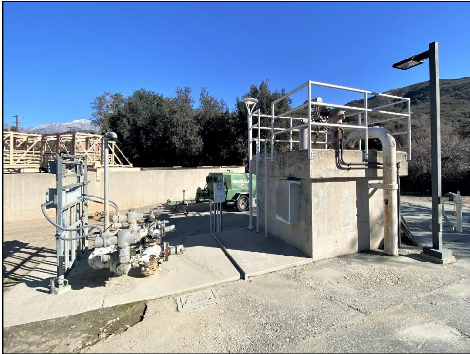
Photograph 14: A splitter box diverts water to one of two clarifiers; camera facing southeast, November 16, 2022.
