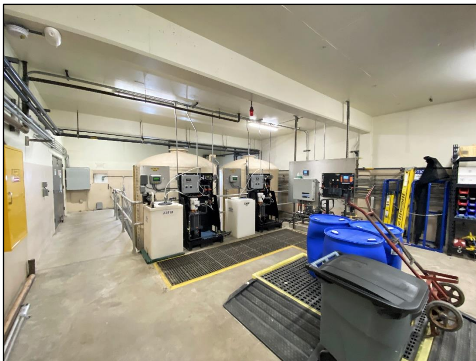
Photograph 9: Chemical dosing room at east end of control building; November 16, 2022.
