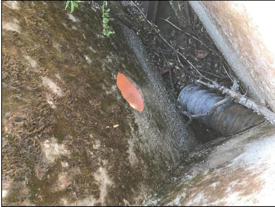
Photograph 6. Inside the Receptor Tank with entry hole from western intake pipe and corrugated pipe for eastern intake pipe.
