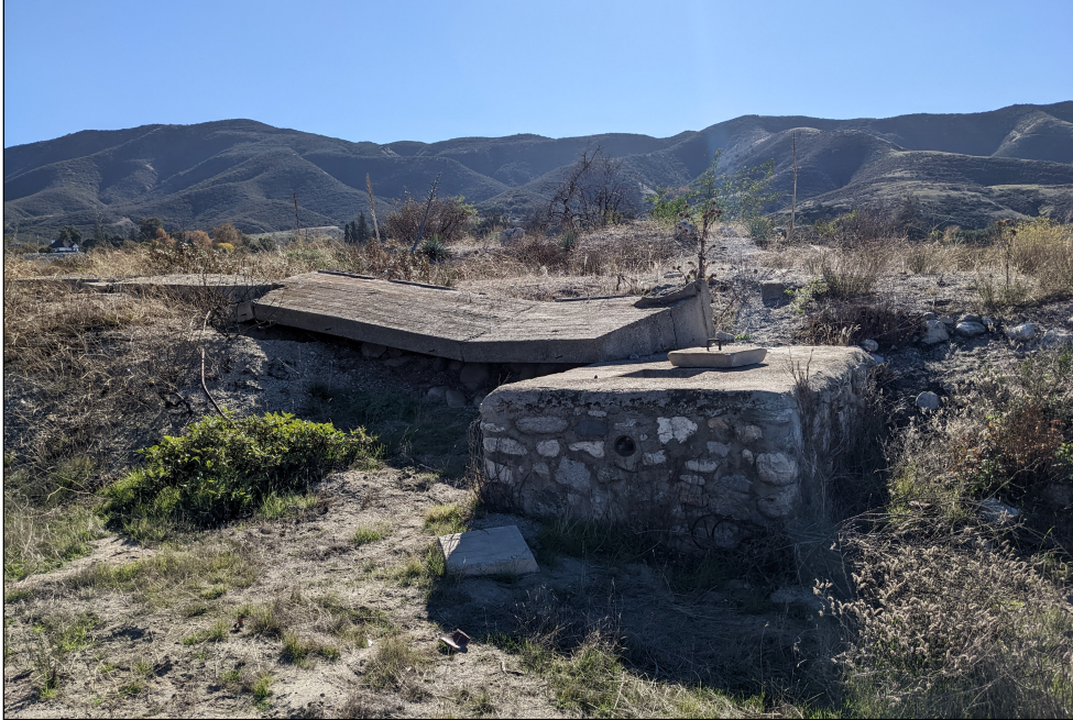
Figure 111: Overview of the filtration plant at the Mill Creek Filtration Plant, Redlands.
