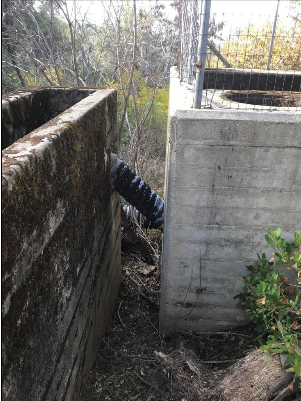
Photograph 9. Light fraction connector pipe between the Receptor Tank (left) and the Primary Processing Tank (right). View west.
