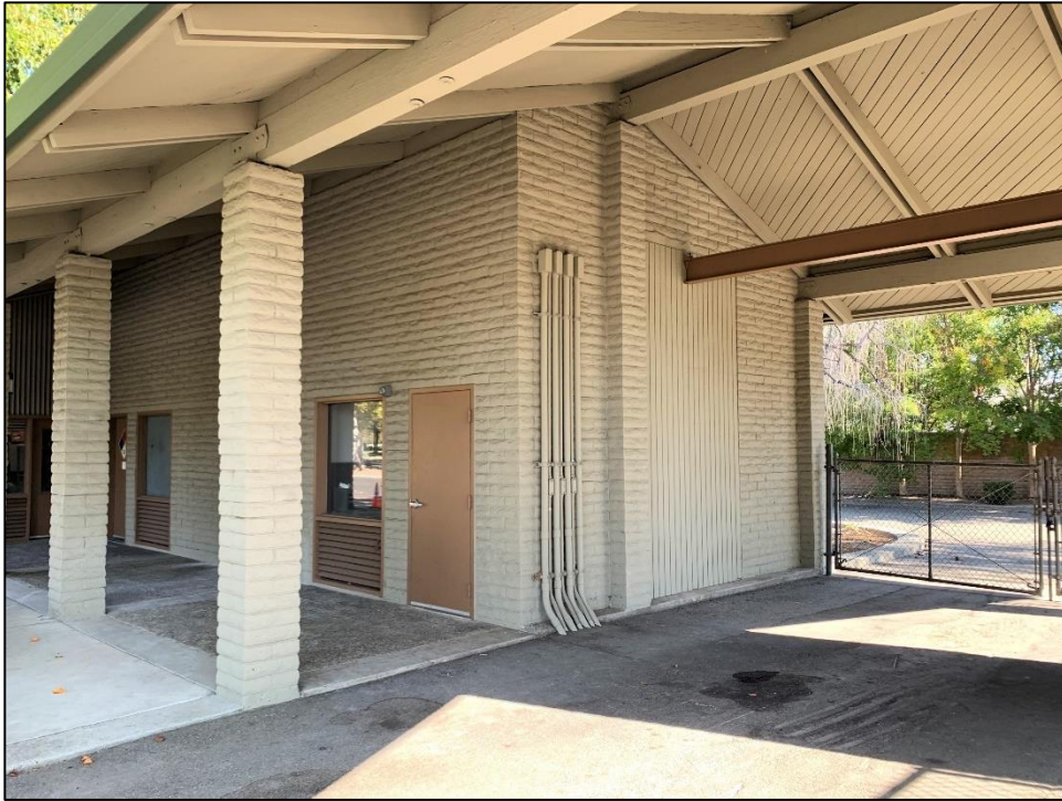
Photograph 4: View of the porte-cochère and south building side, showing exposed roof beams and sheathing; facing northeast, October 13, 2022.
