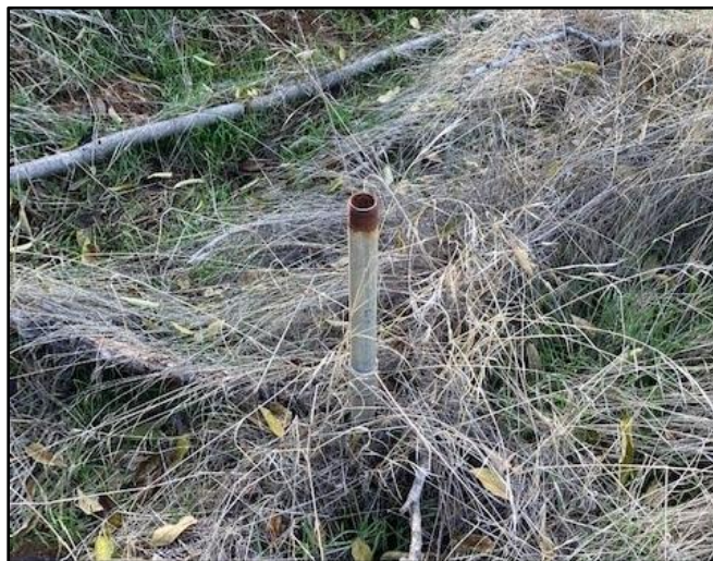
Photograph 20. Example of pipe attached to supply line pipe that filled the leach fields.
