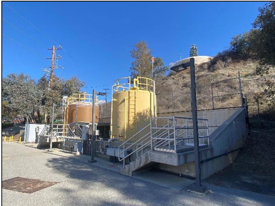
Photograph 13: Modern chemical feed and storage tanks; facing northeast, November 16, 2022.
