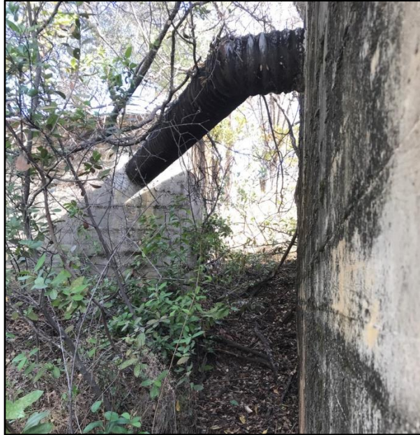
Photograph 11. Connector pipe between the Primary and Secondary Processing Tanks. View east.
