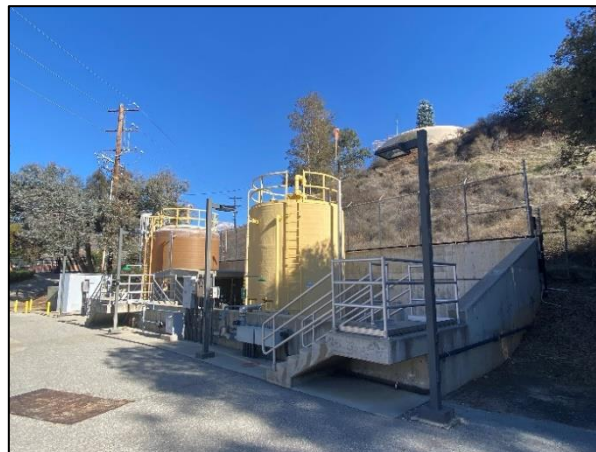
Figure 72: Chemical storage tanks (JRP photograph, November 17, 2022).
