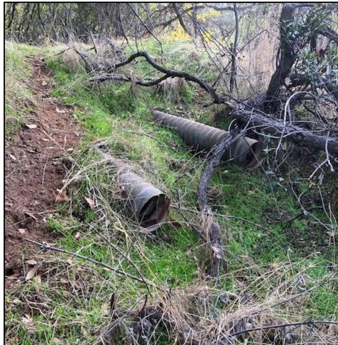
Photograph 24. Corrugated pipe exiting the northern Pond berm into Leach Field #3. View southwest.
