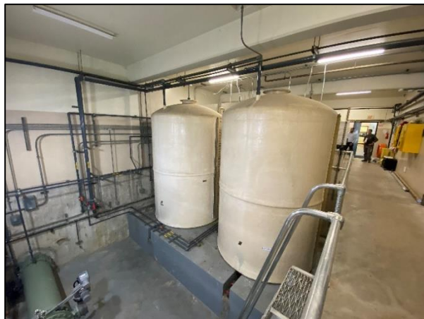
Figure 71: Plastic tanks hold chemicals for injection into the raw water influent pipeline at left edge of image (JRP photograph, November 17, 2022).
