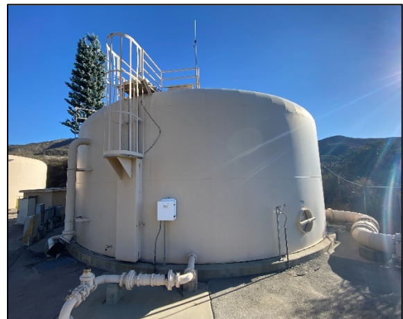
Figure 78: A steel tank for holding water for filter backwashing (JRP photograph, November 17, 2022).
