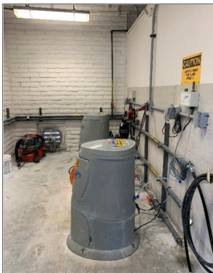
Figure 66: A modern dry chlorine feeder (JRP photograph, October 13, 2022).
