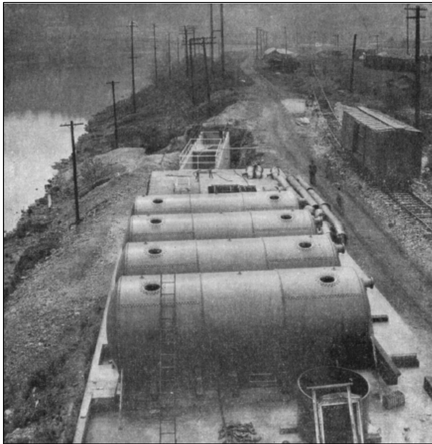
Figure 27: Zeolite water softening tanks at the Ohio Valley Water Company Plant. 189
