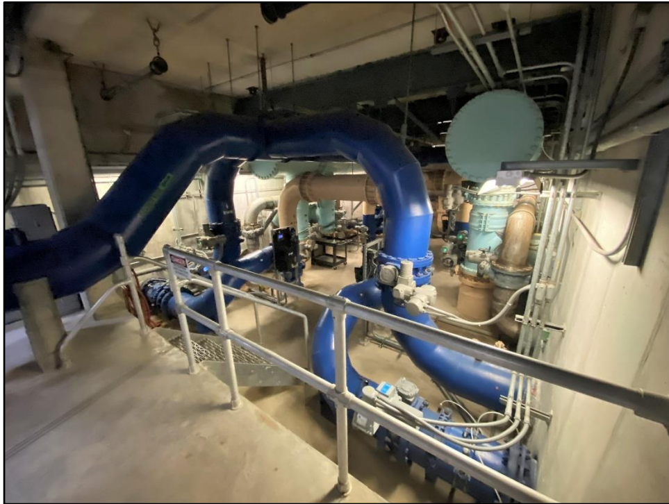
Photograph 12: Filter gallery in basement of control building; November 16, 2022.
