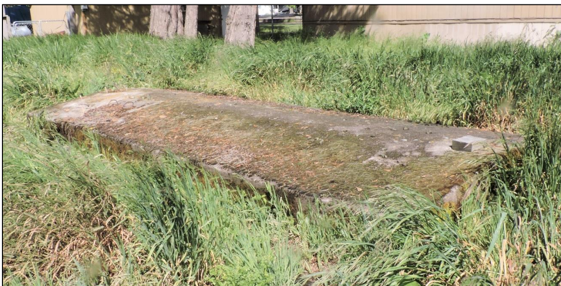
Figure 92: A concrete septic tank lid, approximately six by 20 feet, at the Mount Shasta Fish Hatchery in Siskiyou County (JRP photograph, May 22, 2019).
