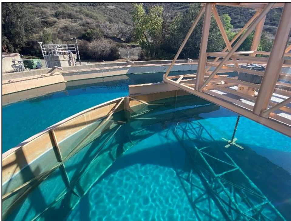
Photograph 16: Interior view of clarifier shows rake arm at bottom of tank, a mechanical fan-shaped agitator, and a baffle wall for containing the agitation zone; November 16, 2022.
