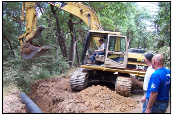
Workers install a properly sized culvert to capture water emanating from steep slopes above this rural road and direct it to a location protected from erosion.
