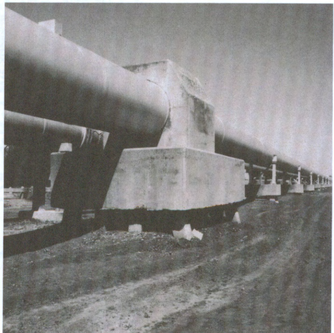
Land subsidence on Orwood Tract is exposing piles supporting the East Bay Municipal Utility District Aqueduct. These piles extend deep into the ground to assure continued stability.
