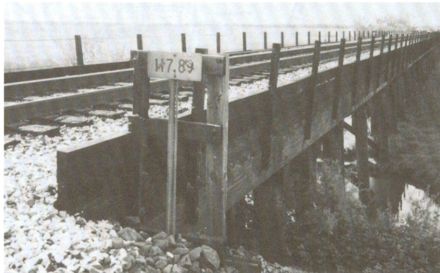
A raised section of the Union Pacific Railroad line northeast of McCormack-Williamson Tract.
