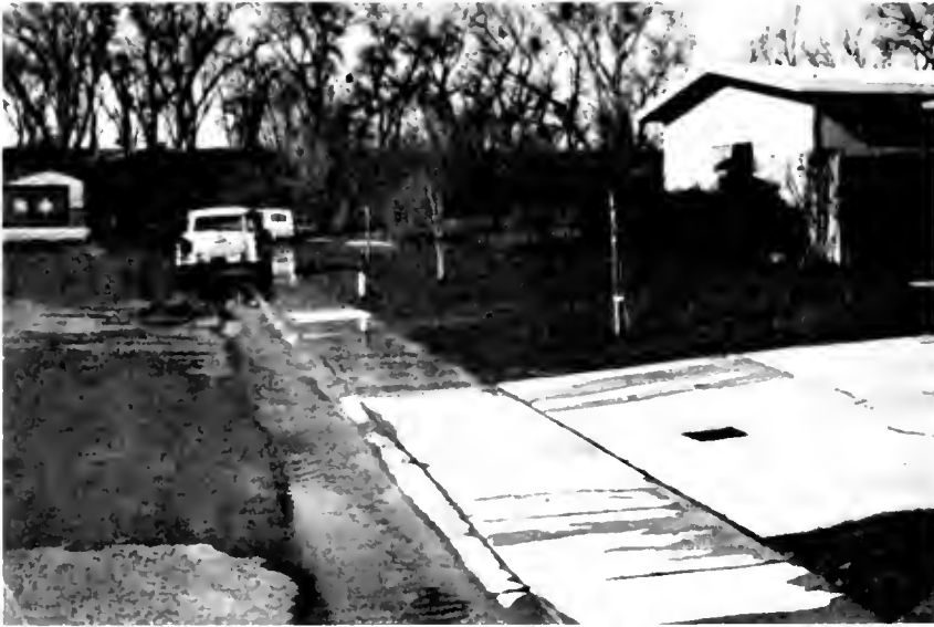
(Location 1) Seepage flowing through sidewalks and lawns along Riverview court.
