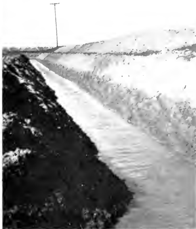
Seepage flowing down the cut-bank of drainage ditch about 1/2 mile away from the Sacramento River on the River Farms property north of Knights Landing.
