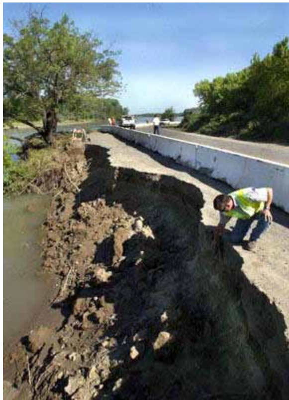
Erosion along the Sacramento River
