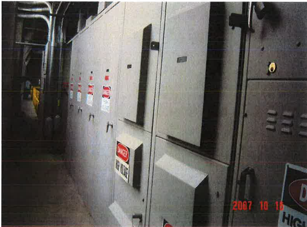
Figure 5-2 Switchgear 1 and Switchgear 2 Back View
