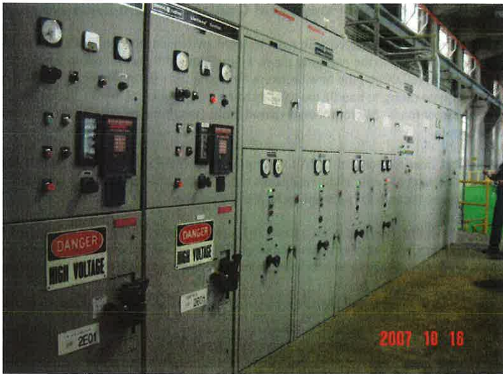
Figure 5-1 Switchgear 1 and Switchgear 2 Front View
