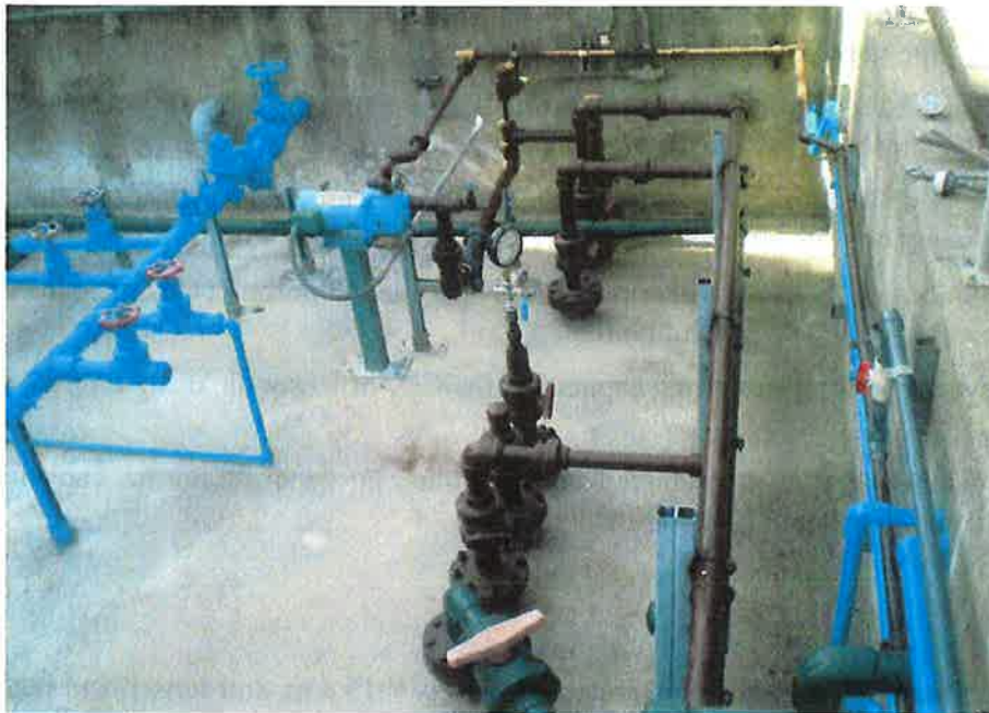
Photograph 5. Gage/data logger in SJWD chemical feed vault
