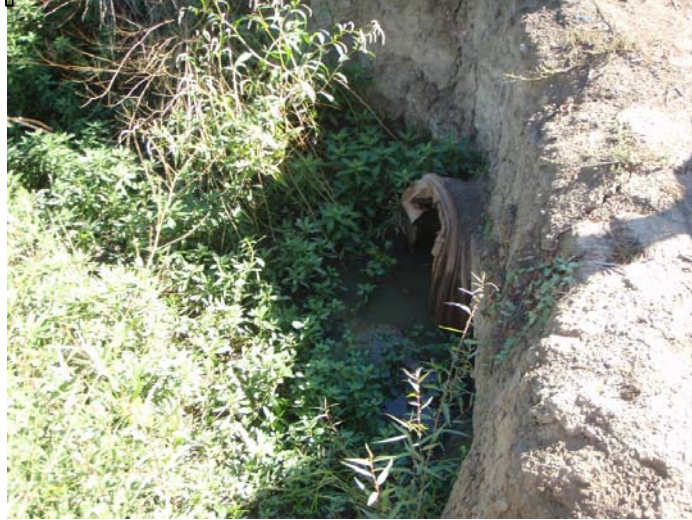
Figure 26. A culvert and unimproved road crossing in the Tule Canal. Photo by Dave Vogel.
