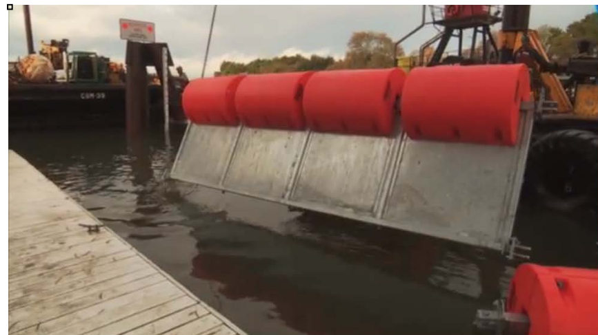
Figure 31. Floating wall being installed near the entrance to Georgiana Slough in 2014 (screen capture from: http://www.youtube.com/watch?v=937bXx9QMn8&feature=youtu.be )
