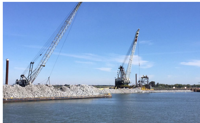
The State installed a salinity drought barrier to stop the encroachment of saline waters into the Sacramento-San Joaquin Delta due to the lack of freshwater flows.
