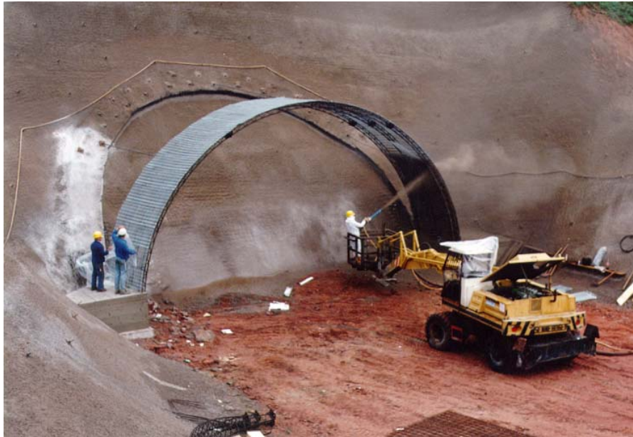
Figure 9-19 Shotcrete Canopy Construction after Completion of Portal Collar and Pre-support (Schürzeberg Tunnel, Germany)
