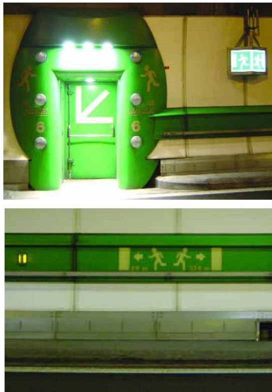
Figure 1-12 Emergency Exit (FHWA, 2006)
