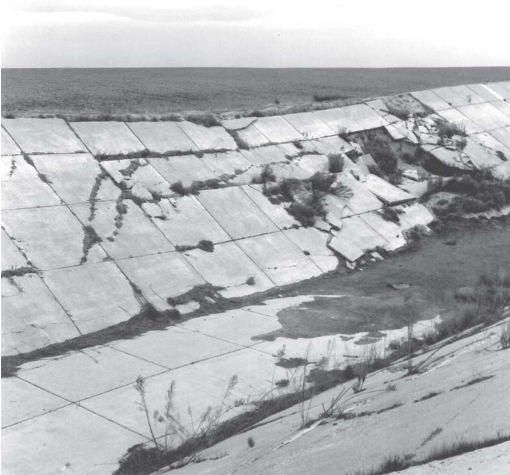
Figure 7.—Severe damage to the test section of an aqueduct similar to the California Aqueduct. The damage was caused by shallow subsidence in an area of Panoche loam, subsided, 0 to 5 percent slopes.
