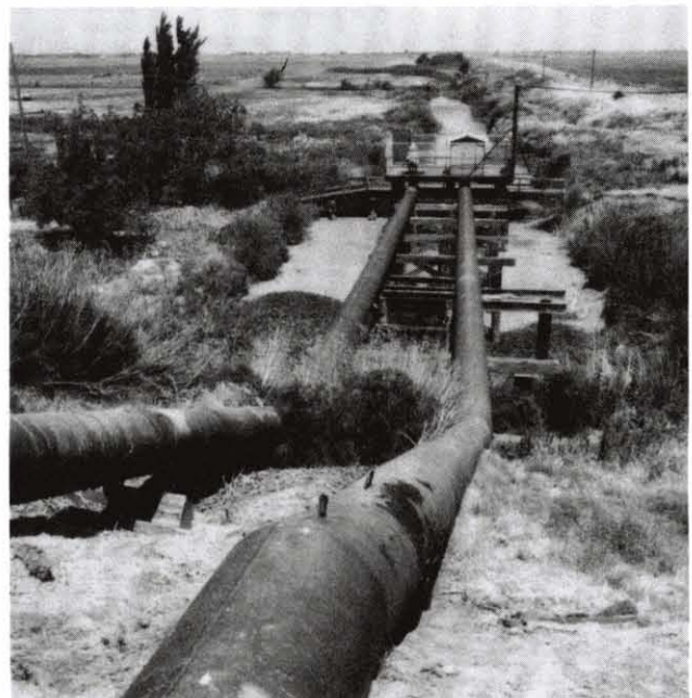
Agricultural drainage pipes on Twitchell Island. (The water is lifted approximately 20 feet to flow into the San Joaquin River.)
