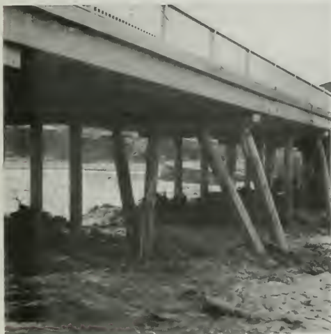
Figure 382. Flood Damage to Lake Hughes Road Bridge
