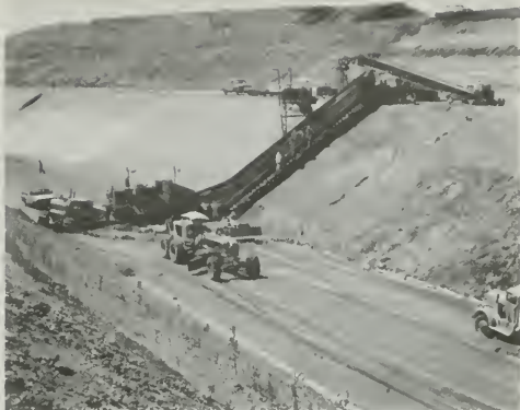
Figure 158. Placing Type II Drain Pipe Along Toe of Slope and Type B Filter Material on Invert of Power Canal
