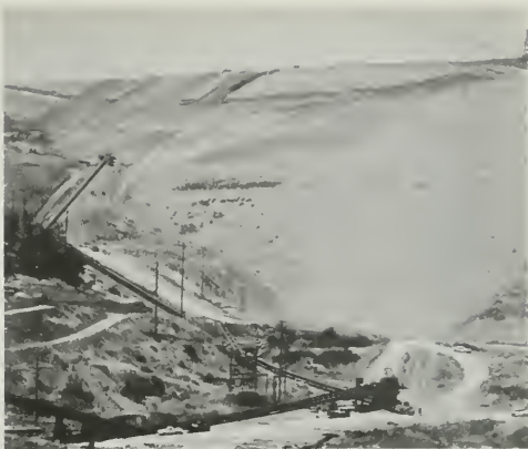
Figure 112. Distribution Conveyors on Right Abutment
