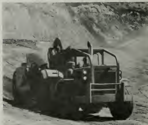
Figure 388. Scraper Spreading First Load of Embankment in First Approved Dam Foundation Area
