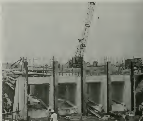
Figure 168. Sutter-Butte Canal Outlet Conduits
