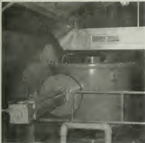
Figure 316. 42-Inch-Diameter Shutoff Valve
