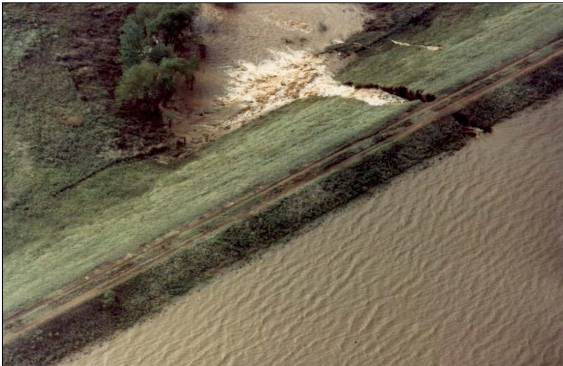
Figure 3-5.—Upper Red Rock Site 20 Dam internal erosion through dispersive soils.
