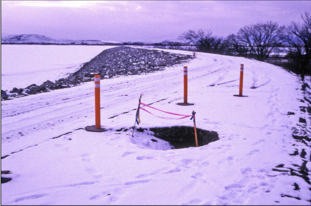
Figure 3-15a.—Sinkhole in crest of a dam in Montana.
