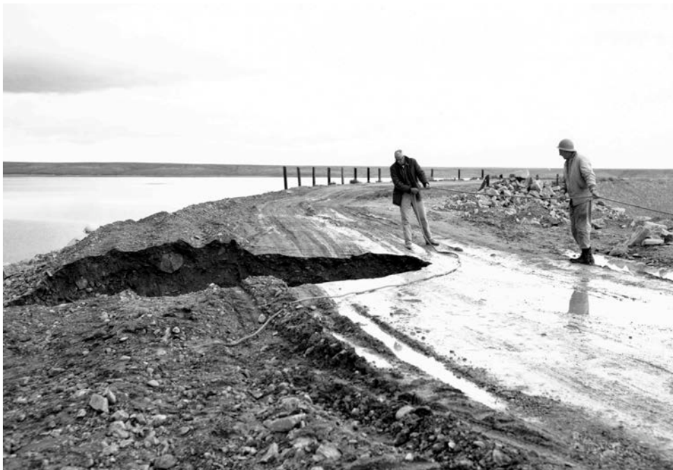
Figure 4a.—20-ft-diameter sinkhole on upstream side of dam crest. (Standing near the edge of a large sinkhole while hanging onto a rope is considered extremely dangerous and is not recommended.)
