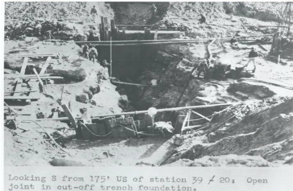
Figure 3.—Solutioned dolomite observed in cutoff trench.
