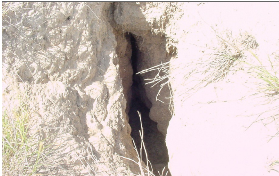
Figure 2.—Large crack in embankment, Olmitos-Garcias No. 2 Dam.
