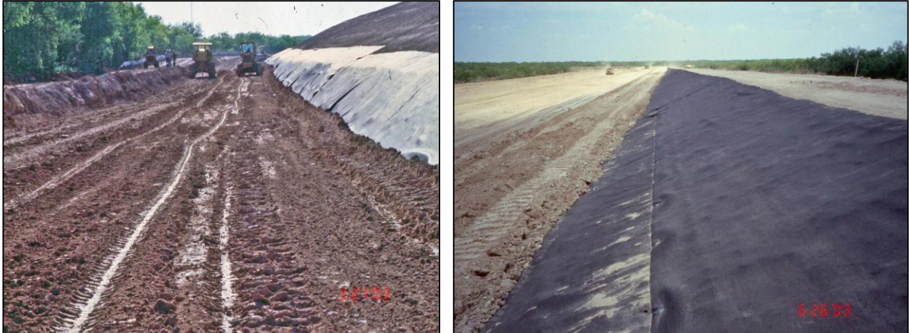
Figure 10-18.—Construction of geotextile barrier in Olmitos-Garcias No. 2 Dam in south Texas. The downstream side of the embankment is shown. Left – geotextile being backfilled in foundation trench. Right – geotextile on back slope of dam prior to backfilling. (Photos courtesy of NRCS, Texas)
