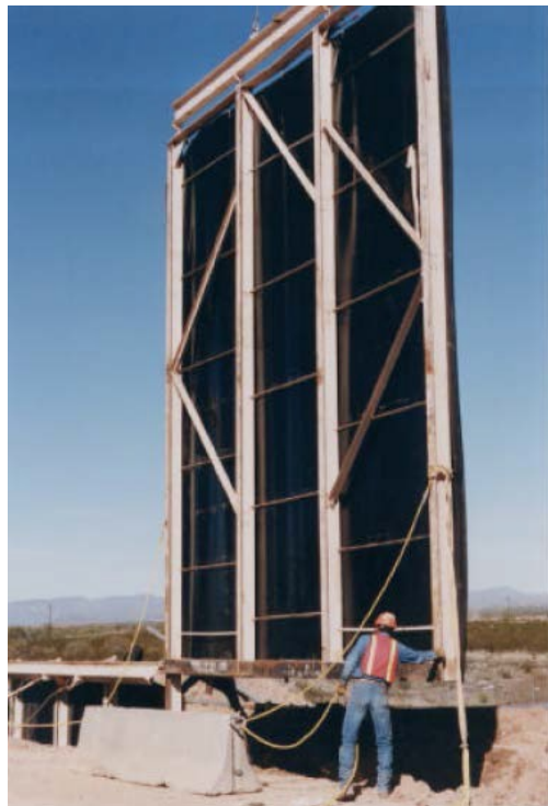
Figure 9.—Installation of geomembrane panel in the trench adjacent to previously placed panel.
