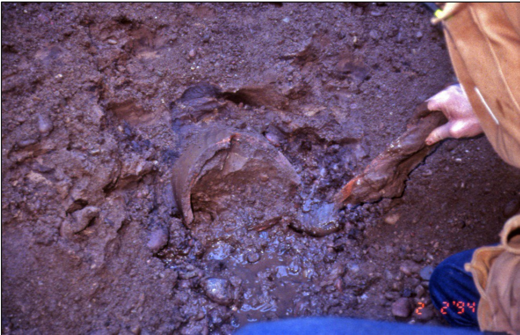
Figure 3-15b.—Excavation of the sinkhole shown in previous photograph revealed original toe drain below the sinkhole.
