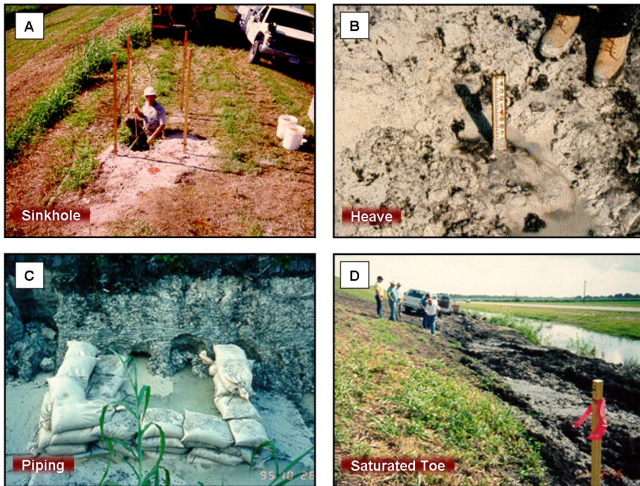
Figure 3.—Representative photographs of prior seepage erosion conditions at HHD near Lake Harbor. Downstream area seepage distresses were observed during events having a ~30-yr return period: (A) sinkhole formation in crest, (B) heave of downstream toe caused by upward seepage flow - surveyrod was easily embedded 4 ft deep, (C) piping at downstream toe of dike, and (D) saturation of landward toe and embankment slope.
