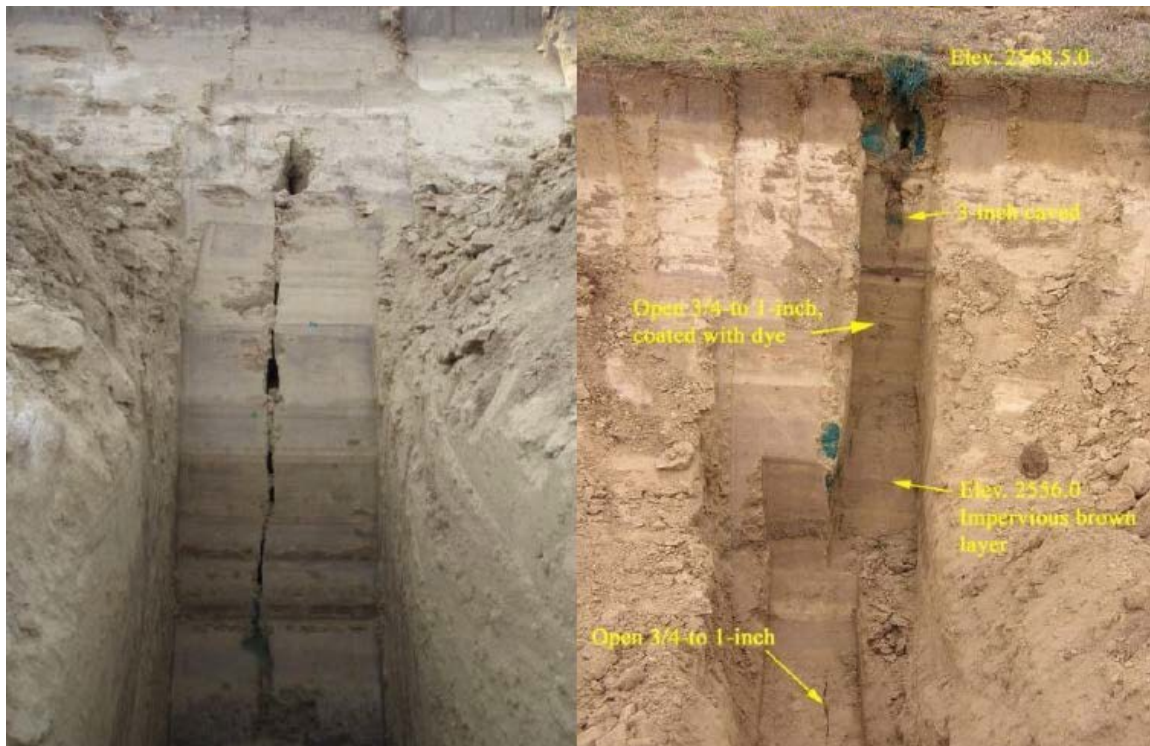
Figure 5.—Representative cracking in the embankment observed in test pit #2. Dye was poured into the sinkholes to aid in tracing the cracks. Cracks were typically 1/4 to 1 in wide.
