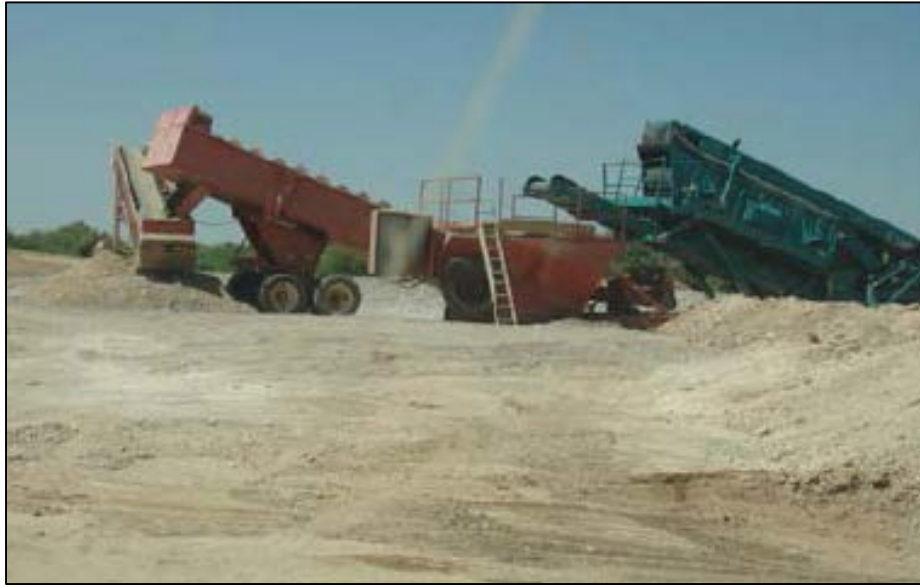
Figure 4.—Screening machine (right) and mixer/elevator (left) for processing filter material, Florence Dam.
