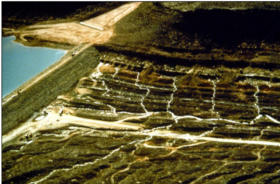
Figure 5.—Excessive leakage during first filling.
