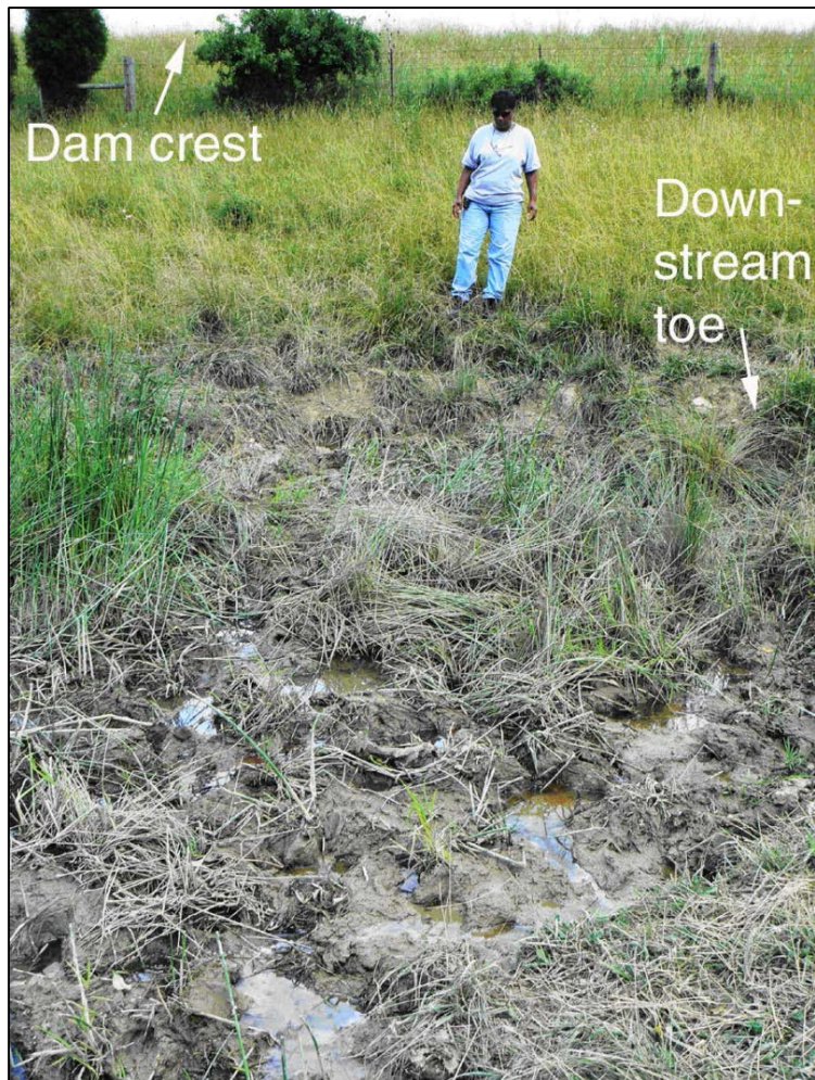
Figure 6-2.—Seepage discharge where the typical grass growth has been retarded in the saturated soil environment and where other vegetation species are becoming dominant.
