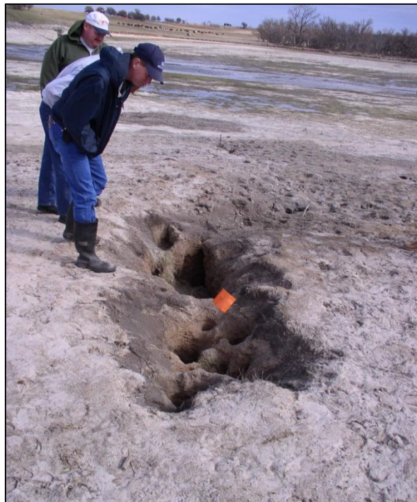
Figure 10-22.—Sinkhole in reservoir area of Little Washita No. 13, Oklahoma. (Photo courtesy of NRCS, Oklahoma)
