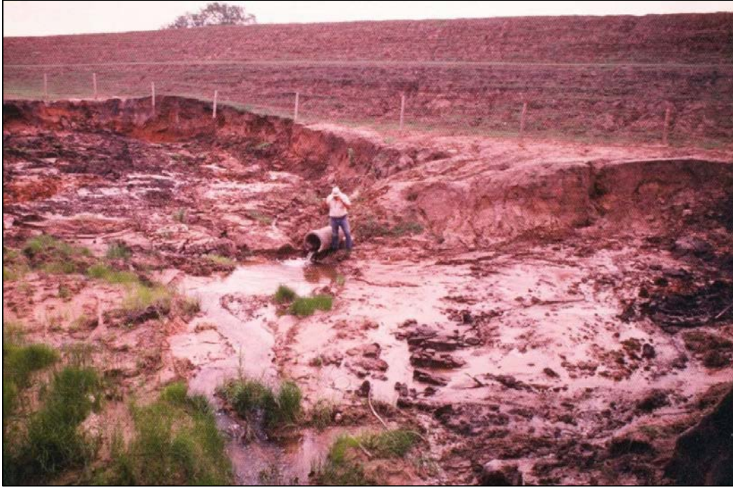
Figure 10-21.—Seepage-caused slope instability near outlet of principal spillway conduit, Little Washita No. 13, Oklahoma (1979). (Photo courtesy of NRCS, Oklahoma)
