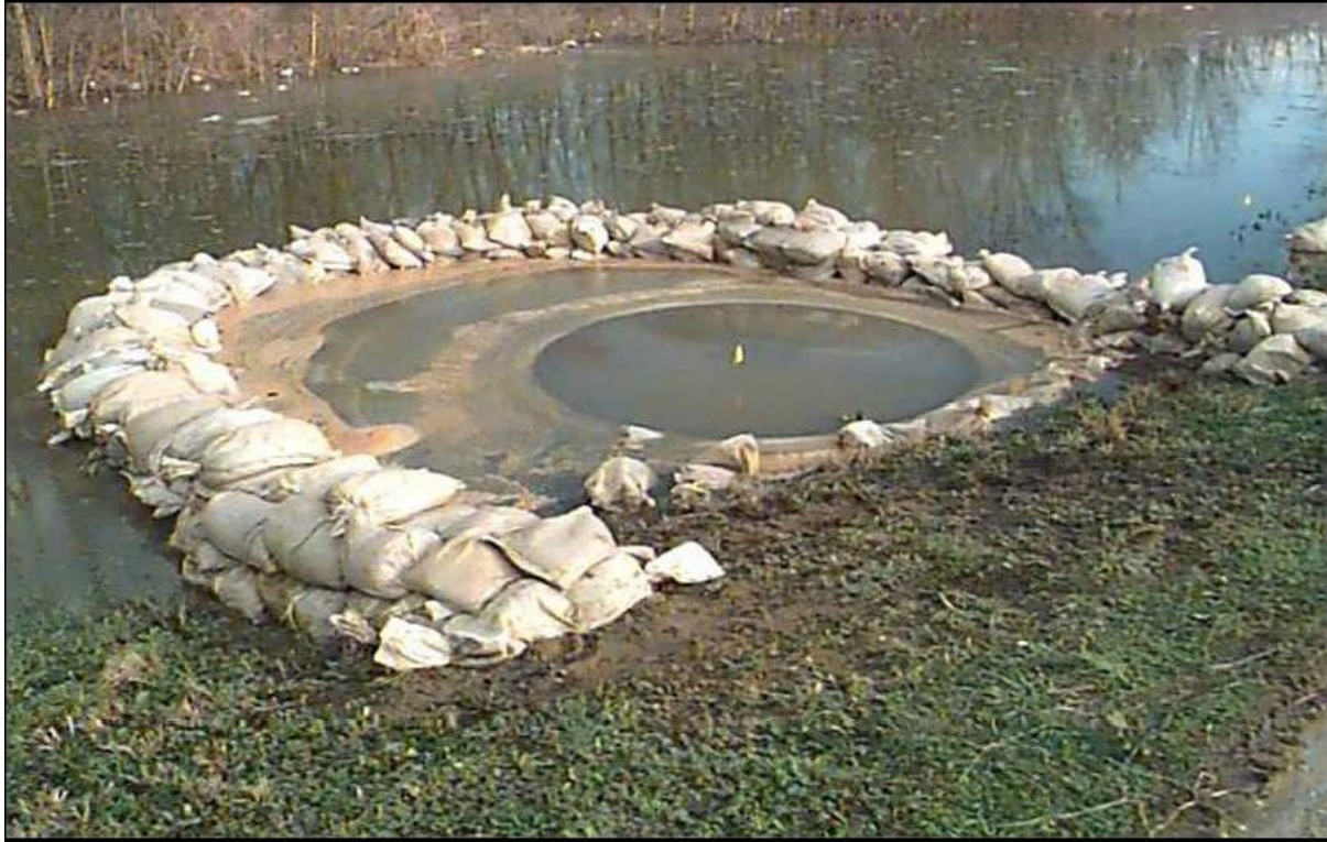
Figure 10-14.—Sandbags placed around a sand boil to increase tailwater level as part of a temporary risk reduction measure. (Photo courtesy of USACE, Missouri Valley Division)
