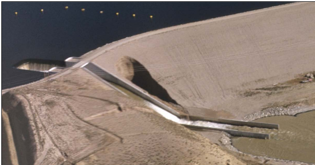
Figure 4-7.—Fontenelle Dam, which nearly breached by sloughing.
