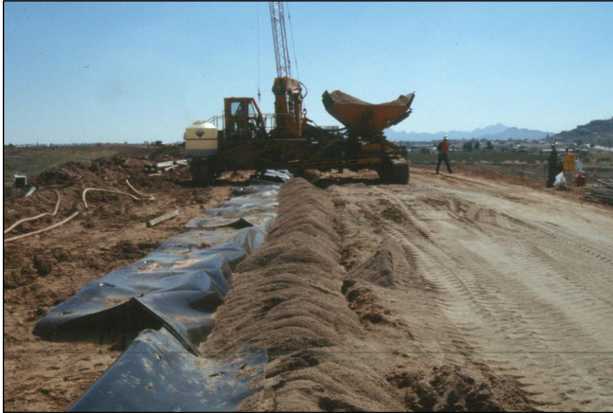
Figure 10-1.—Geomembrane cutoff with sand filter on Reach 11 Dike, Arizona. (Photo courtesy of Reclamation)
