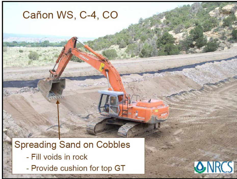
Figure 8.—Placement of geotextile, rockfill, and sand on upstream face (prior to placement of overlying geotextile).
