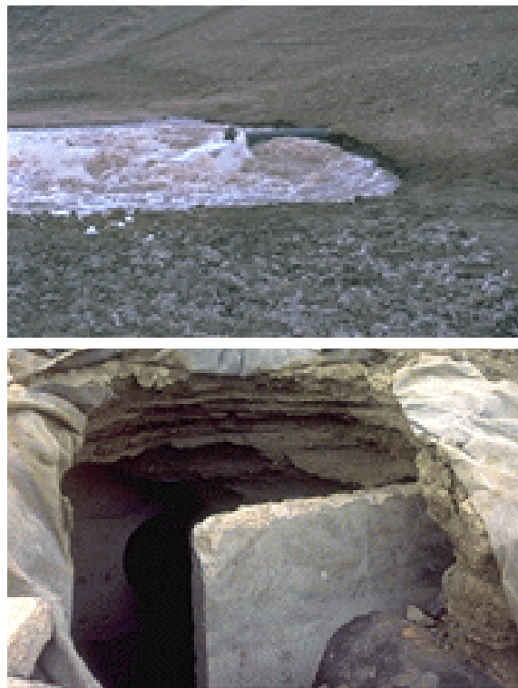
Figure 2.—Discharge of water from internal erosion adjacent to conduit (top photograph) and erosion of fill from around seep collars at upstream end of conduit (bottom photograph) taken after the reservoir emptied.
