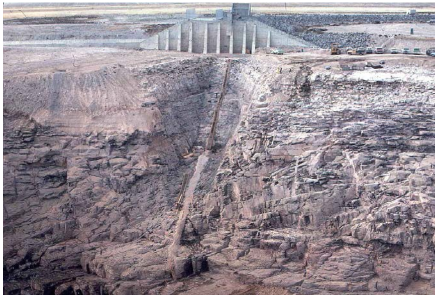
Figure 5.—Deep, highly fracture zone under the right abutment cutoff trench. Joints were generally open, some as much as 2 inches.
