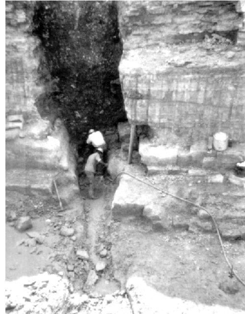
Figure 4.—View of solution feature in cutoff trench of the left abutment.
