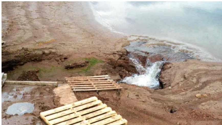
Figure 5.—Observed sinkhole at upstream left groin of Horsetooth Dam.
