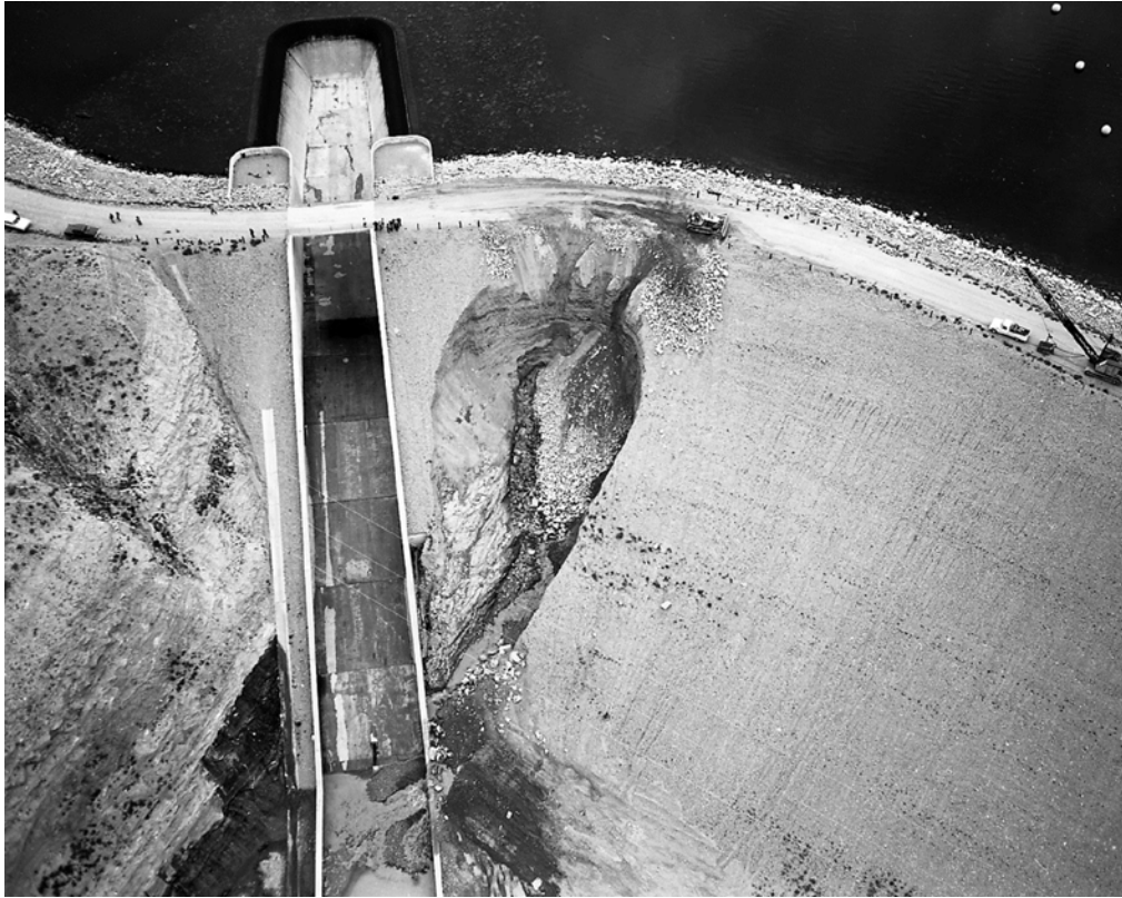
Figure 4b.—The sinkhole migrated in the upstream direction, expanding in size, as material progressively caved from the sides and was washed out of the bottom (stopping).
