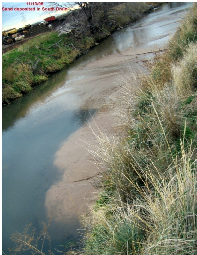
Figure 3.—Eroded sediments in South Drain first noticed by neighboring landowner.
