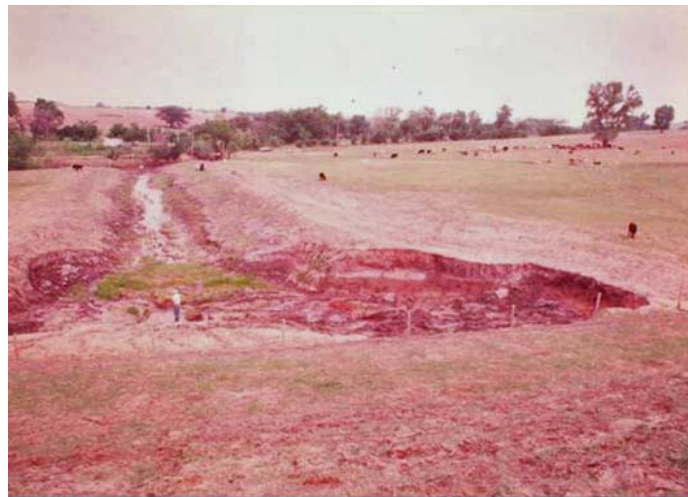
Figure 2.—Sloughing of plunge pool in May 1979.
