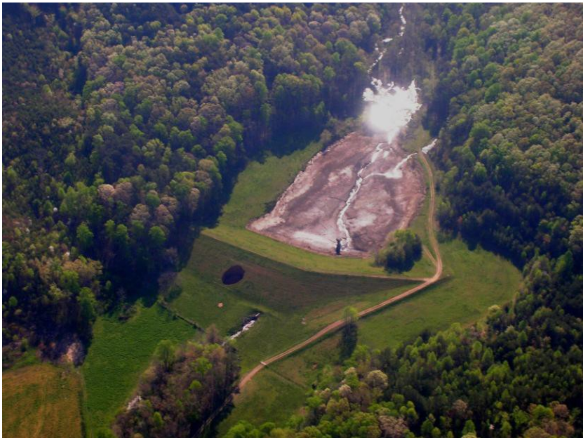
Figure 2.—Aerial view of the sinkhole on the downstream slope of the dam. Photo was taken after the reservoir had been drained.
