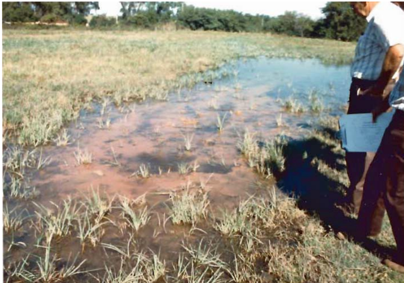
Figure 5.—Seepage occurring downstream from embankment in September 1987.
