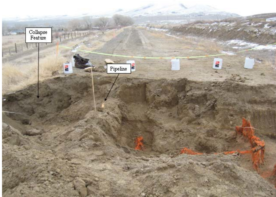
Figure 10.—View of partial excavations of canal embankment crest following grouting with Stratathane™. Features that were found grouted have been painted with orange paint.
