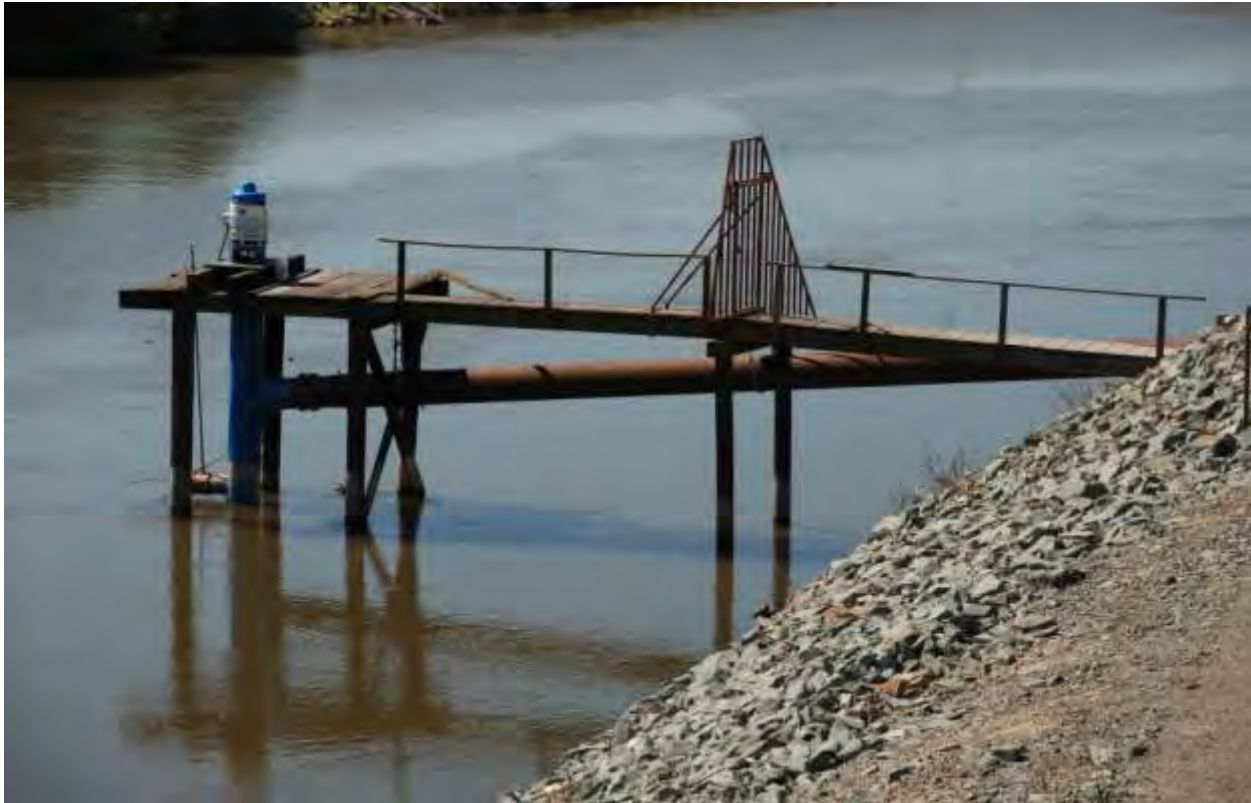
Photo 1. Typical Pump Diversion
