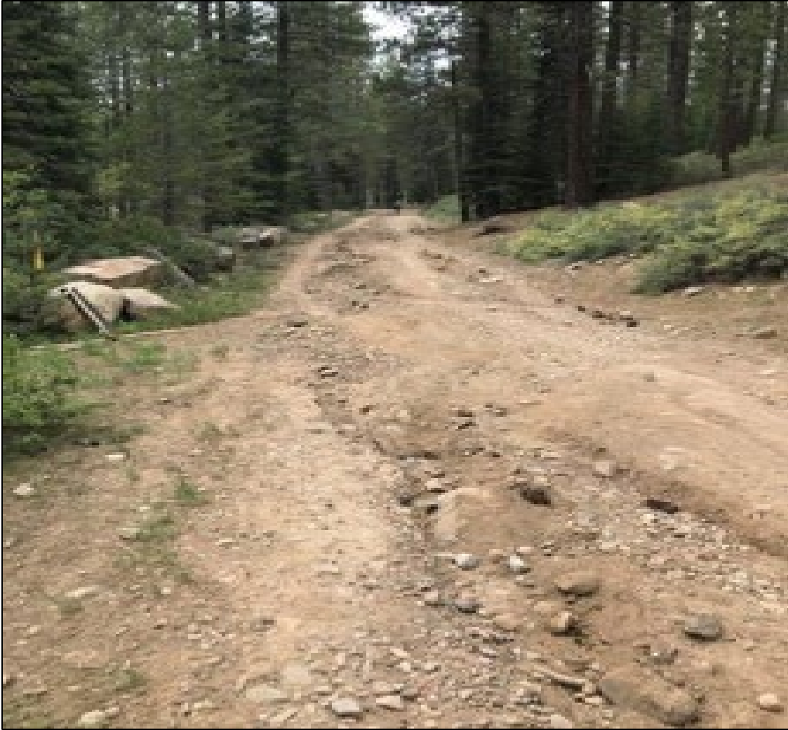
Figure 5.1 - Pre-project: Roadway without drainage features exhibiting significant erosion
