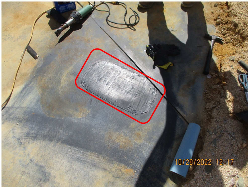
Photo 11 – October 28, 2022, Temporary patch completed covering the three holes discovered in the Pond 1 liner.
