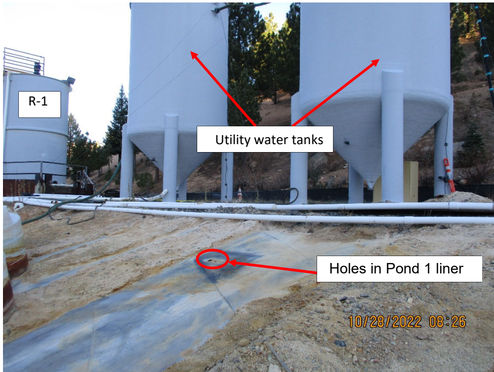
Photo 10 – October 28, 2022, Holes discovered in Pond 1 liner.
