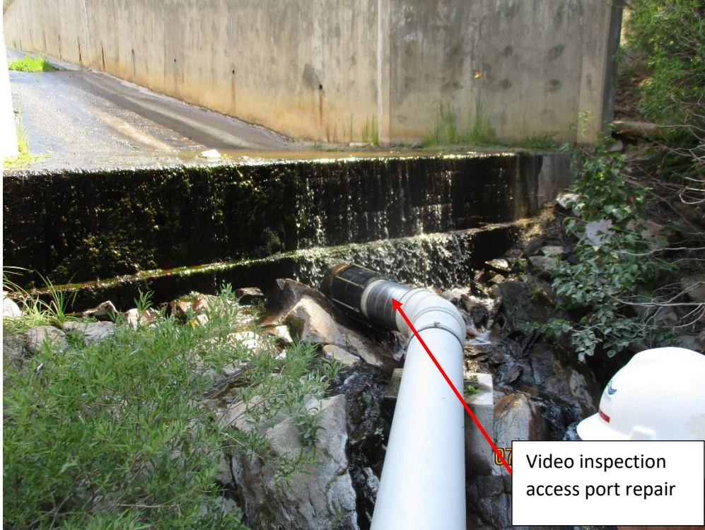
Photo 5 – July 13, 2022, Repair of video inspection access port. Port was covered with a rubber sheet gasket and stainless-steel sheet. The rubber and stainless-steel sheets were secured with four heavy-duty stainless-steel band clamps.
