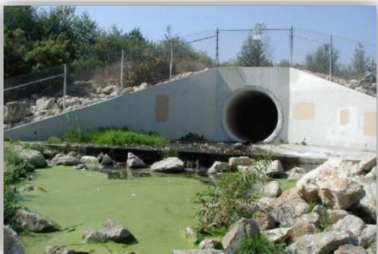
Photo by: Christina Arias, San Diego Regional Water Board staff.
