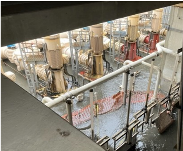
Photo of flooded influent bar racks and influent pumps 8-20-21 (IBWC)
