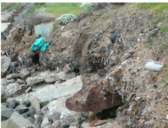
Photo 1. Landfill shoreline before repair work.
