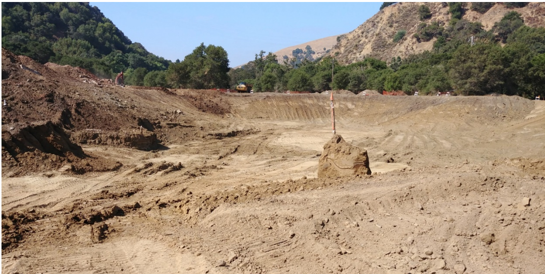
Figure 2: Part of the overburden excavation on August 16, 2018. View looking west. A large haul truck is in the background on the edge of the excavation.
