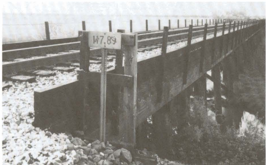
A raised section of the Union Pacific Railroad line northeast of McCormack-Williamson Tract.
