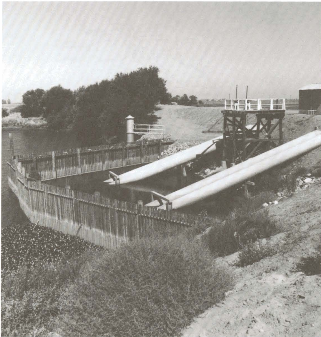
Siphon at Tom Paine Slough, installed as part of a settlement contract to improve water quality in a portion of the South Delta Water Agency.
