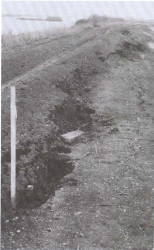
Cracks occurring on the levees of a low-lying island.
