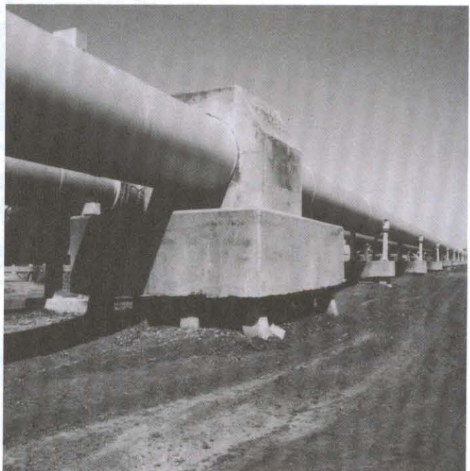
Land subsidence on Orwood Tract is exposing piles supporting the East Bay Municipal Utility District Aqueduct. These piles extend deep into the ground to assure continued stability.
