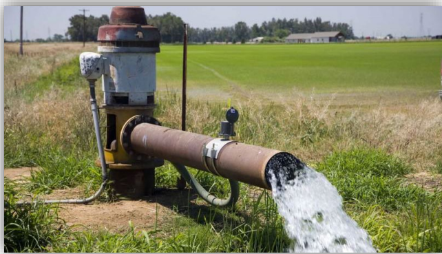
Photo: Water diversion metered using a strap-on meter.
