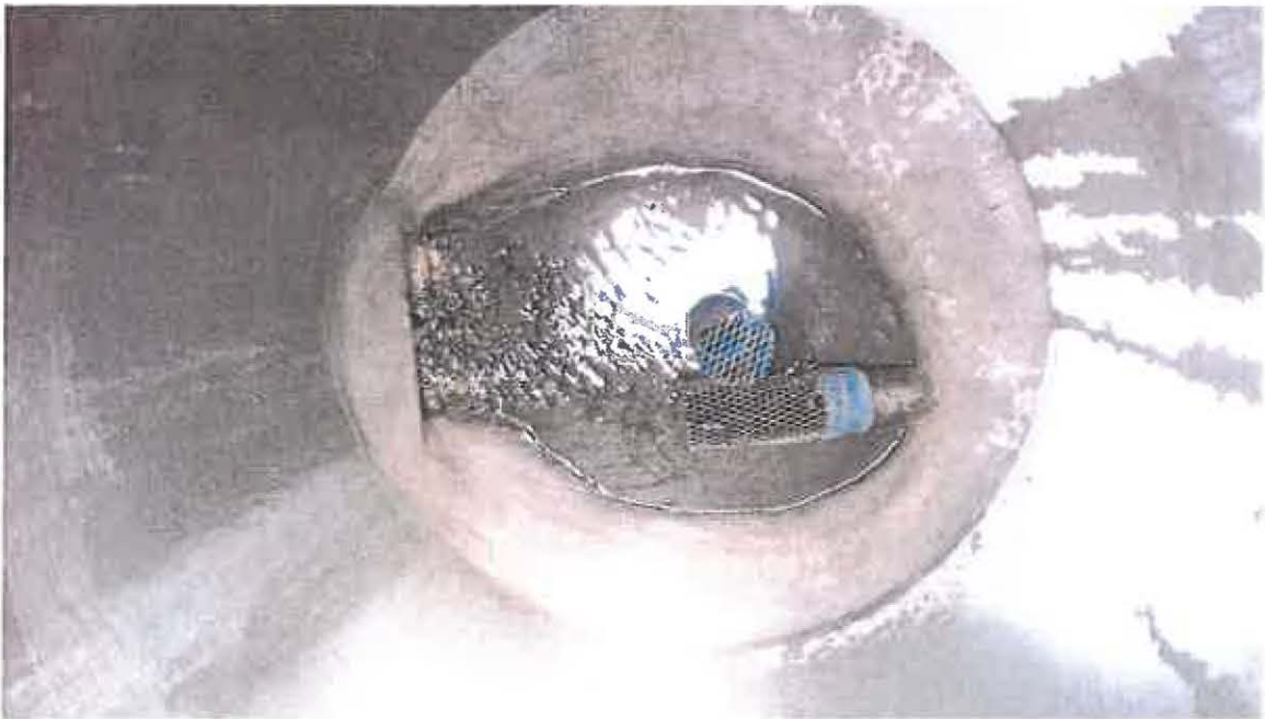
Inside spring well. Perforated horizontal pipe collects sub-surface water and enters the well from the left side. Vertical pipe at center bypasses flow when water level exceeds 4-6 inches. Horizontal pipe at right diverts water to collection system.
