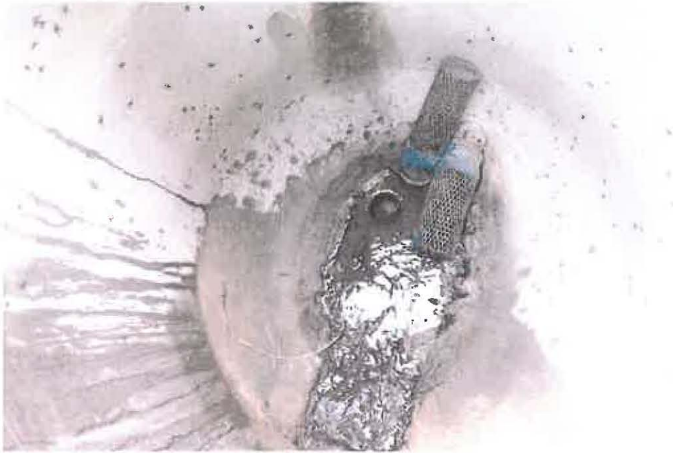
Vertical bypass pipe with cap removed so that all water is bypassed, due to cricket infestation.
