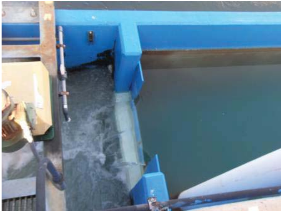
Photo 4: View of final effluent flowing over rectangular weir at the terminus of the chlorine contact basin.
