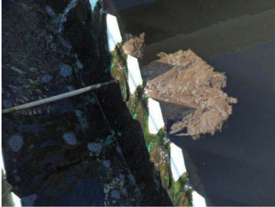
Photo 3: Close-up of algae build-up and solids accumulation shown in Photo 2. Solids accumulation appeared to cause uneven flow distribution over the weirs.
