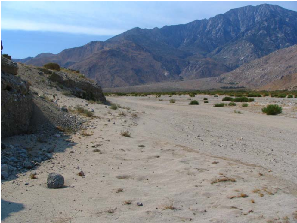
Area 2- looking south at washout (slumping has buried pipeline in left of photo).
