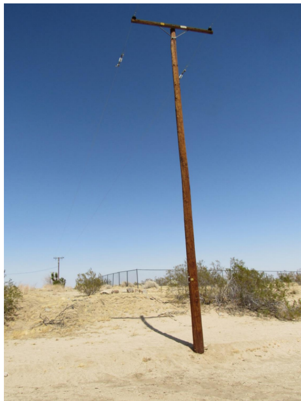
Photo 2. Pole 34112S, Facing North
