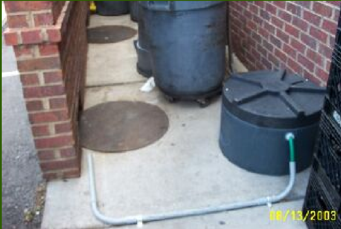
Interceptor 1 st chamber under aeration
