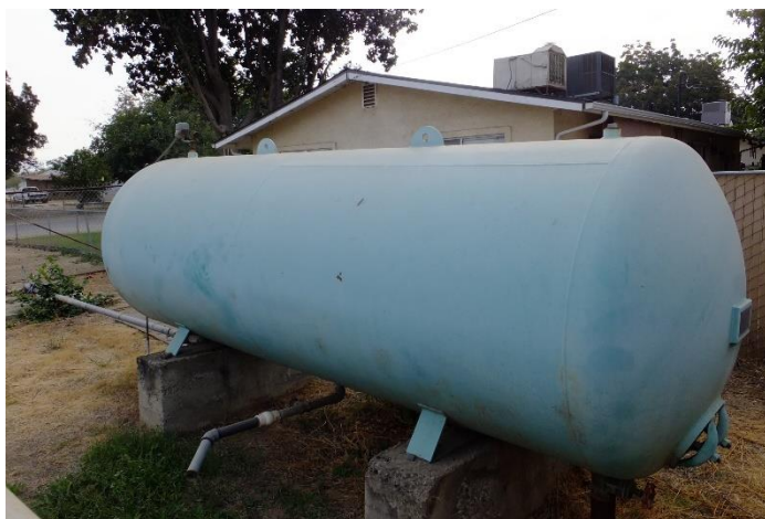
Figure 1: Beverly Grand Hydro Tank
