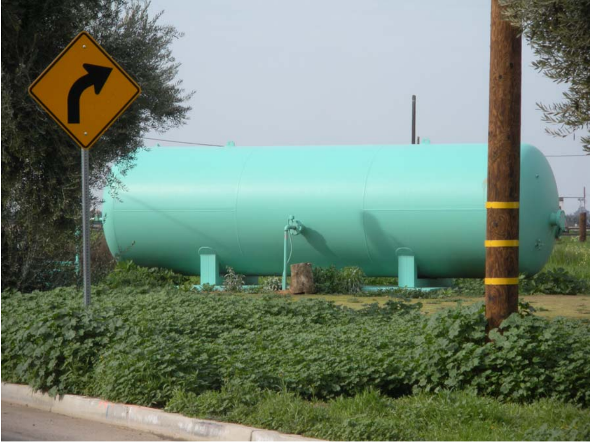
Installed hydro-pneumatic tank
