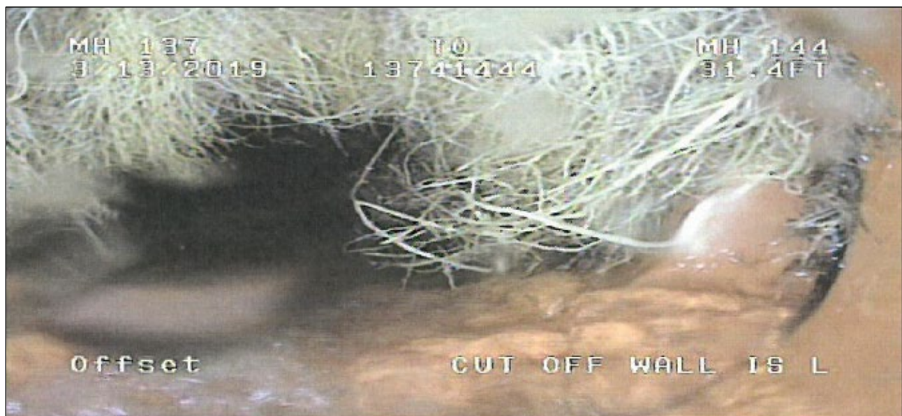
Figure 9.1. Broken Collection System Pipe found during 2019 CCTV Inspection showing roots penetrating the sewer (top) and a pipe offset (bottom).
