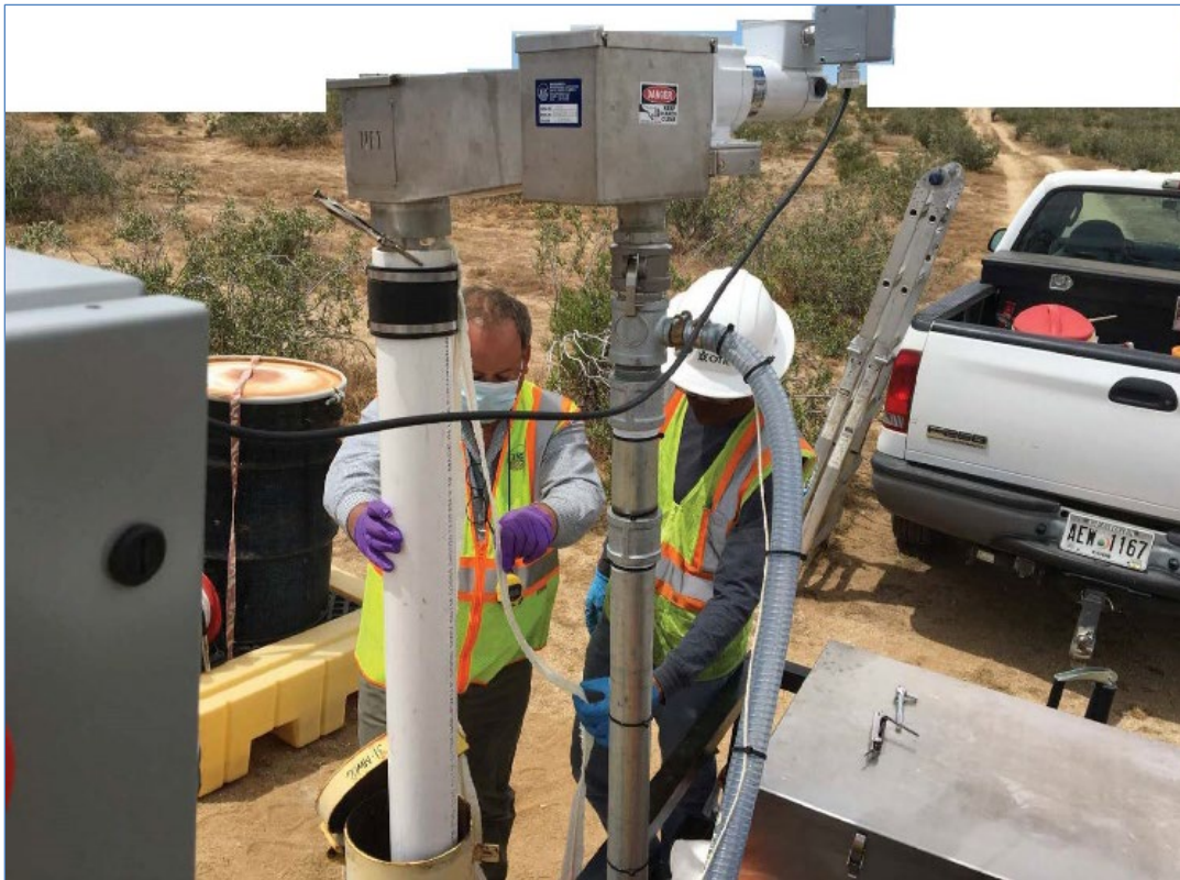
Photo 11.2 showing field technicians gauging LNAPL and water level while the NET system removes product from the well. Note the system is mounted on a small utility trailer and can be moved around the site.
