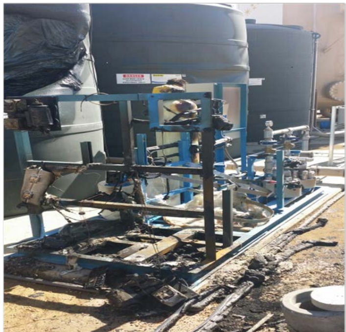
Photograph 2 - Two damaged backwash tanks on the left side. In lower foreground is the destroyed drinking water filtration system. At the right center is an undamaged treated water storage tank (black color). At the far right in a tan color is one of the
