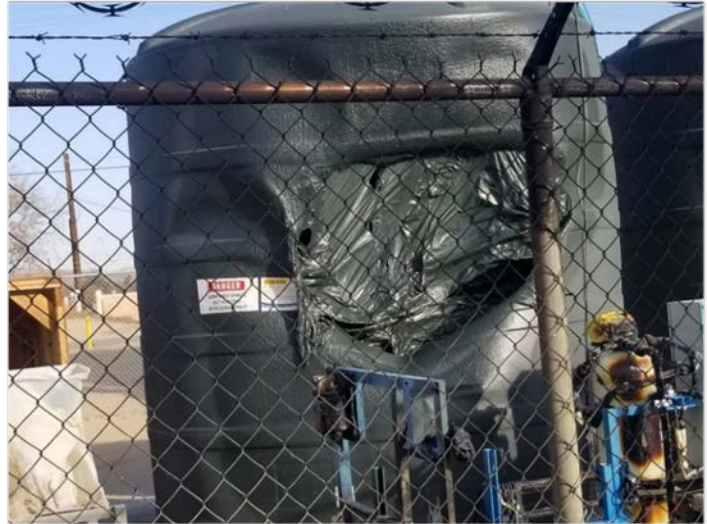
Photograph 1 - Damaged backwash tank (photo from a resident from Soapmine Road)
