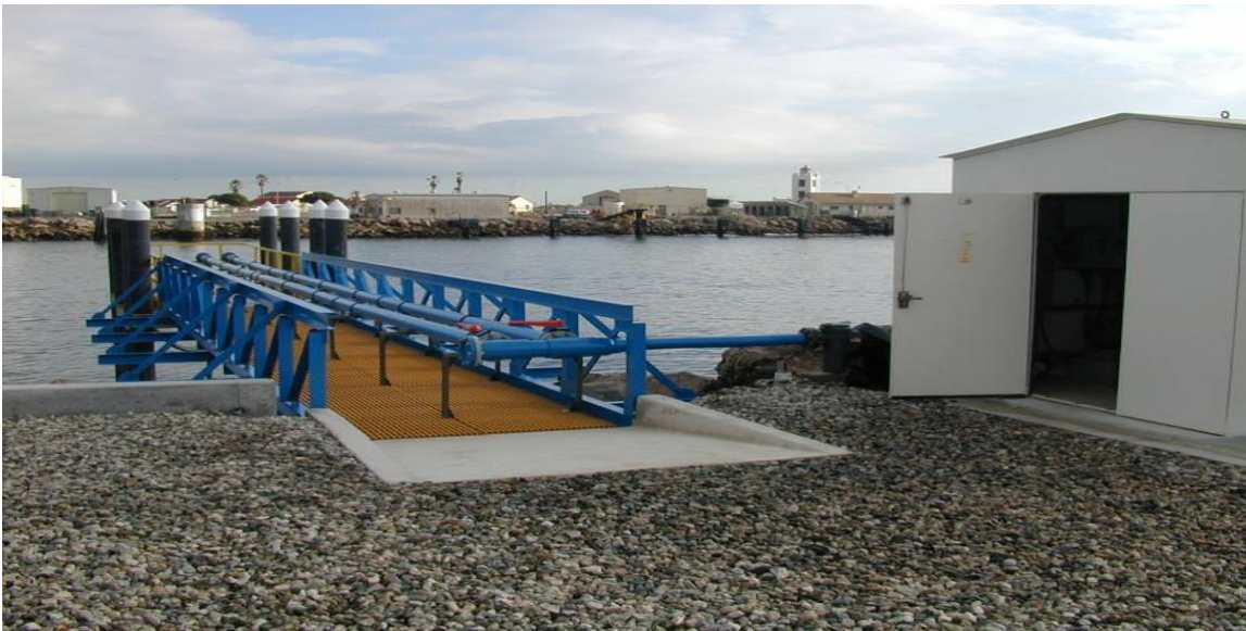
Figure 3: Sewer Intake to Pump House
