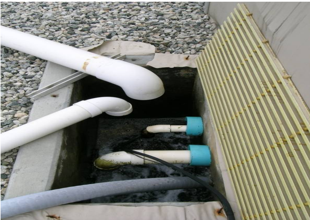
Figure 4: Seawater sump where seawater, permeate, and brine streams are combined before discharging to Port Hueneme Harbor
