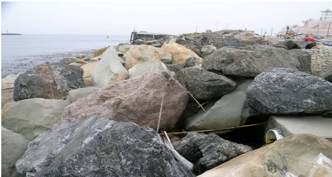
Figure5: SDTF facility outfall consisting of 12-inch conduit positioned on rock rip rap at a distance of thirteen feet from receiving water.
