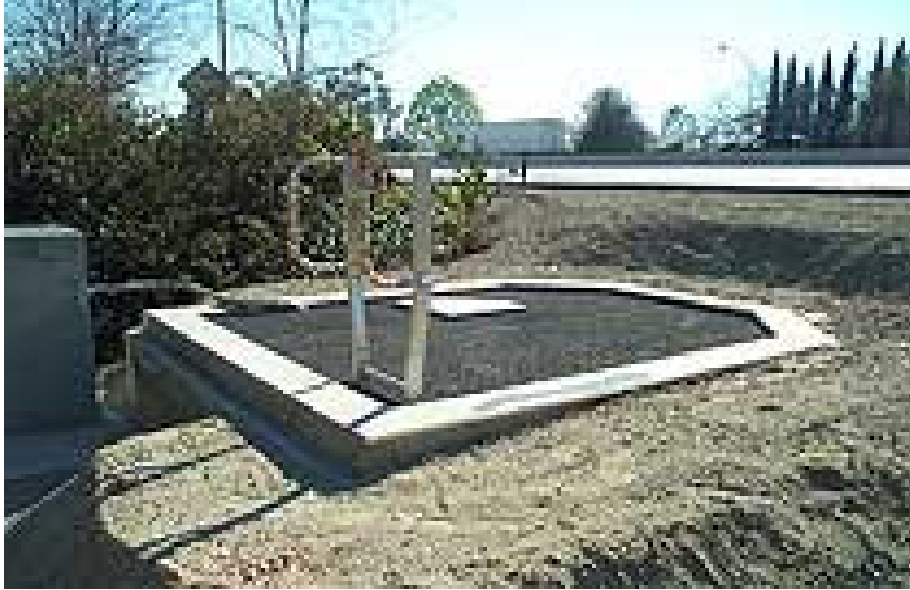
Figure 6.3-4. Location with GSRD Installation.
