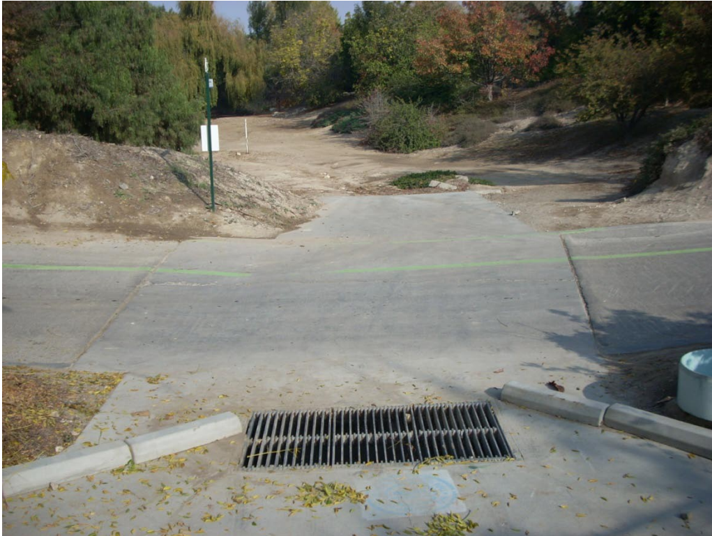
Figure 2.12 Lariat Monitoring Site at Drainage Structure Collecting Flow from Agua Magna/Sepulveda/Blackwater Canyons
