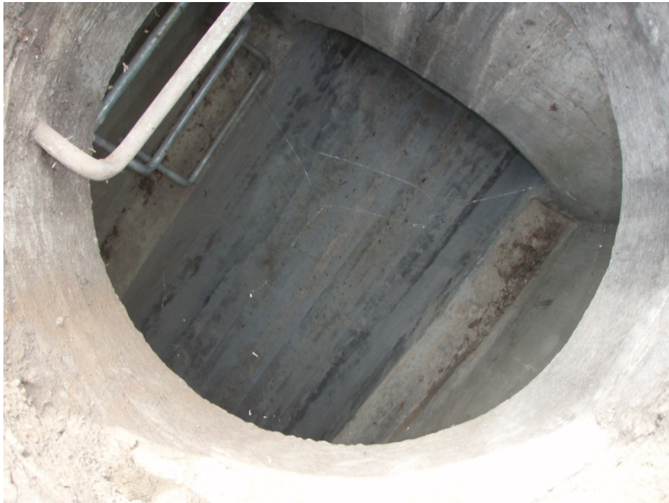
Figure A-2: Site 10_EAST viewed from above the manhole. Taken on January 11, 2011 at 12:30 p.m.
