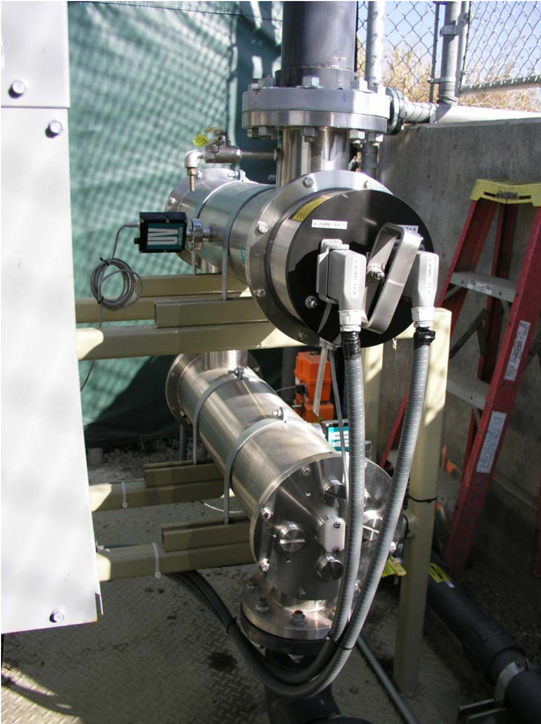
Figure 5. UV Cylinders. Each of the stainless steel cylinders contain four (4) – ultra violet light lamps enclosed in protective quartz sleeves.
