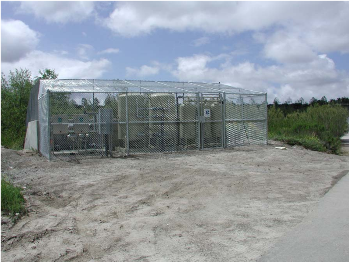
Figure 1. Completed Clear Creek Systems, Inc. (CCS) Package Treatment Plant Installation.
