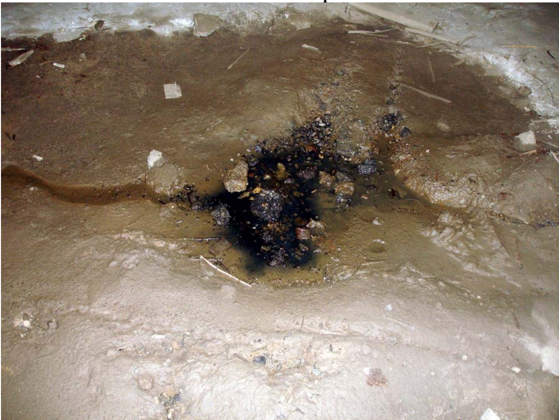
Photo 6: Basin leak puddle
