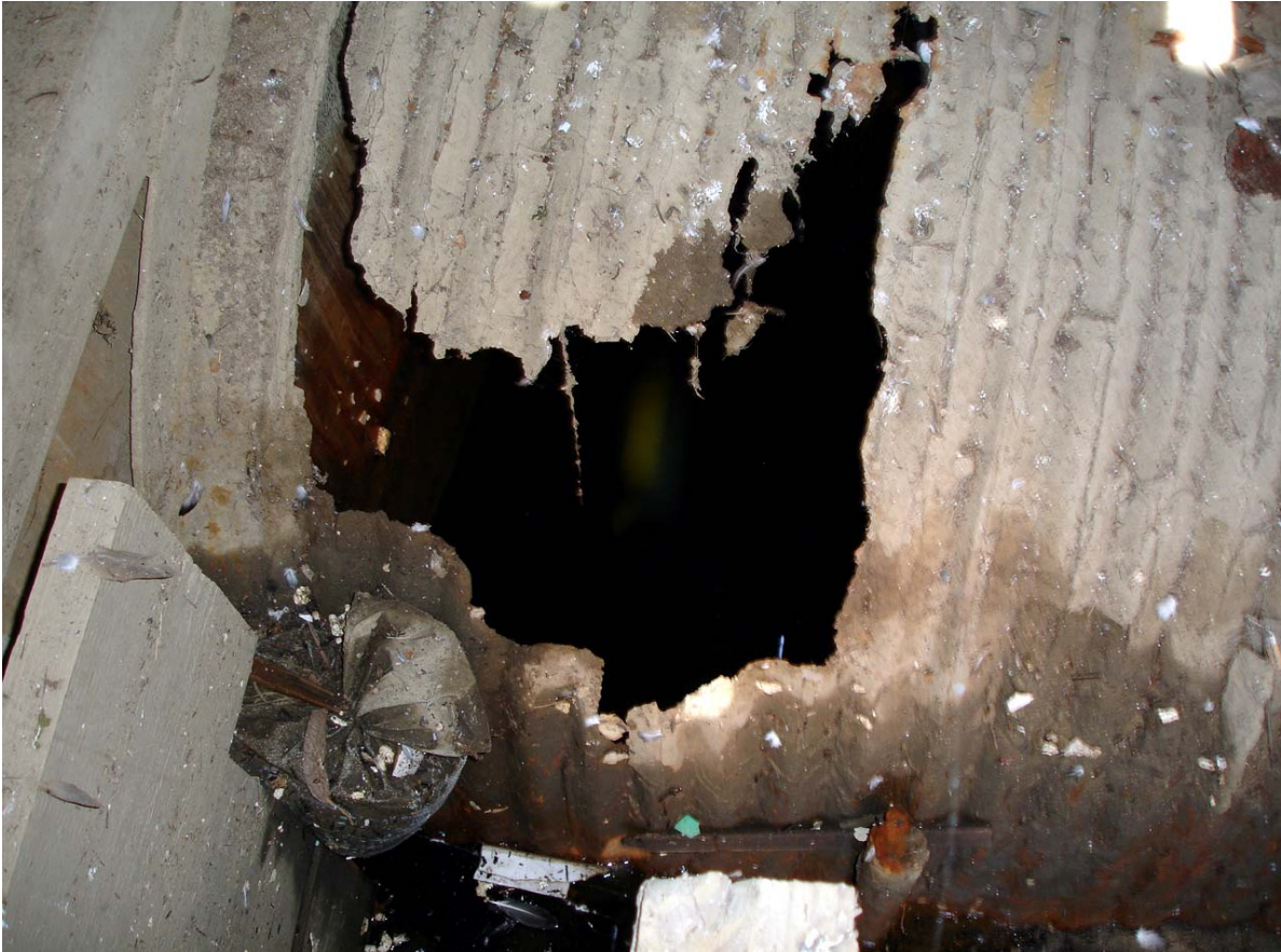
Photo 2: Broken Storm Drain (from above)
