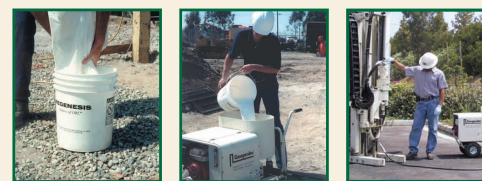
ORC powder is mixed with water to form a slurry. ORC slurry is poured into the hopper of a slurry injection pump. Direct-push injection of slurry.
