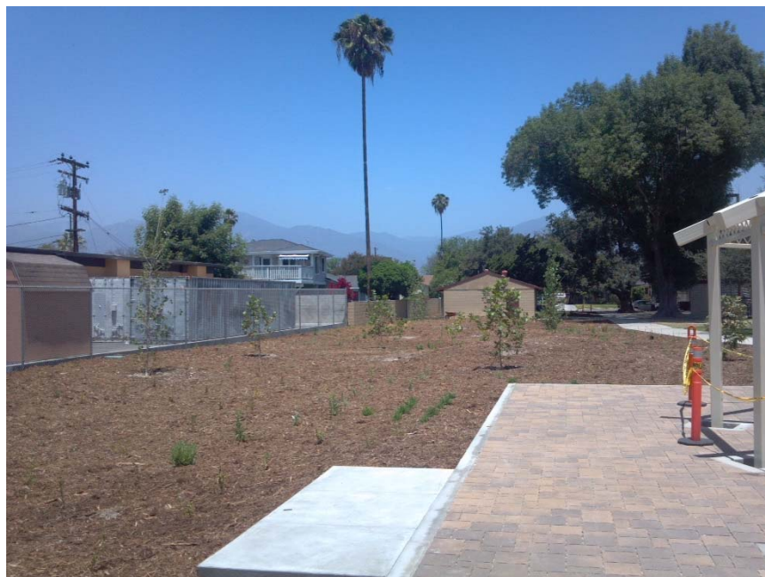
Mulched infiltration swale at Lambert Park
