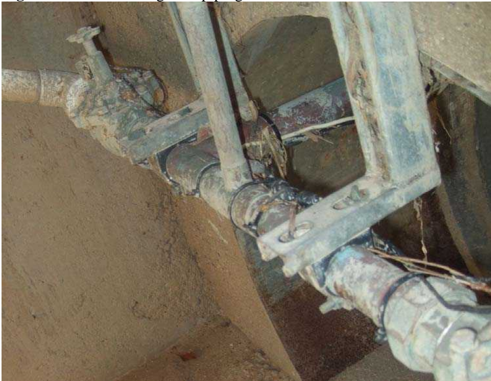
Figure 2-4. Private irrigation piping in storm drain
