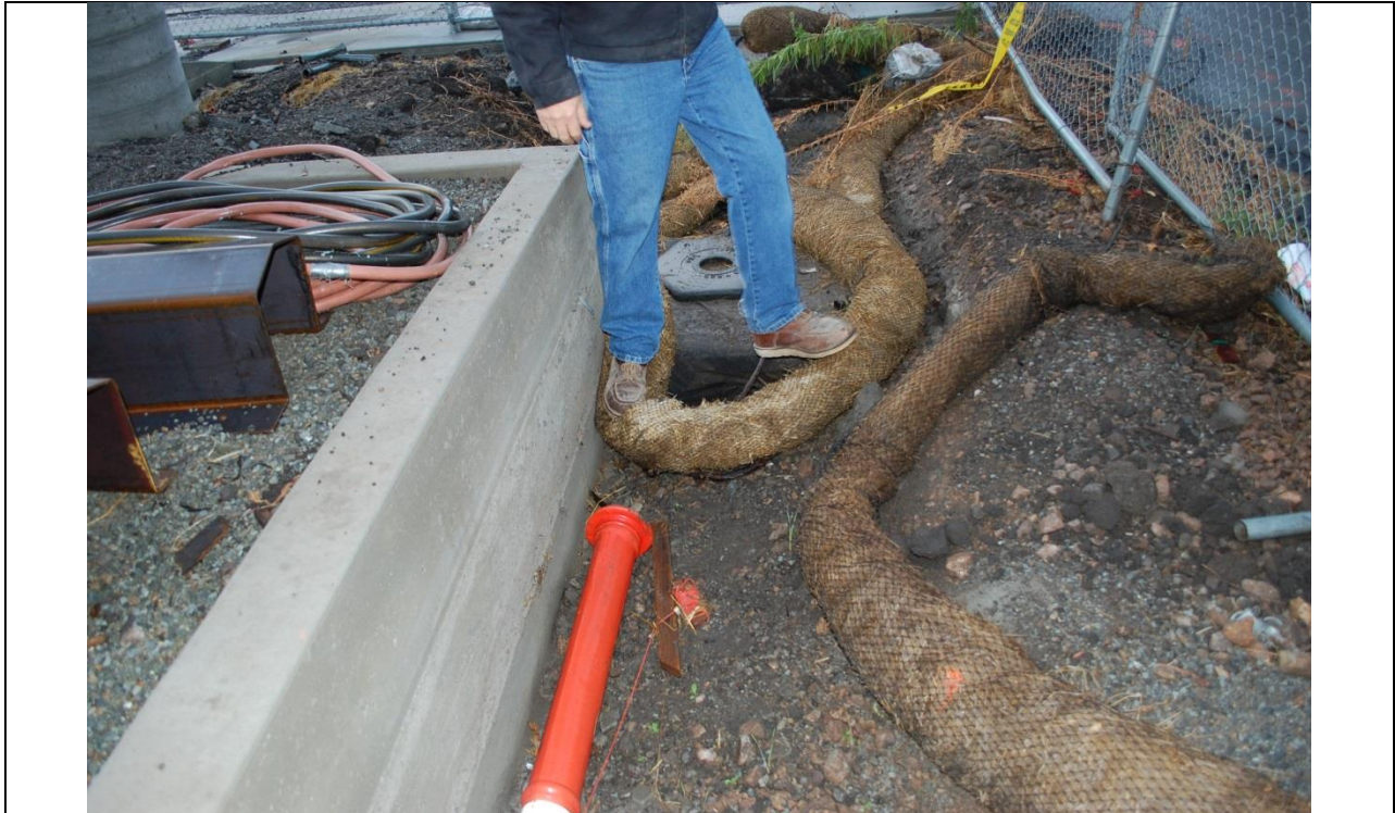
Photo 8: Drop inlet at the southwestern corner of the site. The fiber roll under foot was just placed there by the contractor, but was not in place during the rain event.
