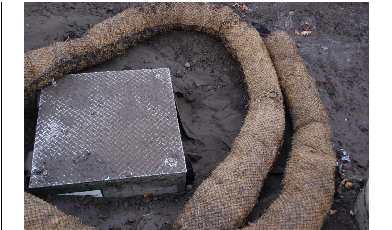
Photo 2: Close-up of drop inlet shown in Photo No. 1
