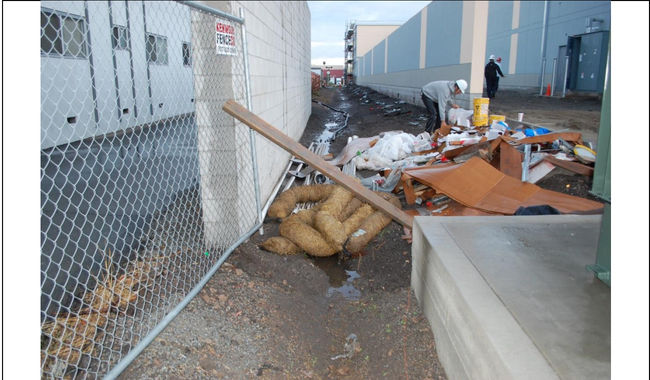
Photo 7: Debris and trash uncontained in a drainage swale with insufficient erosion and sediment controls.
