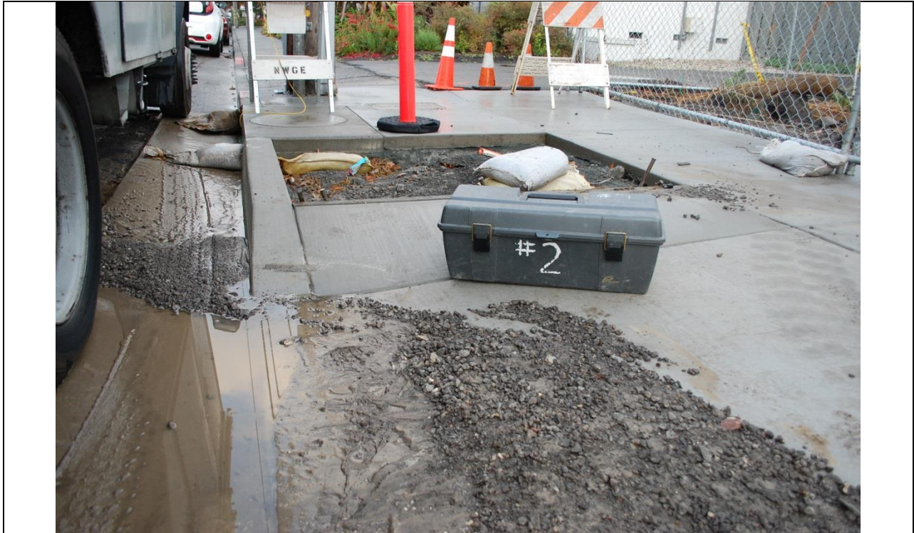
Photo 10: Residual water in the gutter with pH of 10.02.
