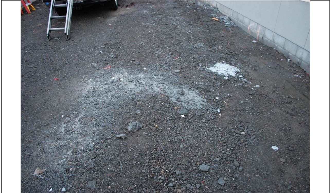
Photo 9: Insufficient containment of residual stucco waste, which was exposed to rain.
