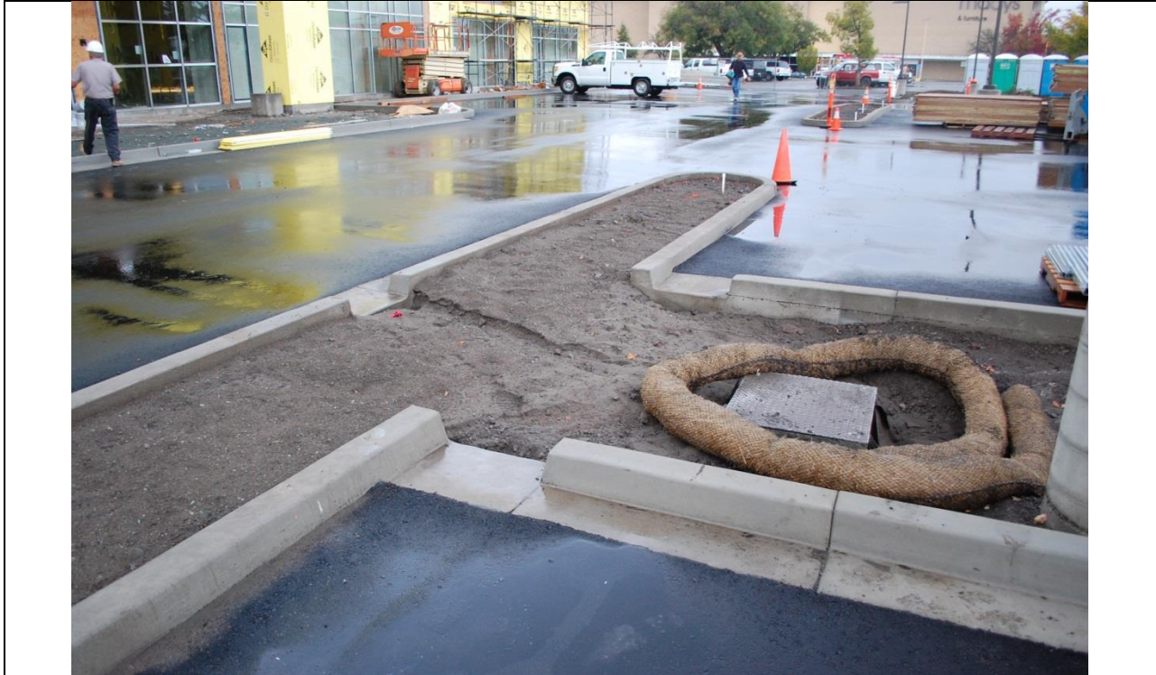
Photo 1: Onsite drop inlet with evidence of erosion and sediment transport. Fiber roll is not installed per specification (not trenched in or staked and is being used in an area of concentrated flow).
