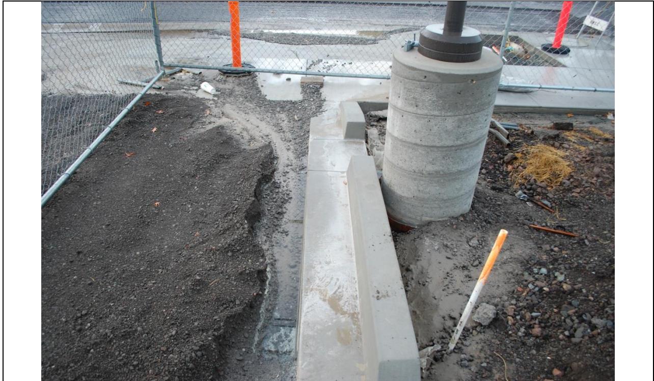
Photo 6: Evidence of erosion and sediment transport with insufficient controls and apparent concrete washout/disposal.
