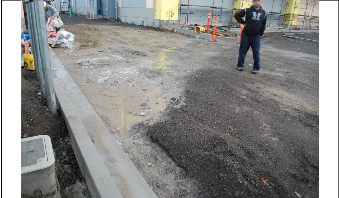
Photo 5: Evidence of erosion and sediment transport with insufficient controls and apparent concrete washout/disposal.
