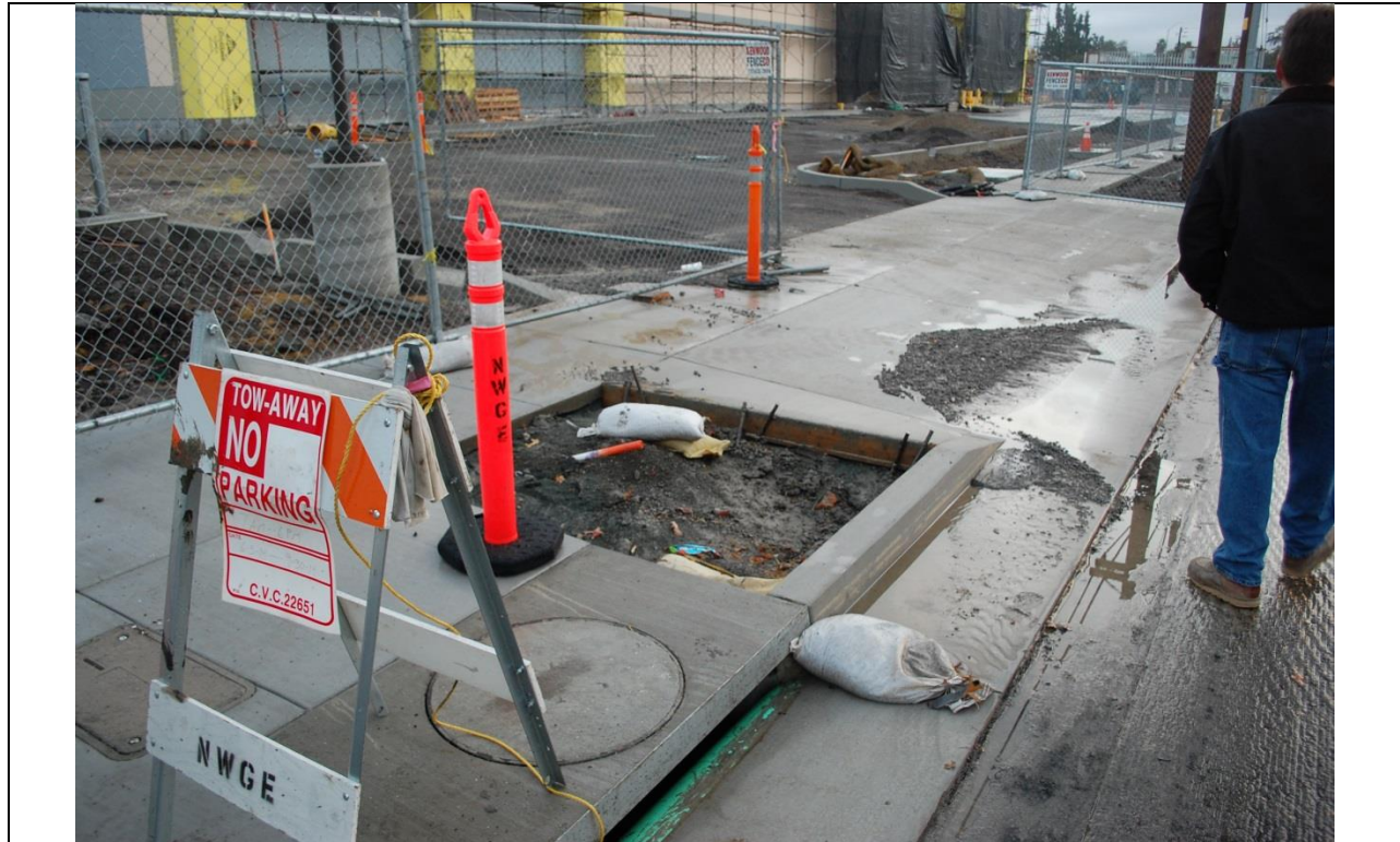
Photo 3: Sediment and high pH water in the gutter.
