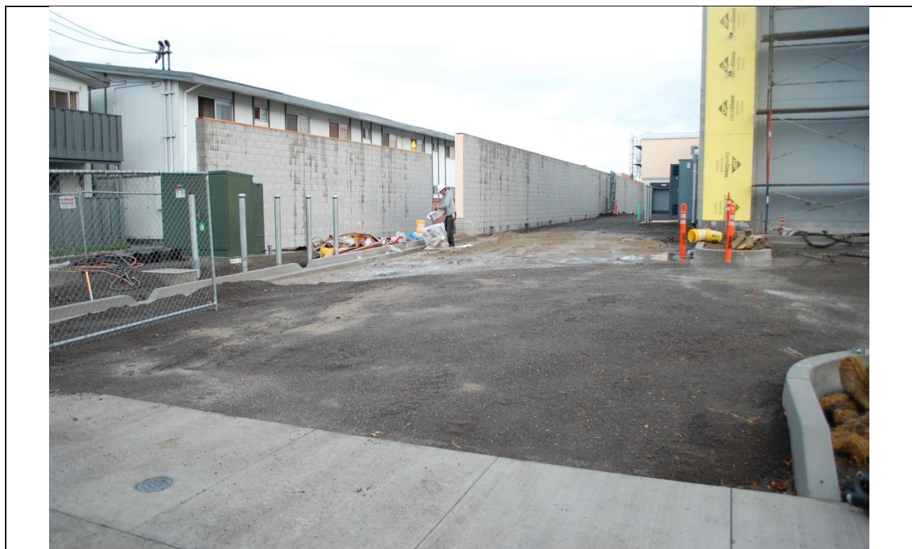
Photo 4: Southwest corner of the Site with insufficient erosion and sediment controls.
