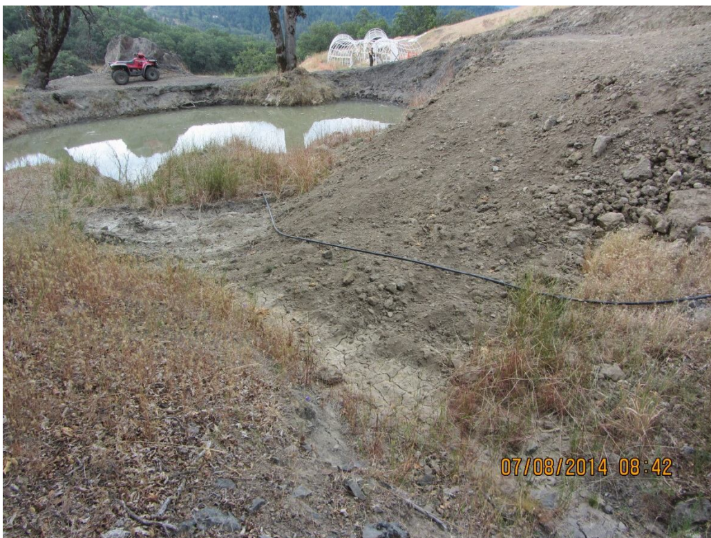
Image 12 – shows perched earthen fill materials adjacent to and deposited in the streams entering the pond. (Photo 6951)
