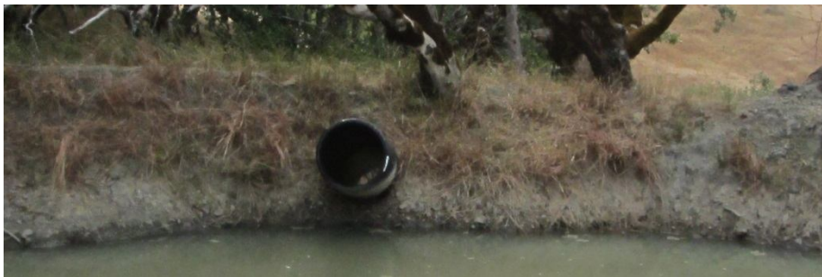
Image 10 – shows the pond, spillway, culvert, and dam. Note the trees are buried in the fill. (Photo 6963 cropped and zoomed in)
