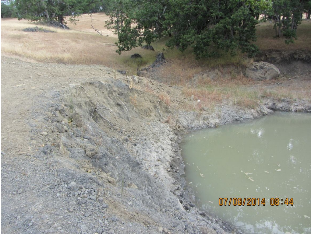
Image 11- shows perched earthen fill materials above the pond, (Photo 6960)
