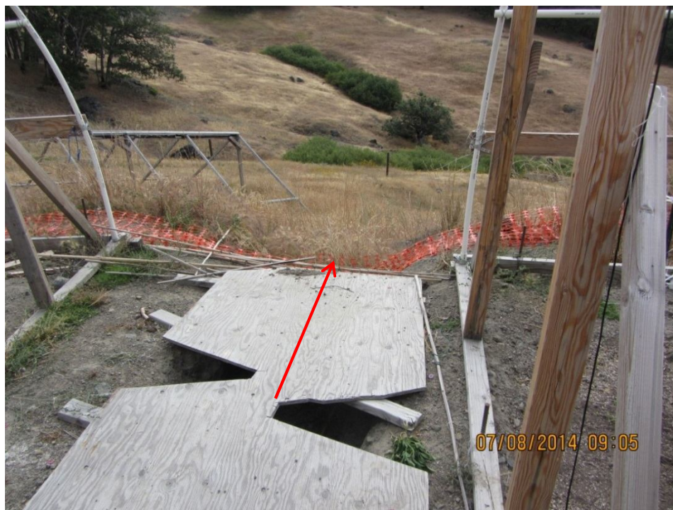
Image 18 – Here the drainage ditch outlets onto the slope below.
