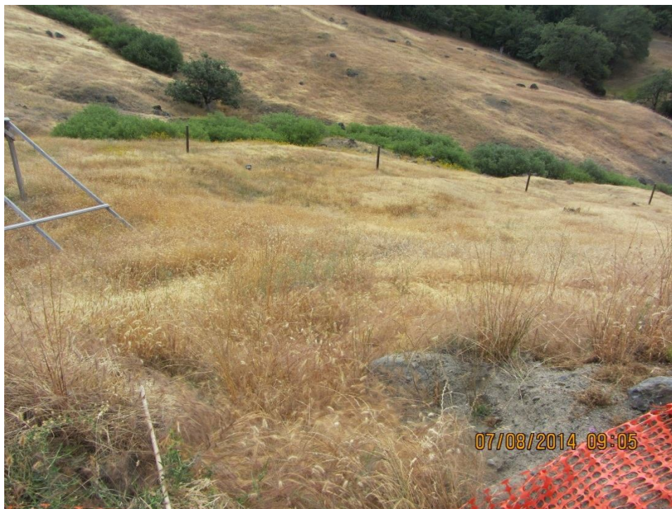
Image 20 – is looking downslope from the four greenhouses to the Class II streams, approximately 200 feet below. Note the hummocky topography, potentially indicating unstable ground. Drainage features and conveyances on the pad for the greenhouse area concentrate runoff from this area onto the slope below. (Photo 6991)
