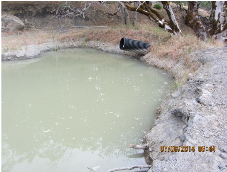
Image 13 – shows the pond spillway culvert. Note the pipe is installed at a steep angle. This is not an orthodox installation, and appears to threaten the dam with overtopping and eroding during heavy rainfall. (Photo 6959)
