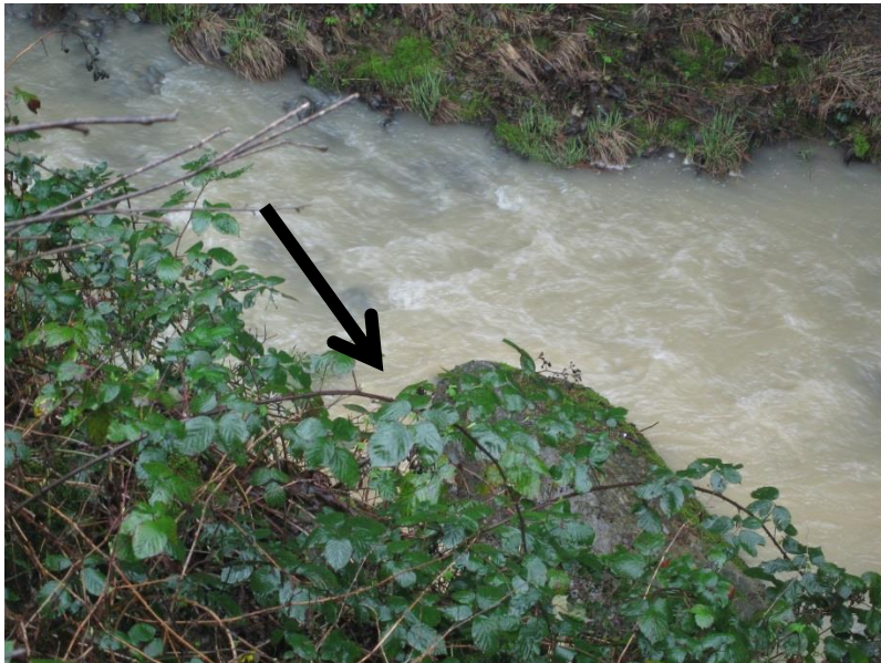
February 19, 2016 – Photo 1D. Point of culvert outfall into Mark West Creek. Paul Keiran, Regional Water Board staff photograph
