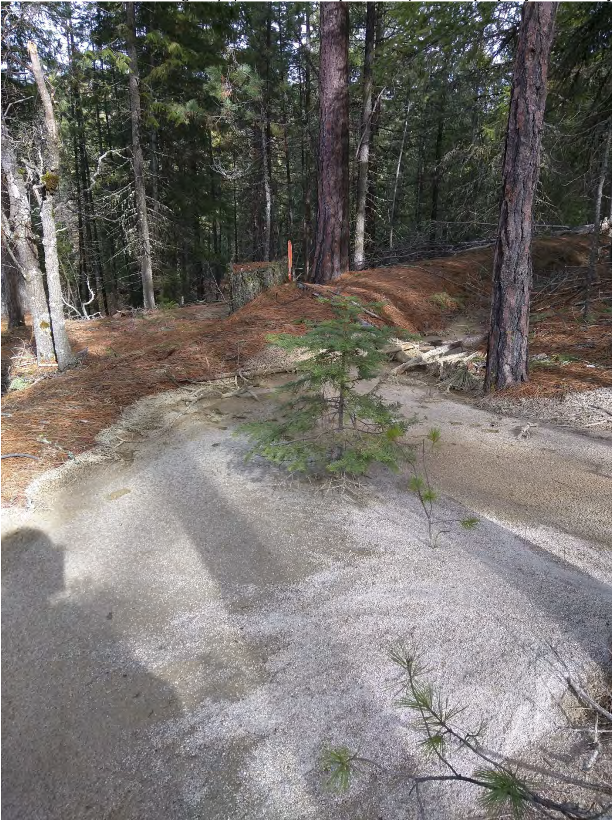
Photo 43: Deposition in the existing ditch line from the well installation area
