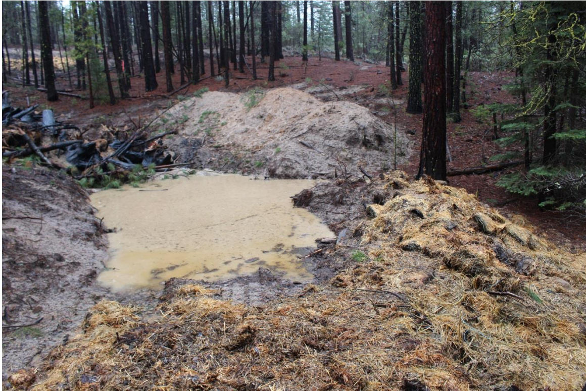
P11 1/29/2016 10:38 AM Looking south at turbid water in catch basin, and burn pile.
