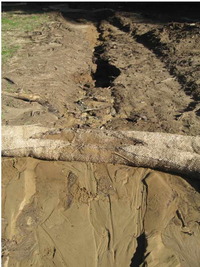
Photograph 2. Mary Court Subdivision – 11/02/16: Discharge of sediments from the Site into a small ravine. Photograph by Paul Keiran, Regional Water Board staff
