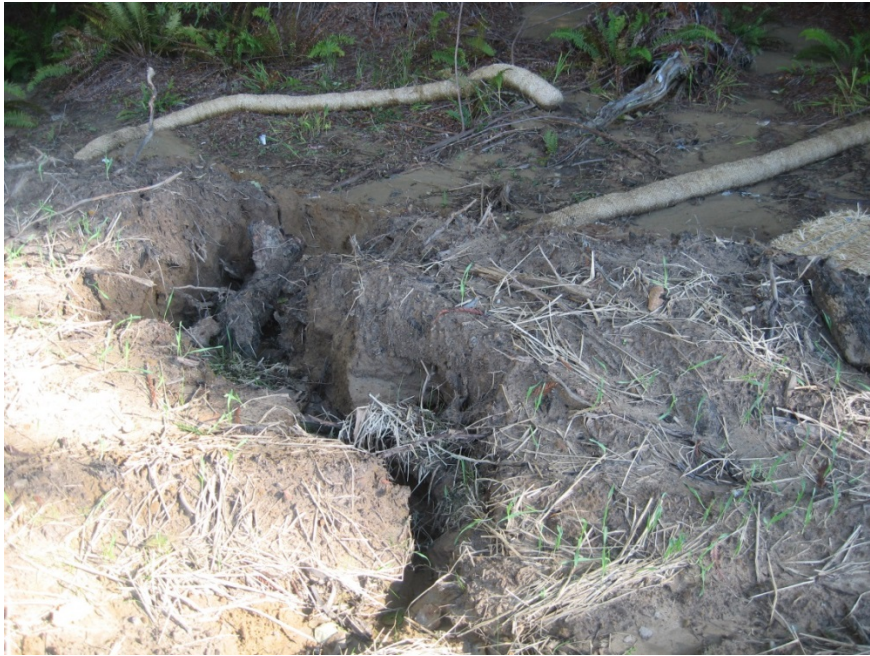
Photograph 3. Mary Court Subdivision – 11/02/16: Large gullies formed by high velocity flowrate. Photograph by Paul Keiran, Regional Water Board staff
