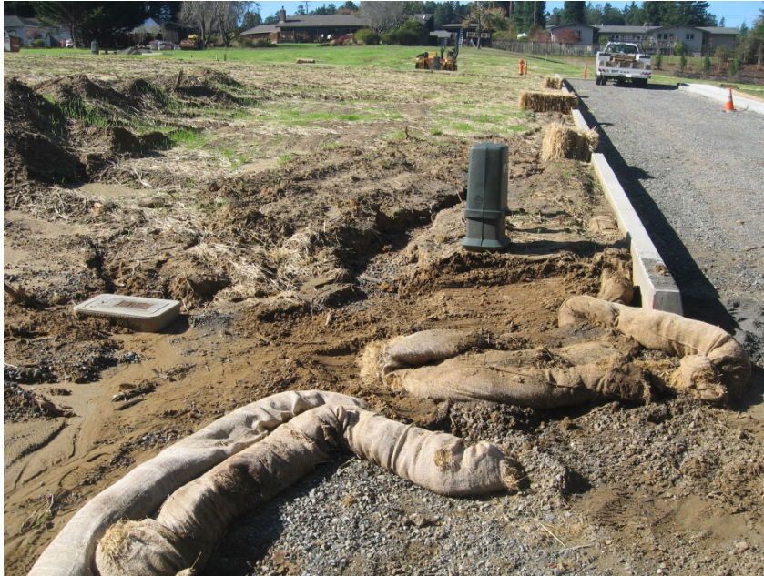
Photograph 1. Mary Court Subdivision – 11/02/16: Curb and gutter alignment that concentrated storm water runoff. Photograph by Paul Keiran, Regional Water Board staff
