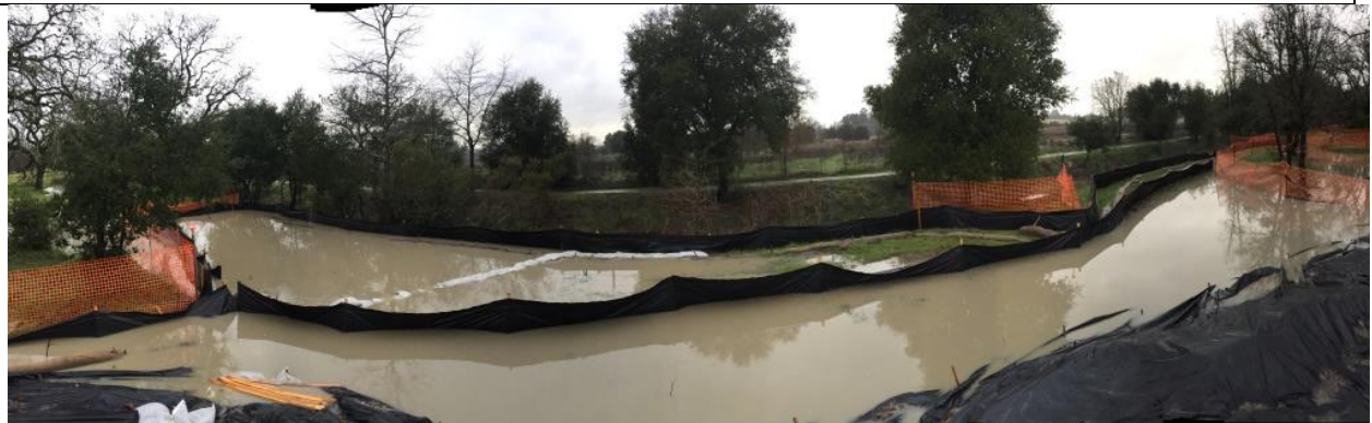
Photo 14: A view of improvised detention basins along western Project boundary, looking west.
