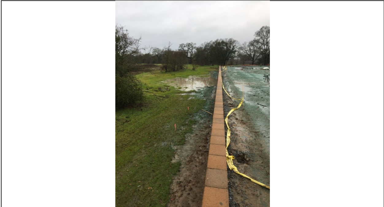
Photo 13: Retaining wall along southern Project boundary, looking west. The puddle consists of muddy runoff from the Project site and may be a jurisdictional wetland as identified in Project 401 certification application documents. Runoff from disturbed Project areas reached this depression area by passing below the western end of the wall, whereupon it flowed east into this area.
