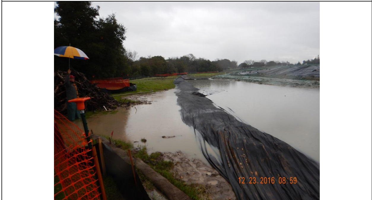
Photo 6: Earthen berm covered with filter fabric. Looking north. Peterson Creek is approximately 40 feet to the left.
