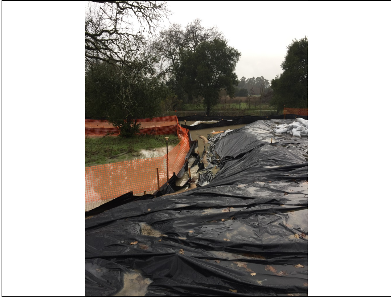
Photo 19: Looking west, at multiple layers of sediment control near southwestern Project boundary.
