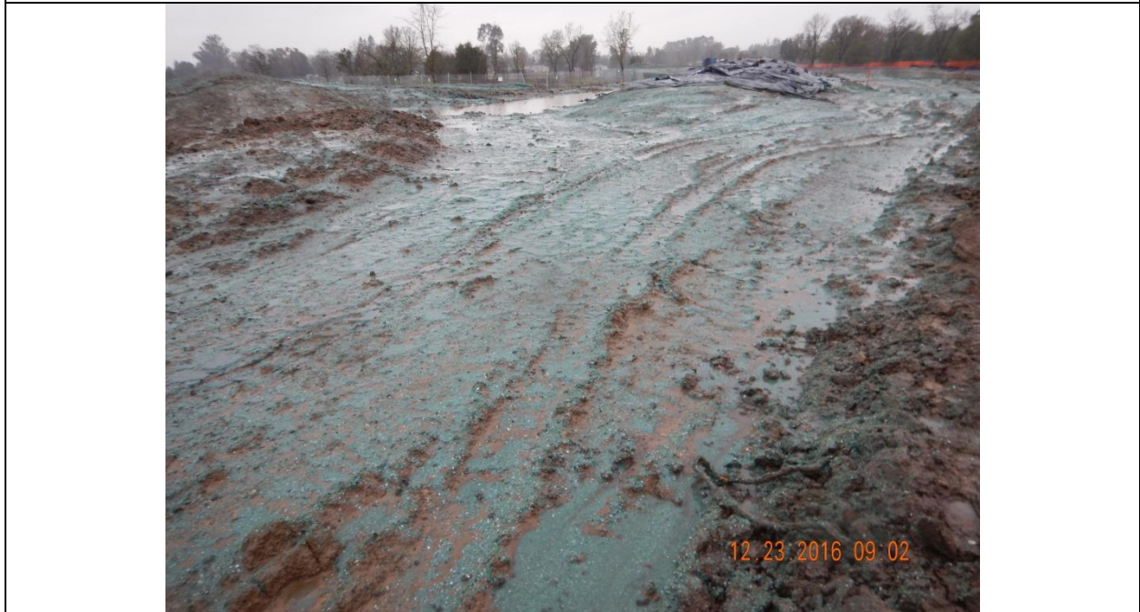
Photo 10: Disturbed area with hydromulch after rainfall.
