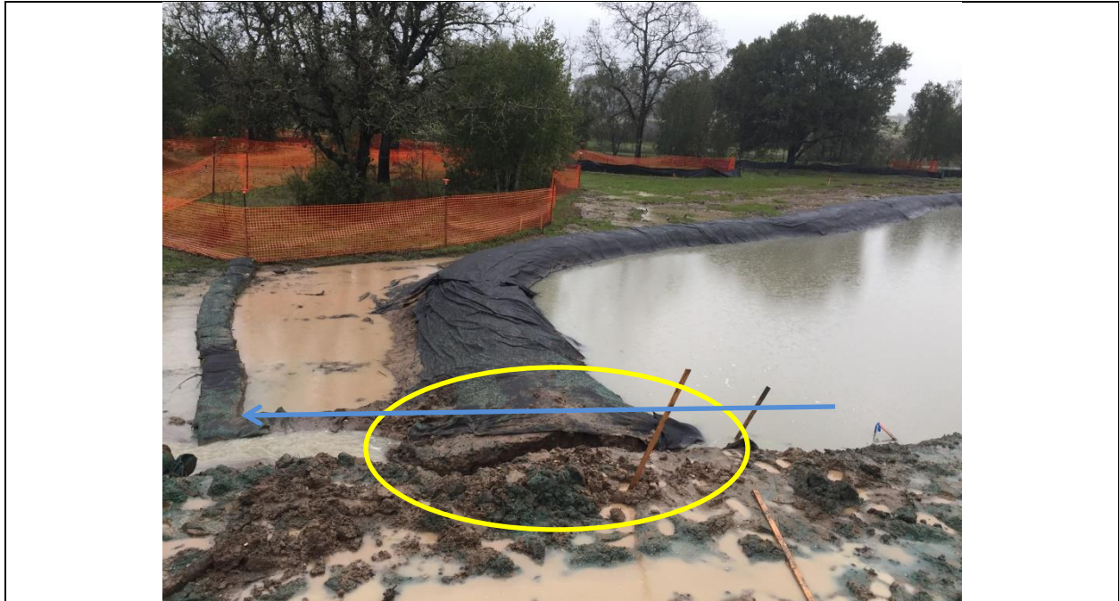
Photo 15. One of the earthen basins failed and storm water was flowing into the next downstream basin. The blue line shows flow direction.
