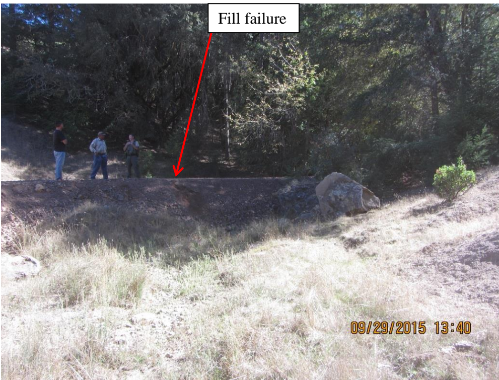
Image 38 looking upstream shows the earthen fills in the stream channel cross sectional area; note the fill failure visible on the road fills and no evidence of a culvert in place to pass stream flows through the earthen fills at GPS 13. (IMG 0316)
