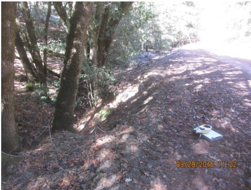
Image 12 shows the road segment at GPS 2. Note the loose earthen material along the road edge adjacent to the stream. (IMG 0252.)
