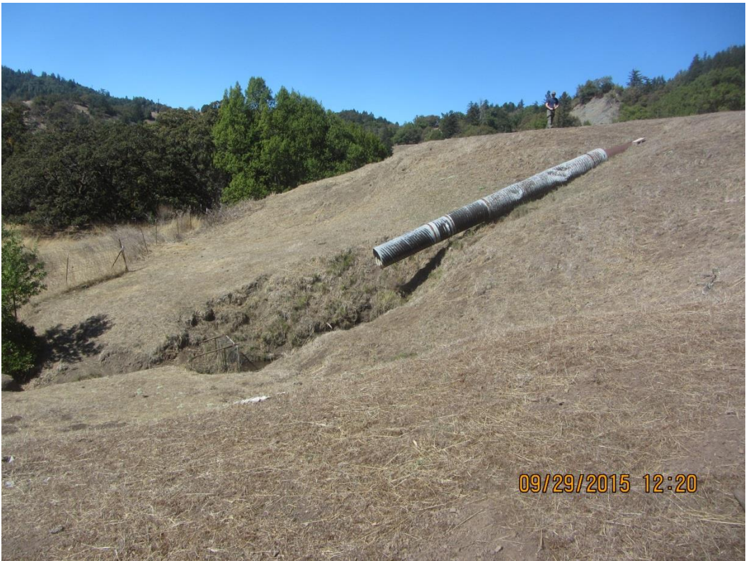
Image 25 provides another view of the shot-gunned spillway culvert outlet for GPS 8. (IMG 0282).
