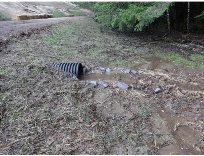
Image 46 shows a recently installed culvert and the sediment deposits at the outlet of the culvert; also note the evidence of possible erosion from slopes above and behind the culvert. (Brandon Rose photo 016).
