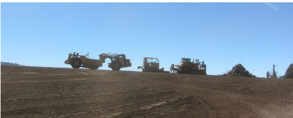
Image 11 shows the equipment observed on site. (IMG 0244 cropped))
