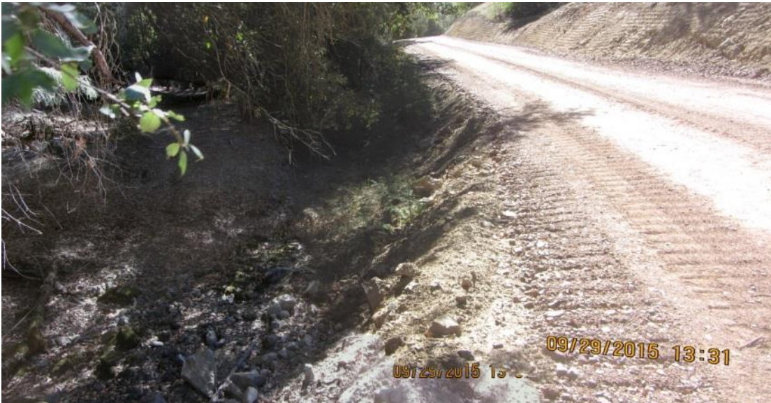
Image 37 shows the recent road construction/reconstruction in and adjacent to the stream that resulted in the placement of earthen fill materials in the stream and in locations where such materials can pass into the stream in the event of rainfall at GPS 13. (IMG 0306_0307stitch)
