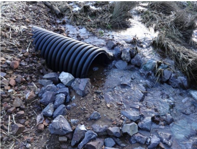
Image 47 shows the outlet of a recently installed culvert delivering into a stream. Note the sediment deposits in the culvert reducing carrying capacity and providing evidence of upstream erosion, sediment delivery and transport. (Brandon Rose photo 118).
