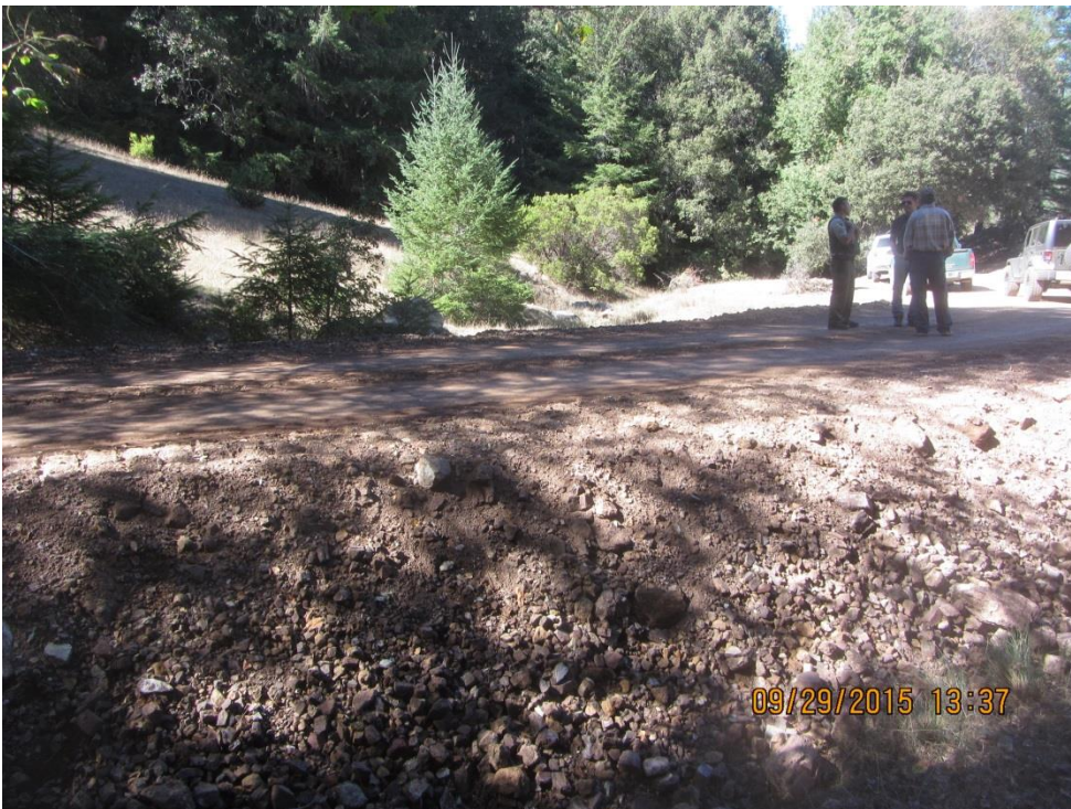
Image 39, looking downstream over the top of the earthen material placed in the stream channel at GPS 13; note the looseness of the materials. (IMG_0314).
