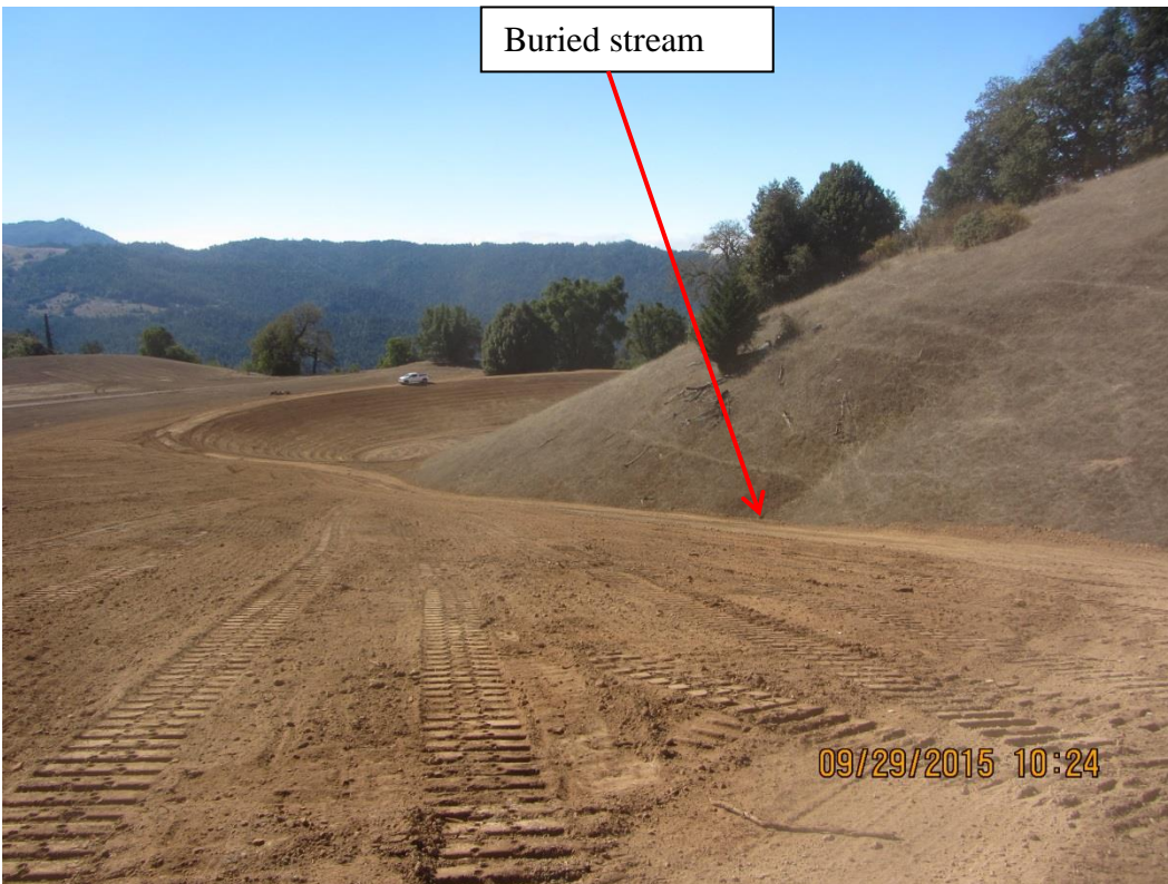
Image 8 shows the pond and the slope contour filled with loose soils leading to the pond from above. (IMG 0208)
