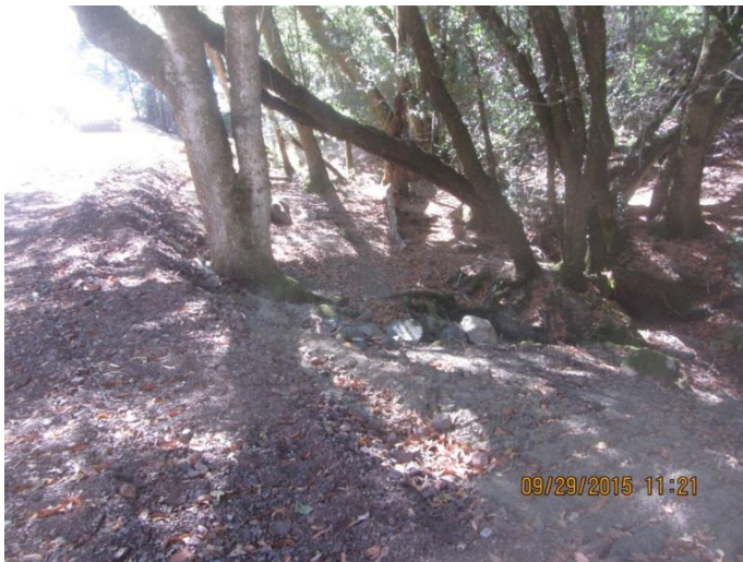
Image 14 shows the stream crossing at the downstream road edge at GPS 3. (IMG 0249)
