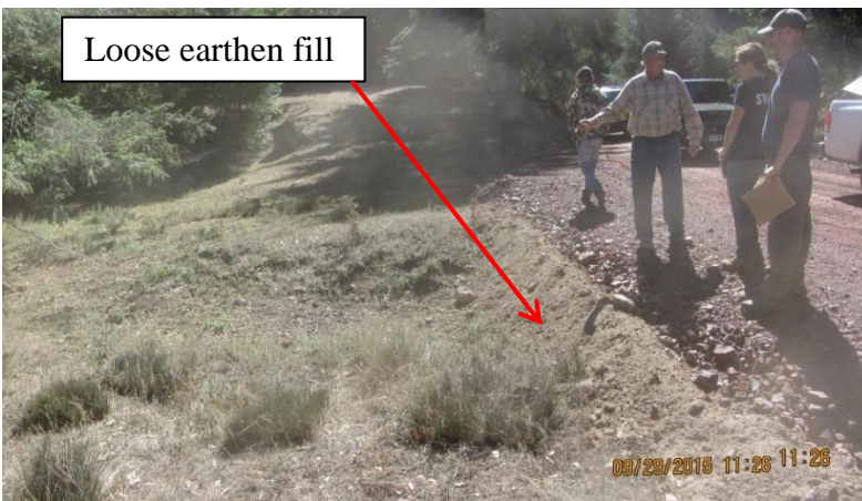
Image 15 shows the road fill in the stream channel on the east (upstream) side of the road at GPS 4. Note there is no culvert visible in the road fills placed into the stream channel on this side of the road. A culvert was visible on the downstream side of the crossing. (Stitch of 0253 and 0254)
