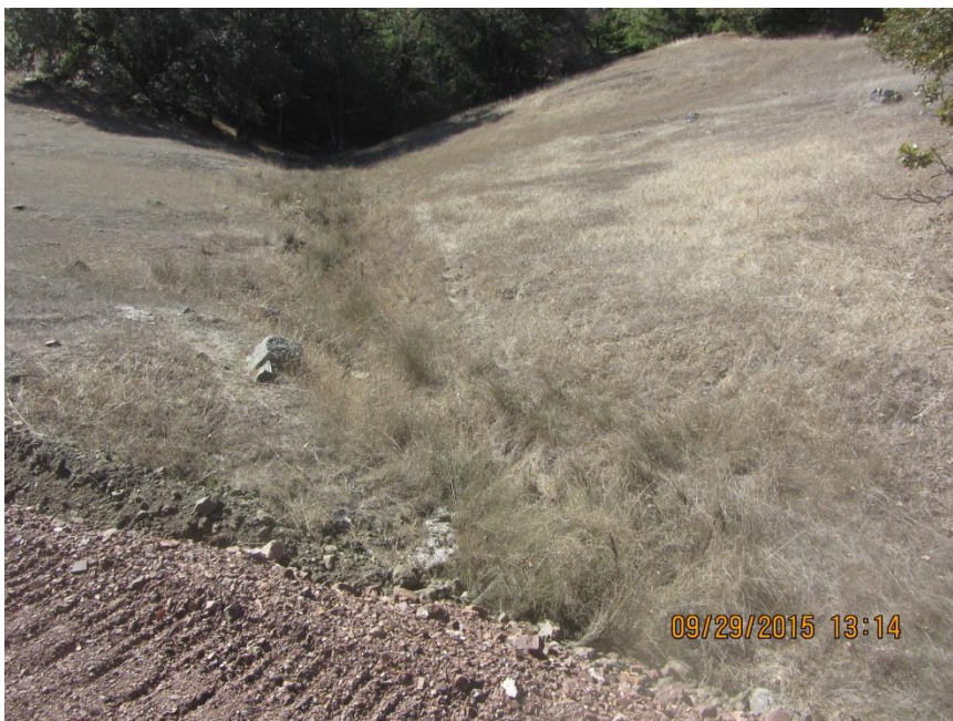
Image 32 shows the upstream channel at GPS 11 as it intersects the constructed/reconstructed road. (IMG_0294)
