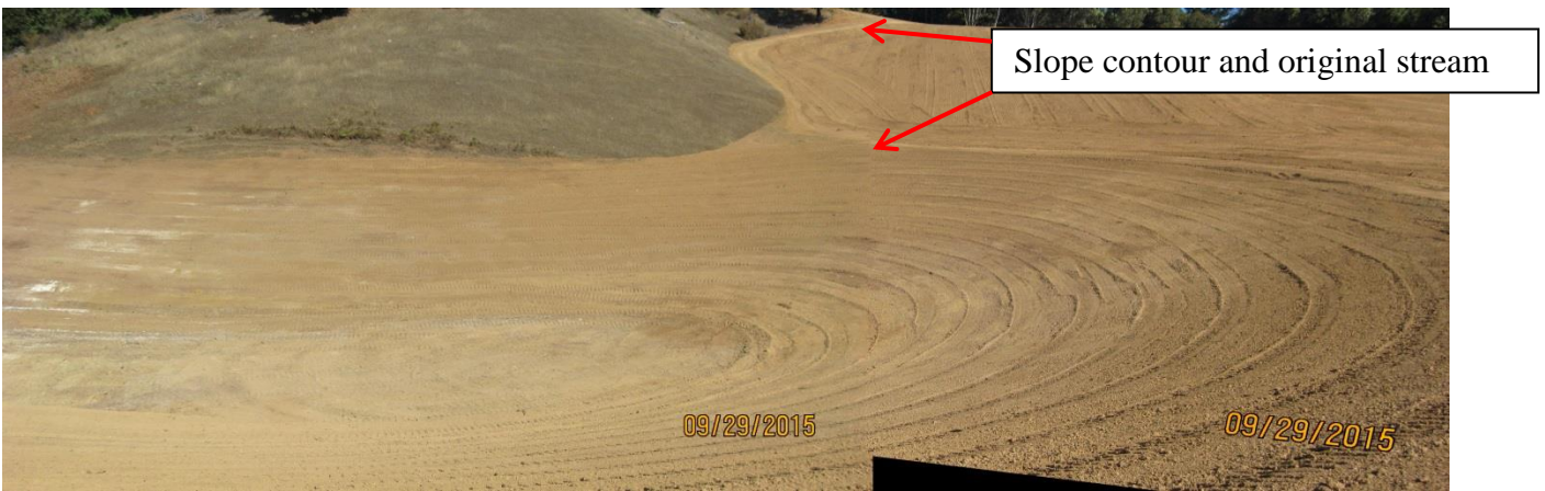
Image 7 shows the hole excavated to extract rock or to develop a pond. Note the stream originally followed the slope contour and flowed down to the meadow area below the pond. Here the drainage has been interrupted and directed to the pond. In addition, the original stream channel has been filled with loose earthen material because of the grading. (Division of Water Rights inspection photos 0587 and 0589 stitched together.)
