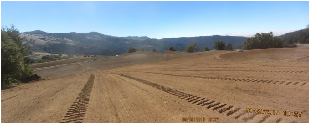
Image 10 shows an overview of the grading; the pond is visible to the far right. (IMG 0209-0212 and 0214 stitch).
