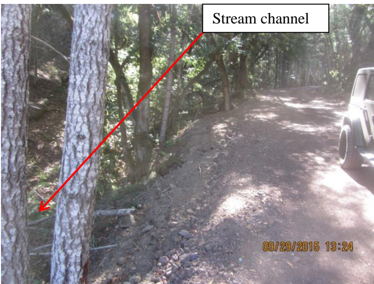
Image 36 shows the perched fills directly above the stream channel south of stream crossing 8 (GPS 12). (IMG_0303)
