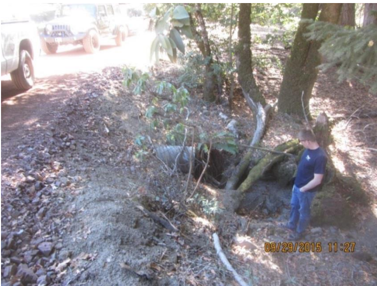
Image 16 shows the downstream side of the stream crossing at GPS 4. Note the erosion below the culvert outlet, possibly as a result of the drop at the culvert outlet and/or as a result of the culvert being undersized and forcing high flows through at increased velocities. (IMG 0257)
