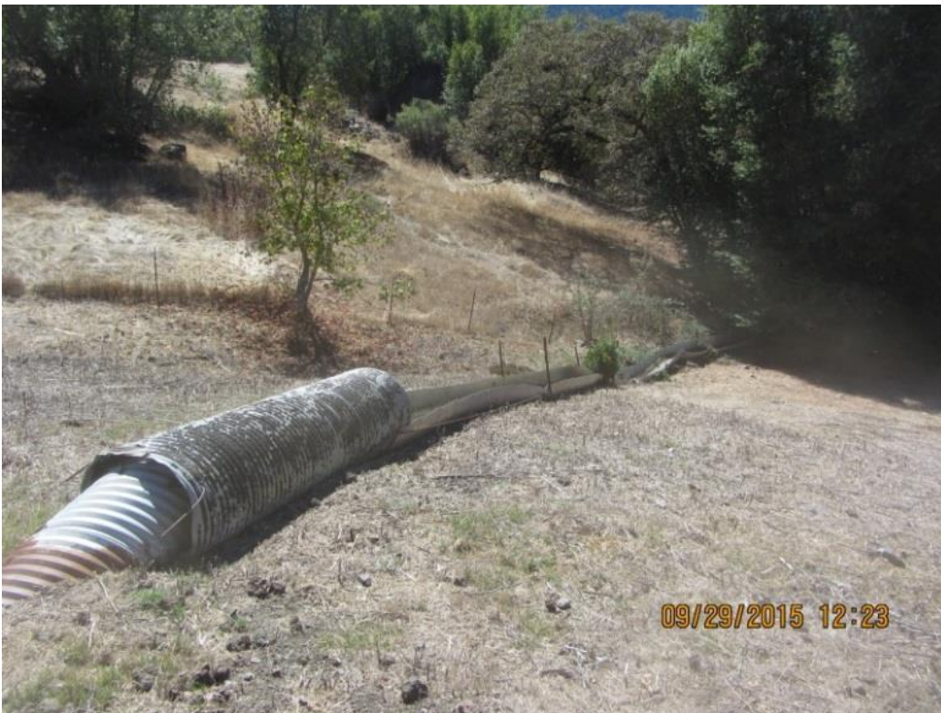
Image 28 shows the outfall from the smaller pond (GPS 9). Note the culvert and half pipe do not appear to be structurally sound; however, the half pipe was carrying flows during the inspection. (IMG_0284)
