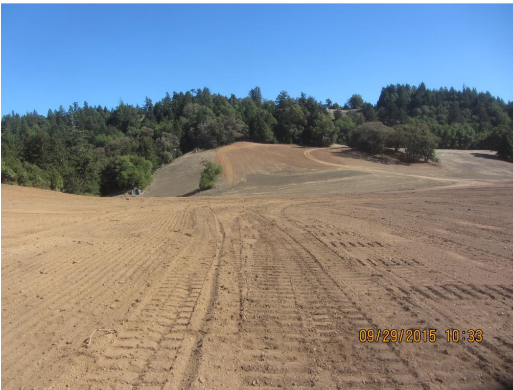
Image 9 shows the slope below the pond looking south at approximately the location where I would expect to see the stream visible in images 4 and 5 flowing to the east across the slope and down to the main stream to the north. (IMG 0219)
