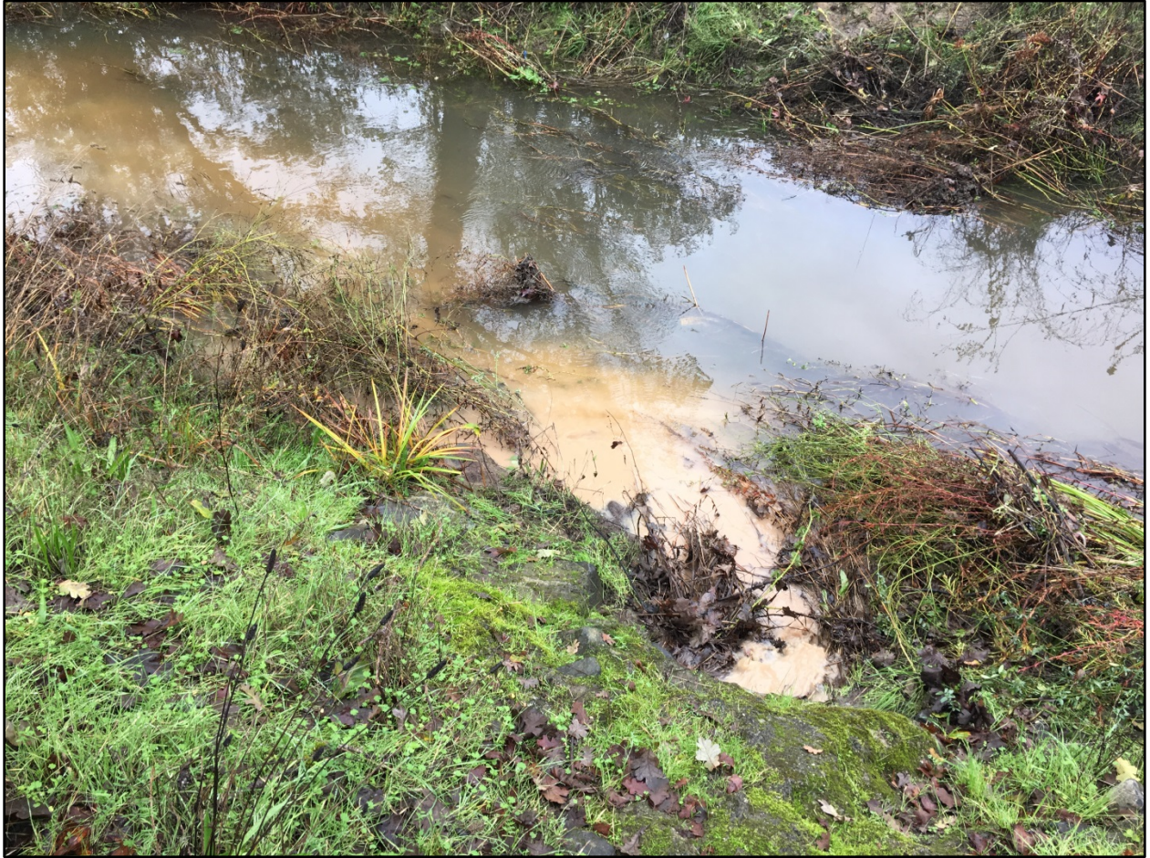
Photo 9. Sediment-laden water discharged into the drop inlet to a culvert and into Peterson Creek. Photo was taken facing west on November 20, 2016, at 09:28.
