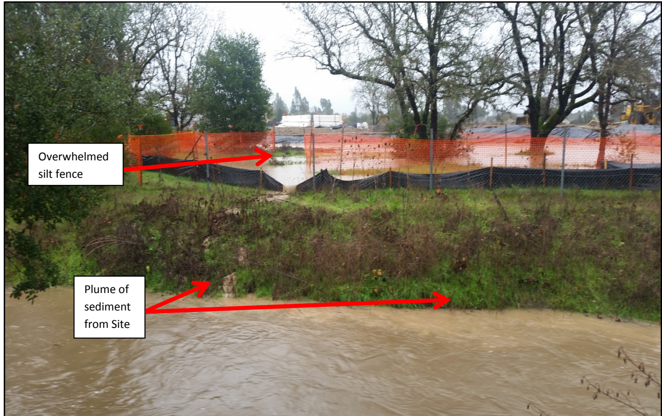
Photo 15. Sediment-laden storm water runoff from Site discharged into Peterson Creek. This area was also overwhelmed by the overflow of water in the containment area. Photo was taken facing southeast at 13:27.
