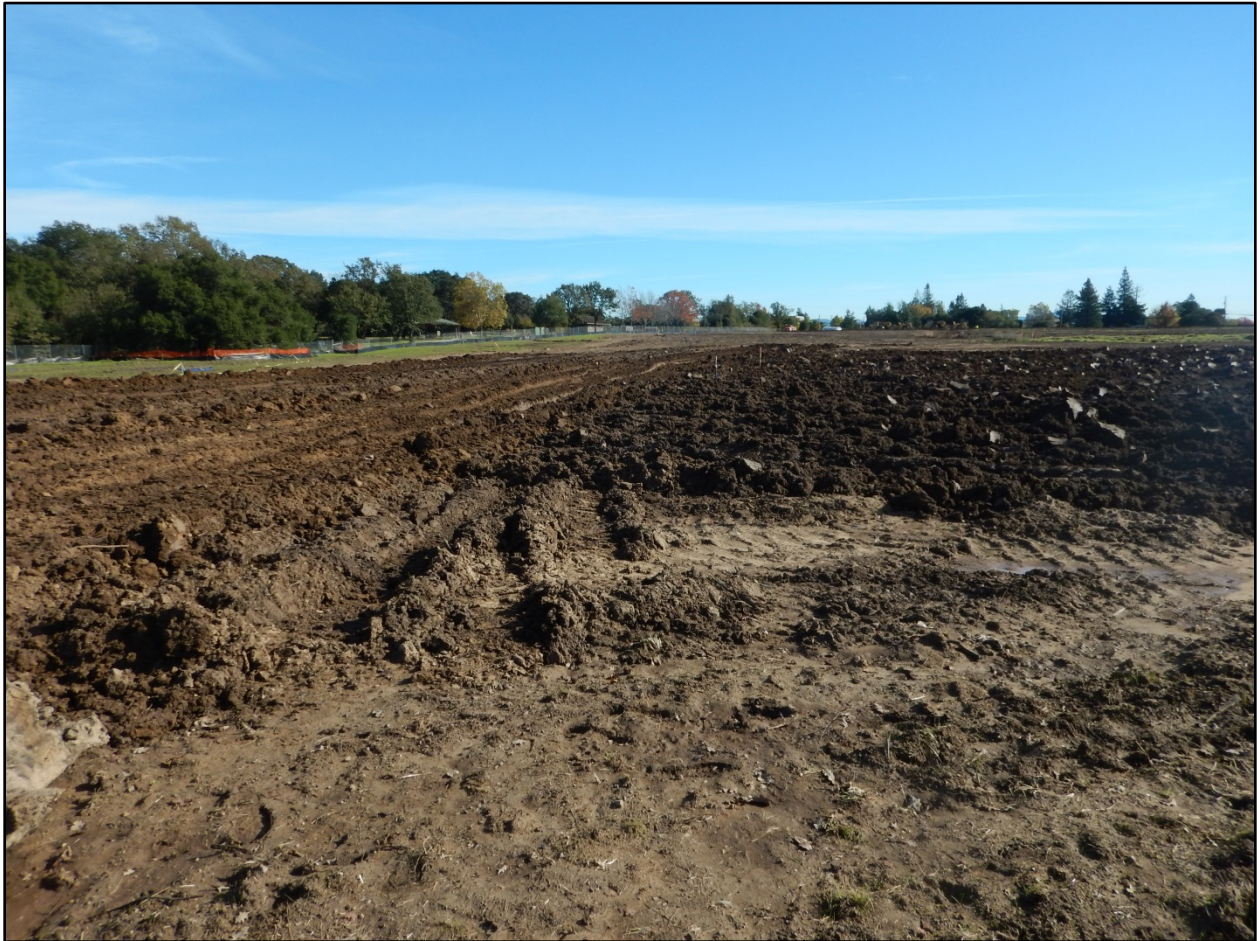
Photo 3. Conditions of the Site during the inspection. Photo depicts around one third of the Site. Staff did not observe any erosion controls in place to prevent sediment from being dislodged and discharged in storm water runoff. Sediment controls that were in place were overwhelmed and ineffective during late October, 2016, rains. Photo was taken standing adjacent and east of the preserved wetlands, facing northeast at 11:01 on November 3, 2016.
