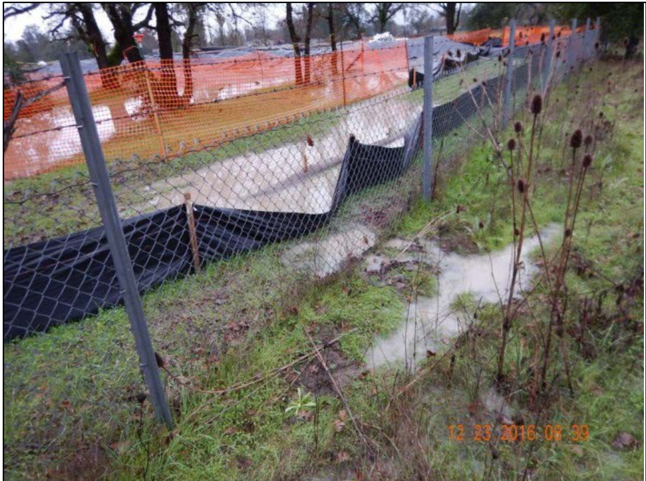
Photo 30. Peterson Creek discharge location 1. It appeared that storm water was passing underneath the silt fence. This discharge location appears to correspond with discharge sampling location #1 as provided in the 12/23/16 Sampling Field Log sheet.
