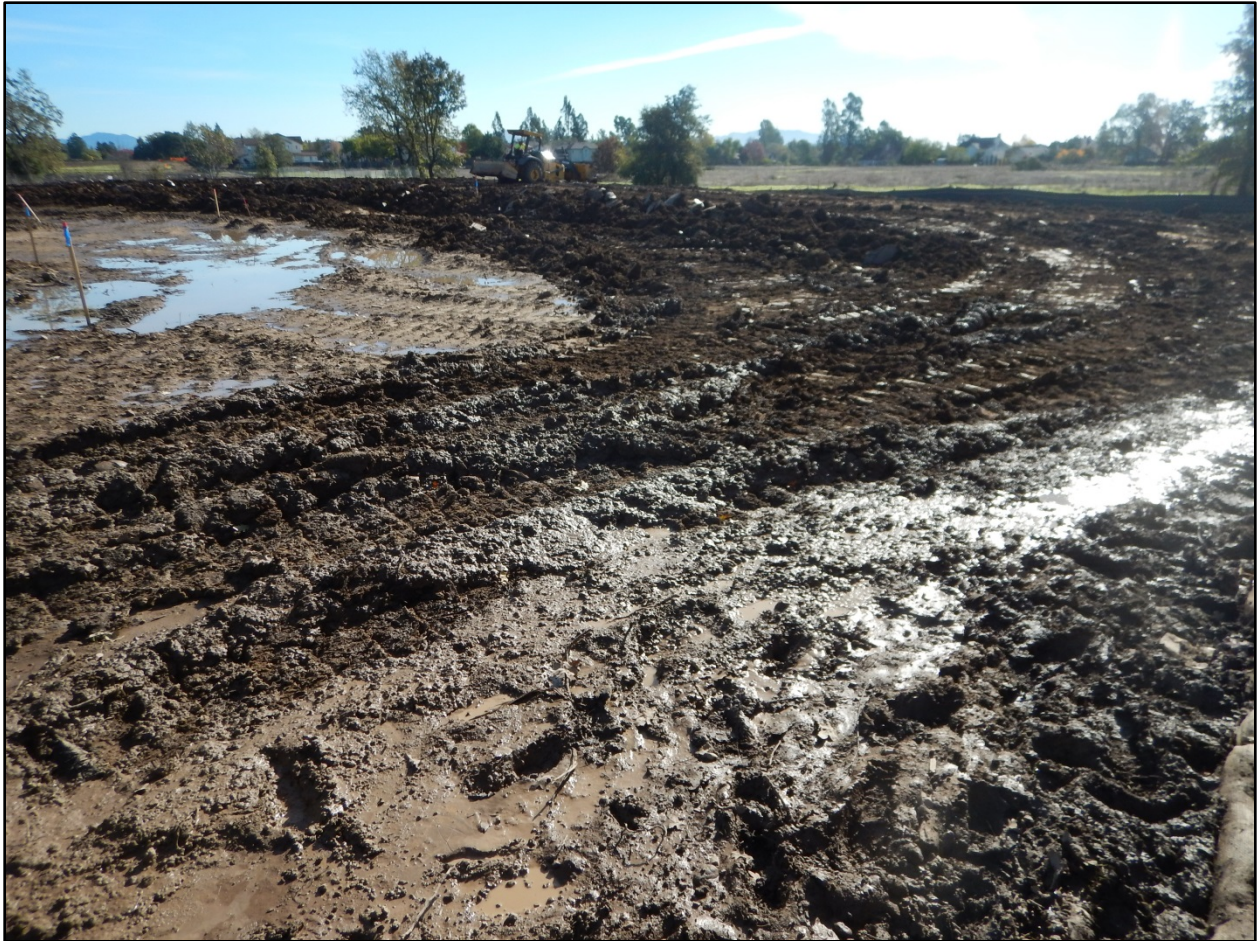
Photo 4. Conditions of the Site near the western boundary. Staff did not observe any erosion controls in place to prevent discharges of sediment. Soil was highly saturated and sediment-laden puddles of water remained on most of the Site after a couple of days of dry weather. Photo was taken facing southeast at 11:05 on November 3, 2016.
