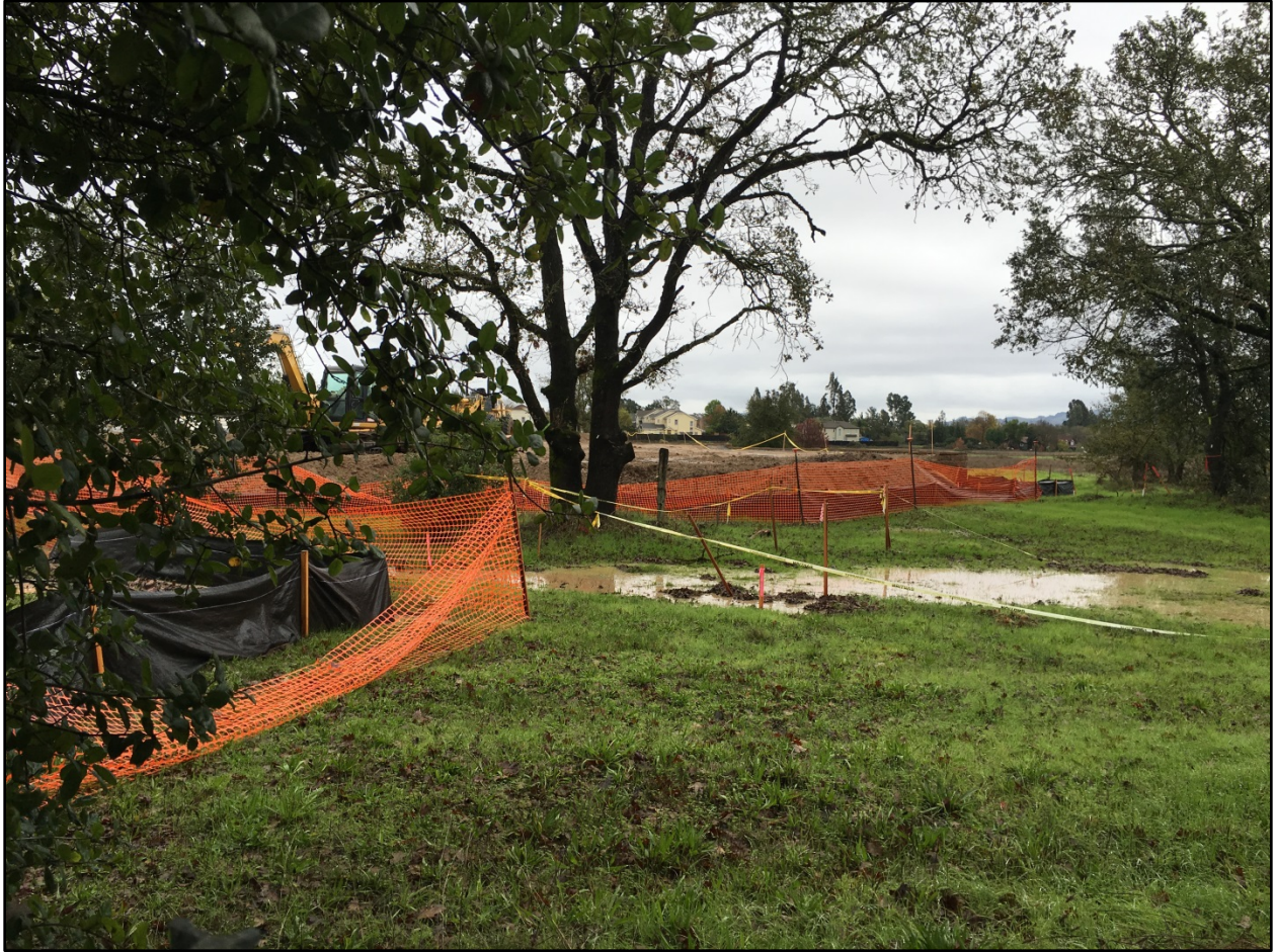
Photo 7. Sediment-laden water discharged through BMPs on the western boundary of the site adjacent to Peterson Creek. Photo was taken facing southeast on November 20, 2016, at 09:25.
