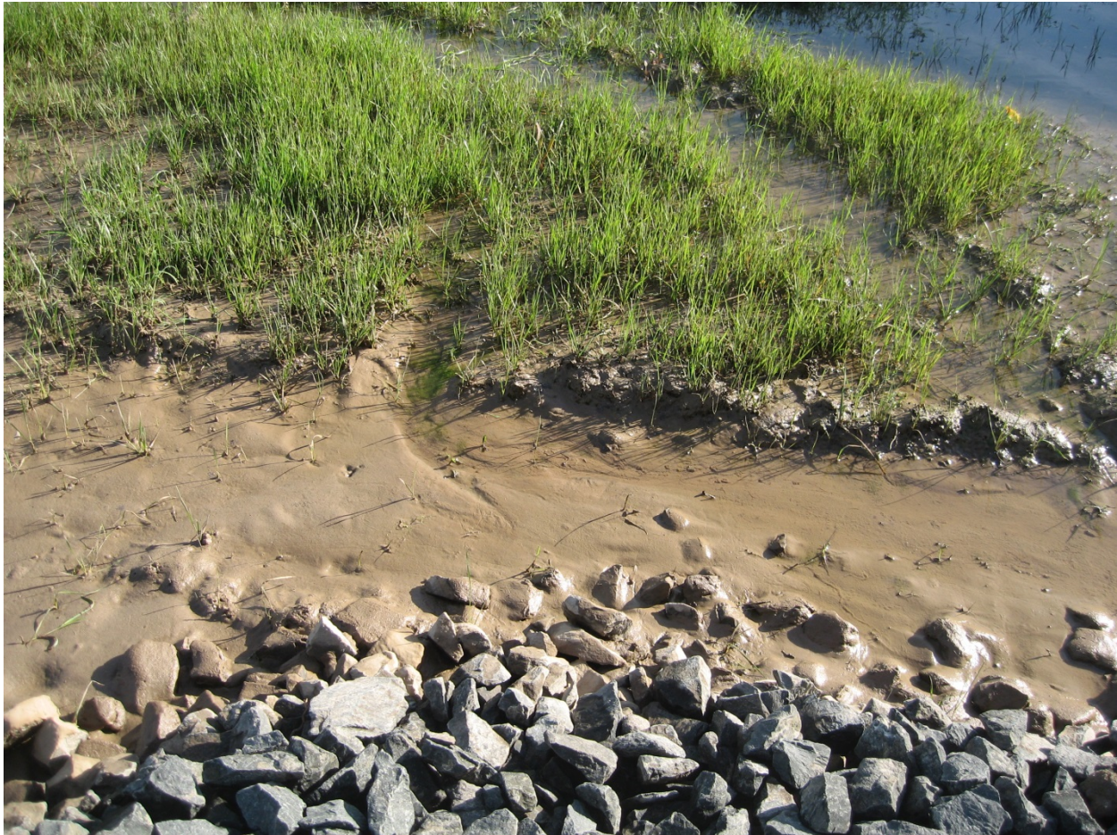
Photo 27. Deposits of fine sediment in the flow path to the MS4 inlet represent evidence of a previous discharge. The inlet is located around 10 feet to the right of the photo. Deposited sediment and debris was observed closer to the inlet, but the lighting at the time of the photograph did not allow for a clear image. Photo was taken at 11:44.
