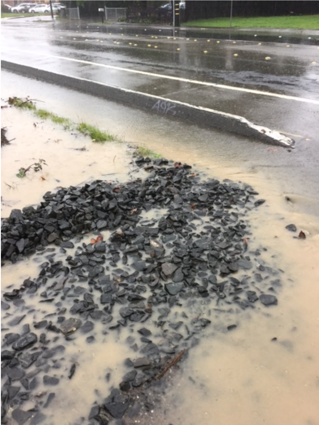
Photo 21. Sediment-laden discharge from Site's entrance to Fulton Road. Discharge occurred due to lack of adequate BMPs on construction entrance. Photo was taken by Mr. Gary Morris of LJP Construction Services during his inspection on December 15, 2016.
