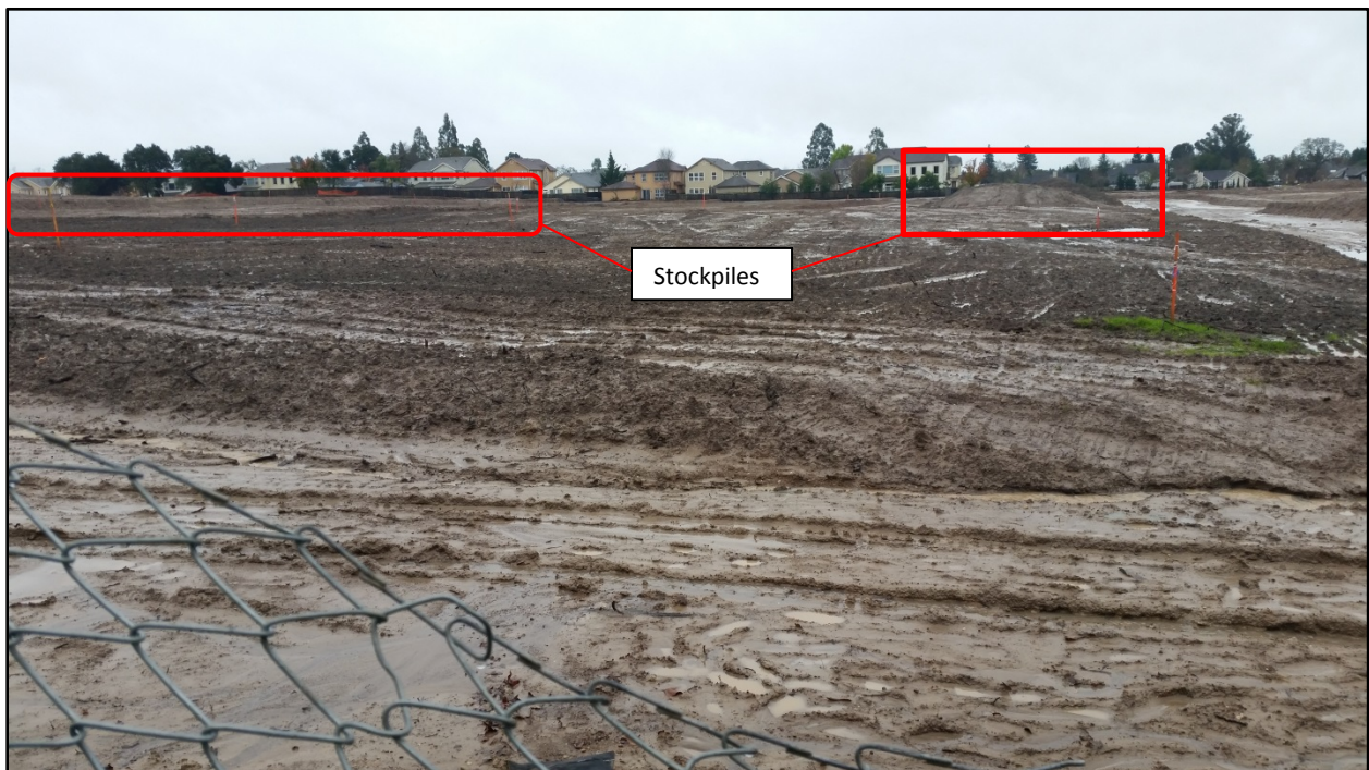
Photo 19. Conditions of the Site at the time of the discharge. Note the lack of erosion controls and the stockpiles lacking coverage and berms/perimeter controls (Construction General Permit, Attachment D.B.1.b.) Photo was taken at northern boundary of project facing roughly south at 13:54.
