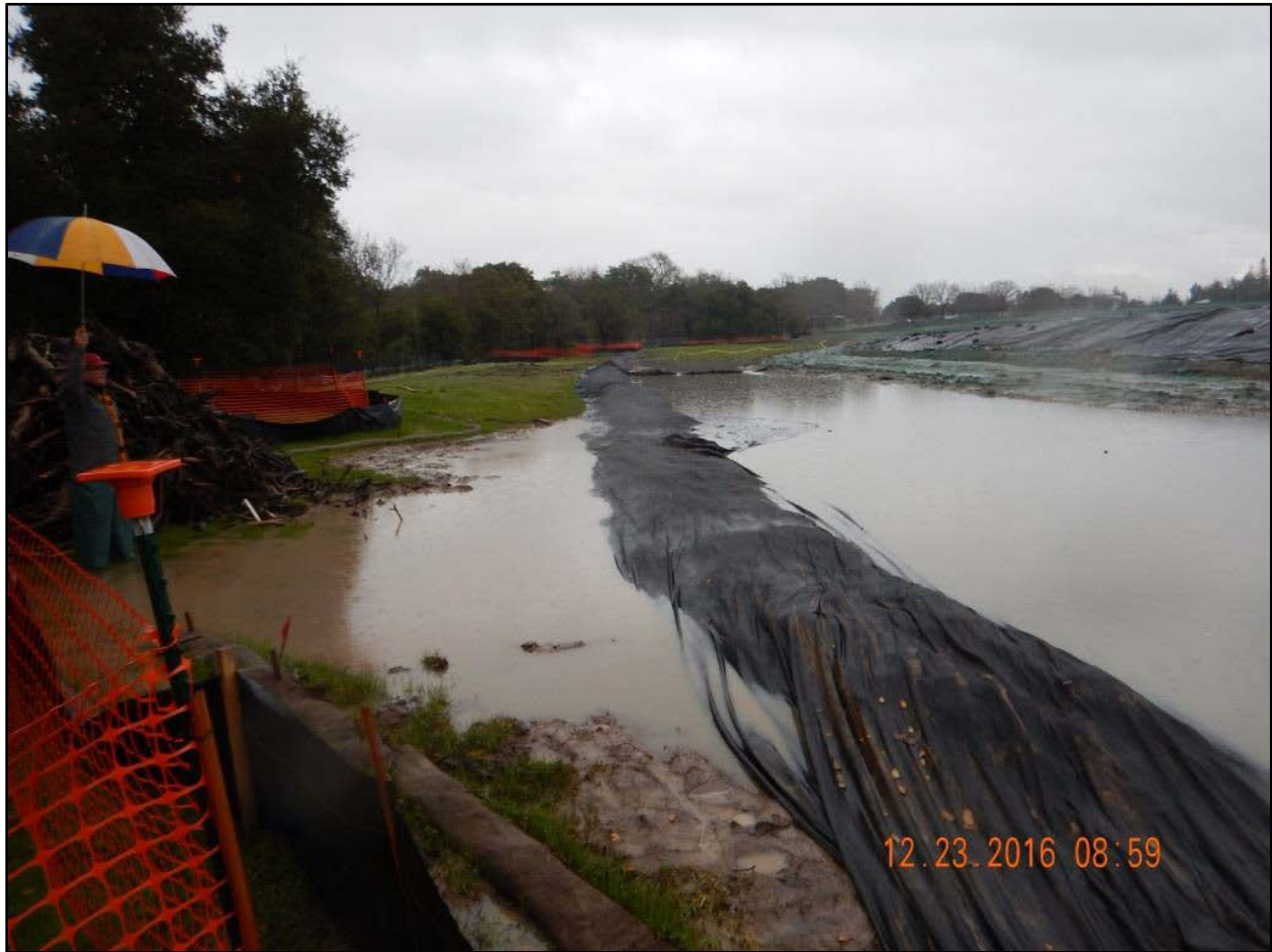
Photo 34. Earthen berm covered with filter fabric. Looking north. Peterson Creek is approximately 40 feet to the left.
