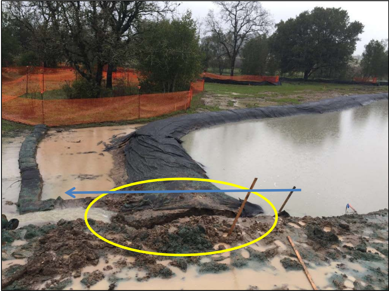
Photo 36. One of the earthen basins failed and storm water was flowing into the next downstream basin. The blue line shows flow direction.
