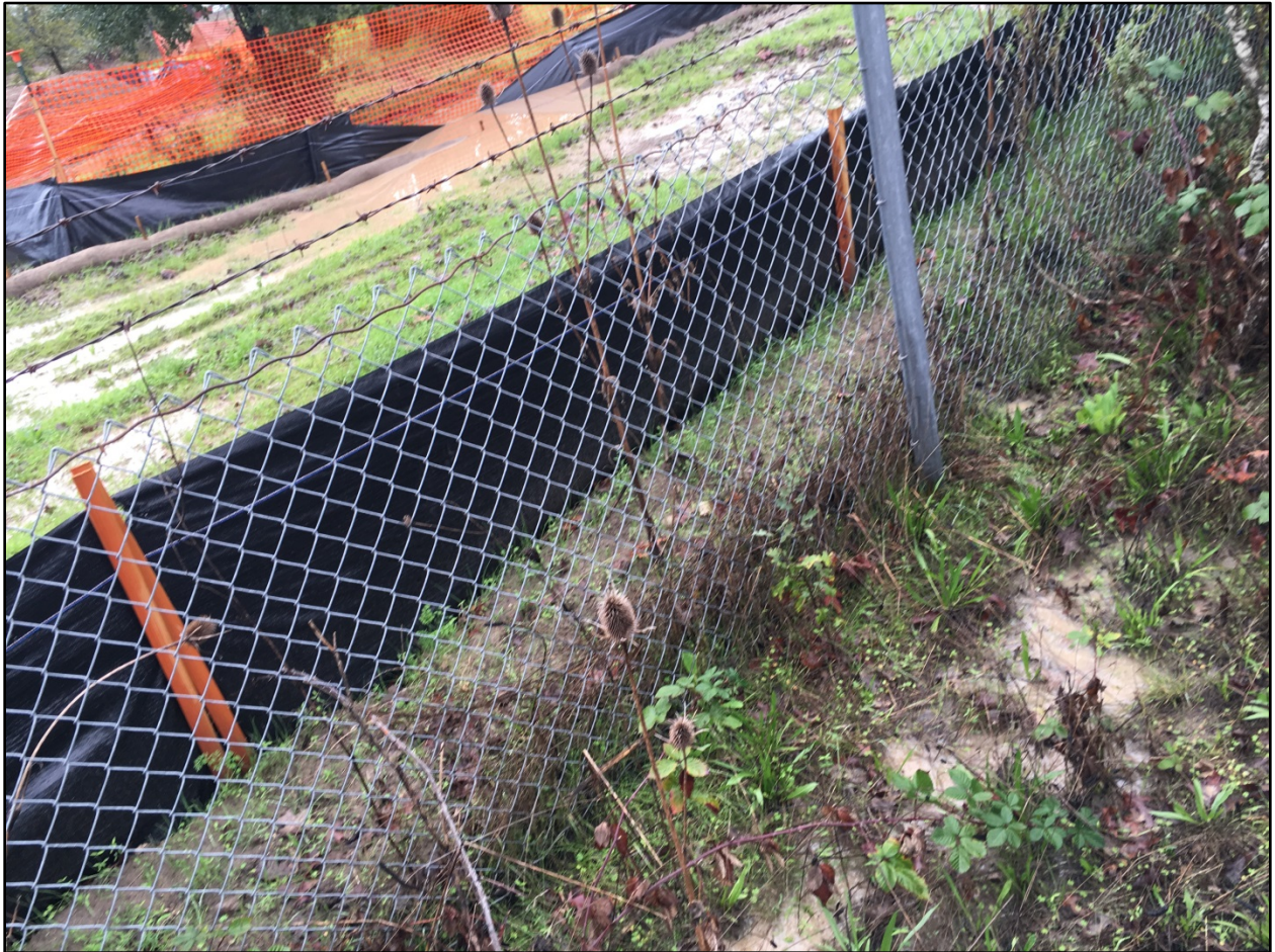
Photo 12. Sediment-laden water seeped through silt fencing on the western boundary of the Site as a result of highly-saturated exposed soil. Silt fencing (in the background of the photo) was breached by a large volume of sediment-laden water. Photo was taken facing southeast on November 20, 2016, at 09:22.
