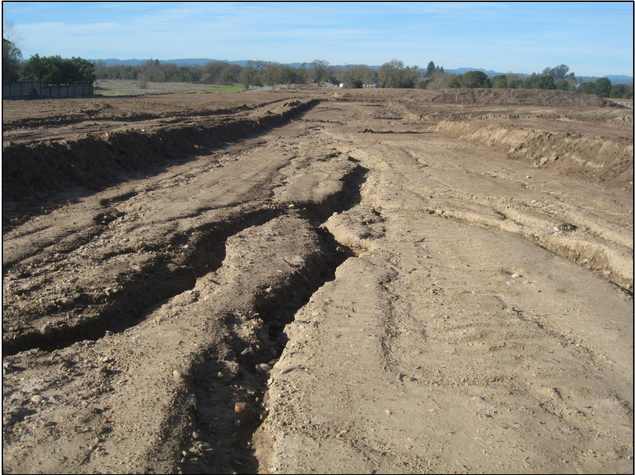
Photo 22. Gullies formed along the one of the roads on the southern portion of the project. The gullies ranged from one to two feet wide and deep along this and other roads. The gullies formed as a result of concentrated flow on the exposed soil lacking erosion and adequate sediment controls. Photo was taken facing west at 11:48.
