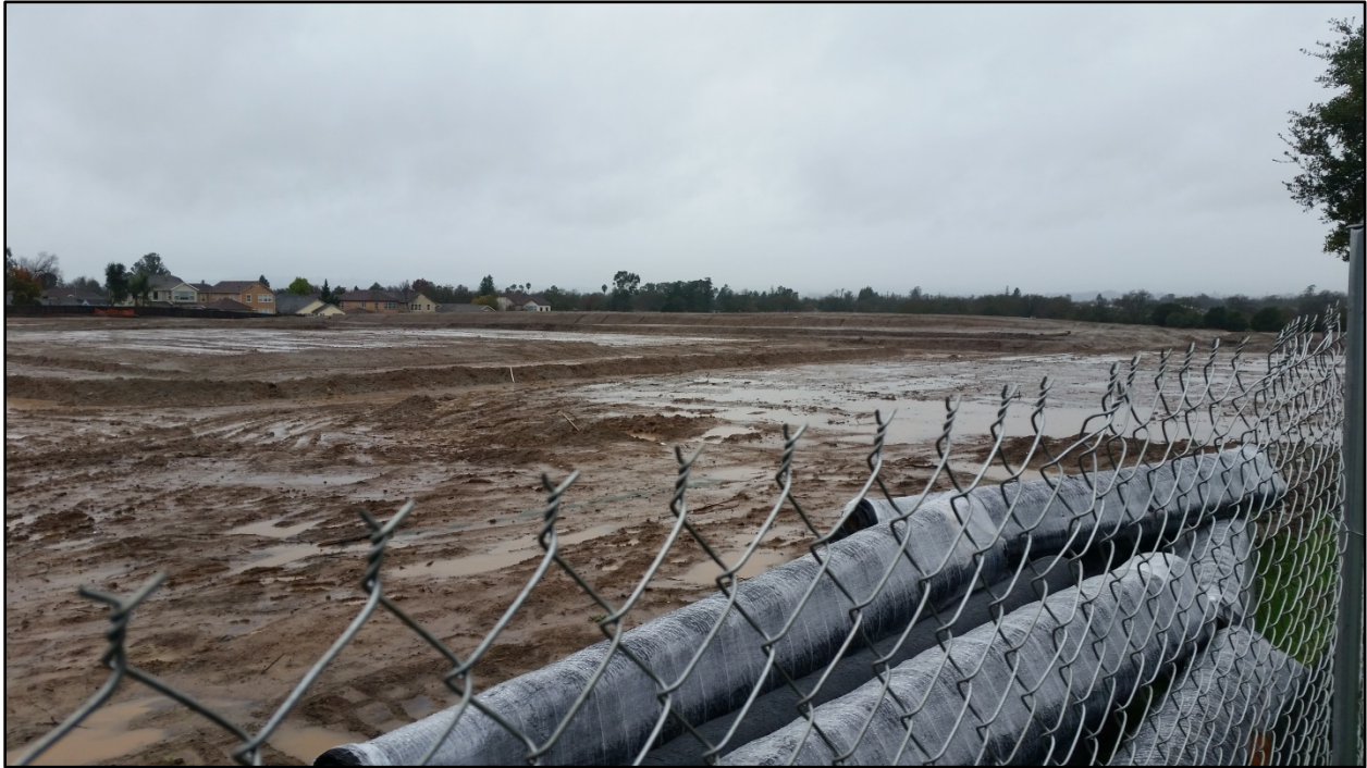
Photo 18. Conditions of the Site at the time of the discharge. Note the lack of erosion controls. Photo was taken at the northern boundary of the Site facing southwest at 14:02.
