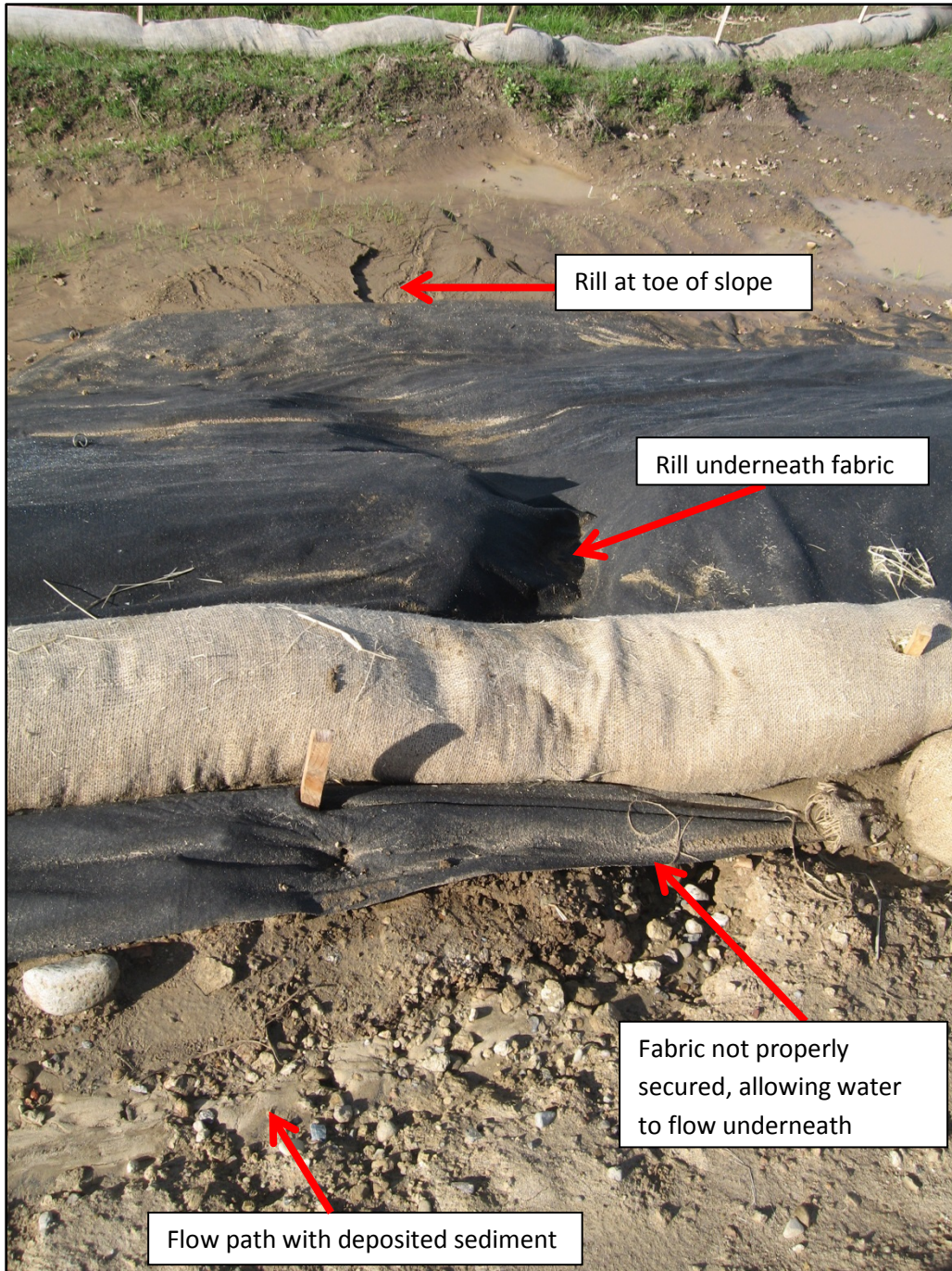
Photo 25. Inadequately secured fabric on slopes of the perimeter of disturbed area allowed for rilling and sediment transport during rain events. If fabric was properly secured, water would not be allowed to flow underneath the fabric, preventing erosion and sediment transport. Photo was taken east of the preserved wetland's eastern boundary at 12:04.
