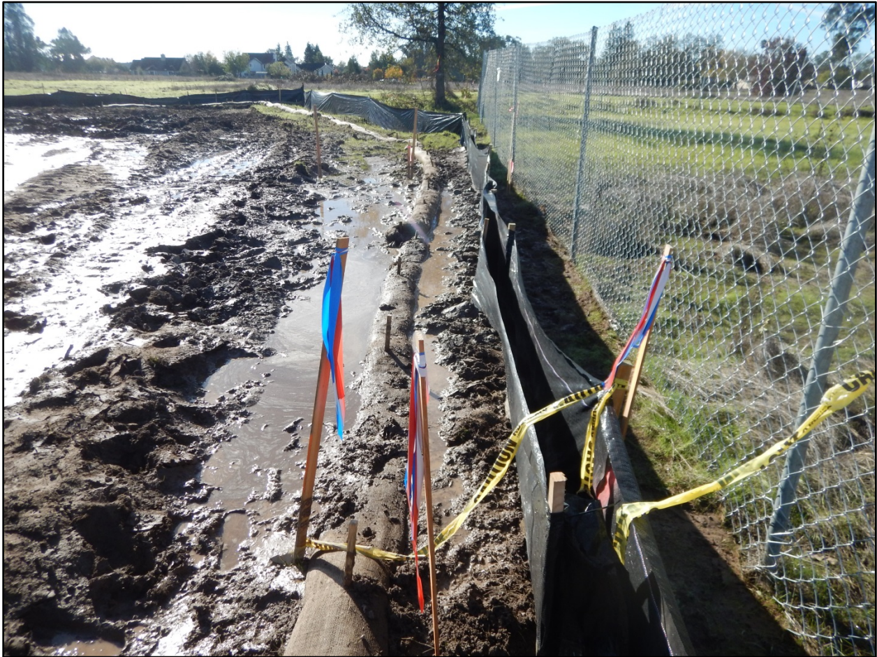
Photo 5. Conditions of the Site adjacent to the east side of the persevered wetland. In order to prevent discharges of sediment into the wetland in future rain events, the sediment controls needed to be maintained immediately. Photo was taken facing roughly south at 10:49 on November 3, 2016.
