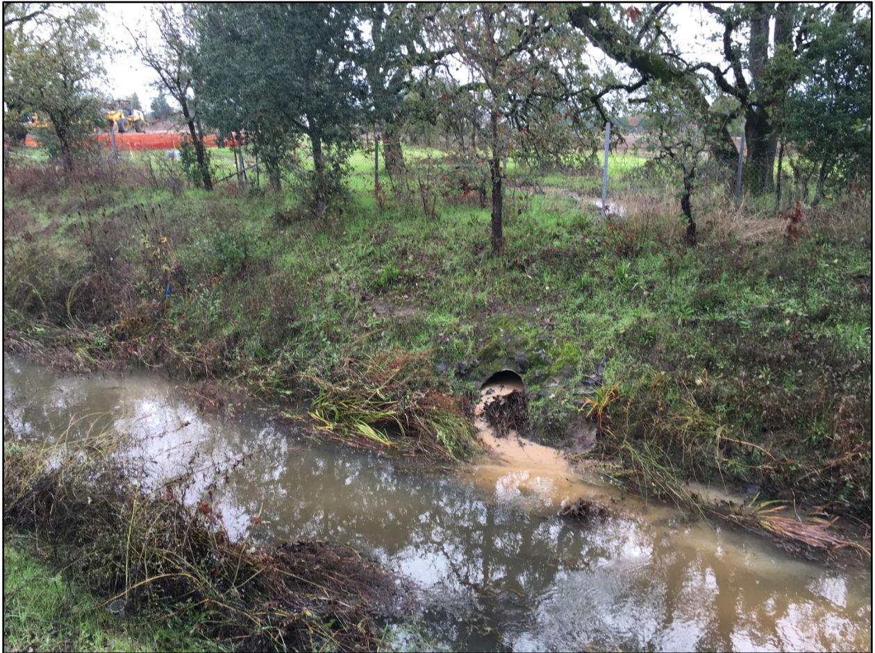
Photo 10. Sediment-laden water discharged from the southwestern boundary of the site (see orange fencing in background) to a swale on the adjacent property to the south, and into a culvert to Peterson Creek. Photo was taken facing east on November 20, 2016, at 09:13.
