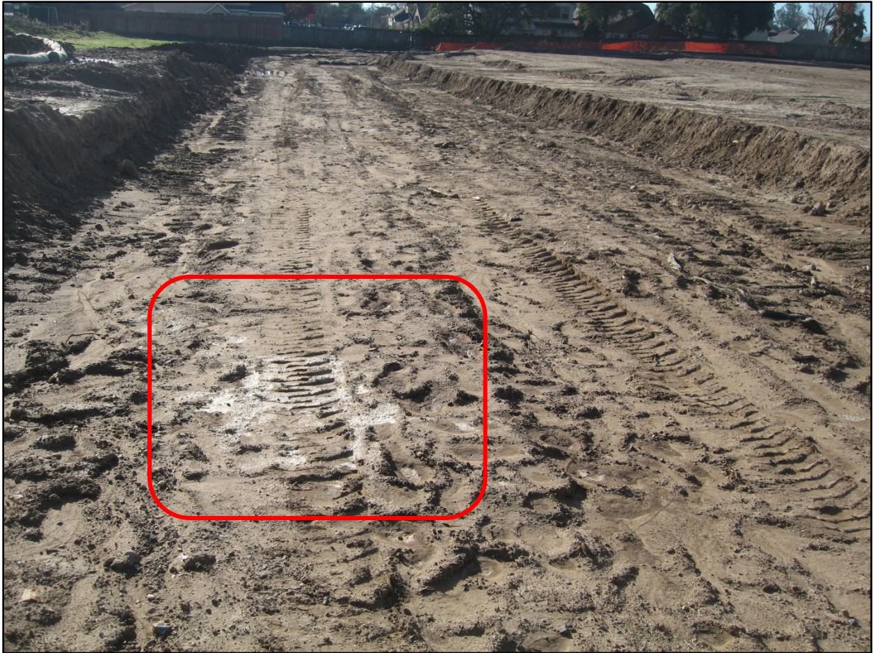
Photo 28. The red rectangle outlines remnants of the bonded fiber matrix (BFM) that Mr. Fortney said was applied prior to the December 15, 2016, rain event. Photo was taken on the eastern-most road on the Site. Note the lack of erosion and sediment controls. Photo was taken facing south at 11:36.
