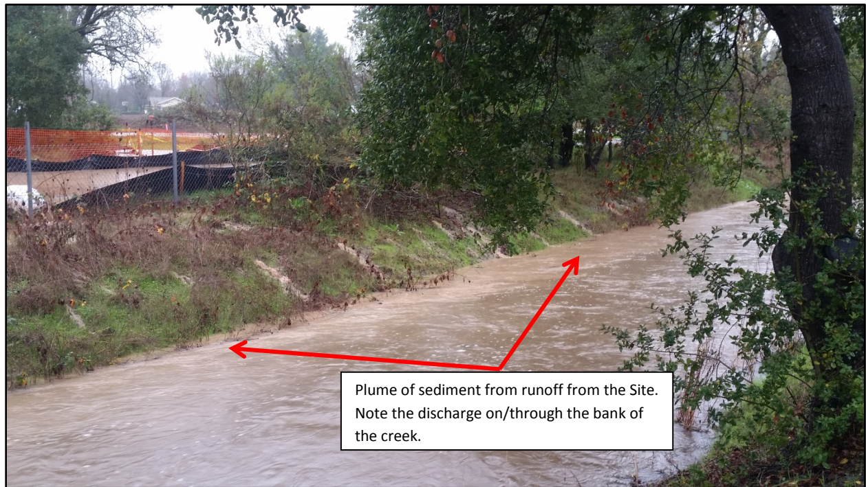
Photo 16. Sediment-laden storm water runoff discharged from the Site into Peterson Creek along western boundary. Discharges were a result of overwhelmed BMPs and highly-saturated, unprotected soils, which allowed the water to seep under BMPs and through the bank of the creek. Photo was taken facing southeast at 13:28.
