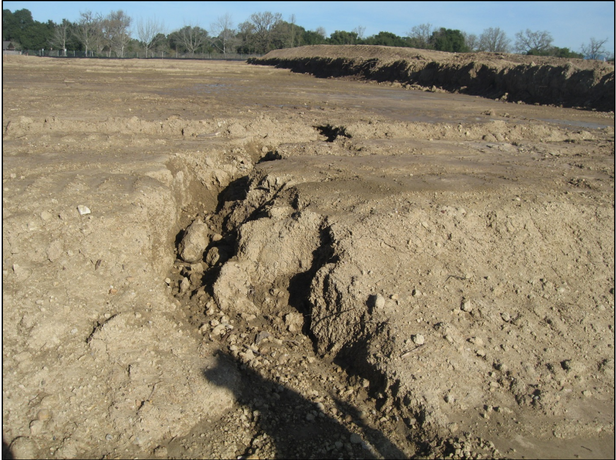
Photo 23. Gullies formed on the slopes of the housing pads as a result of concentrated flow on the soil lacking erosion and sediment controls. Gully depicted in photo ranged from one to three feet wide and one to feet deep. Photo was taken facing roughly north at 11:47.
