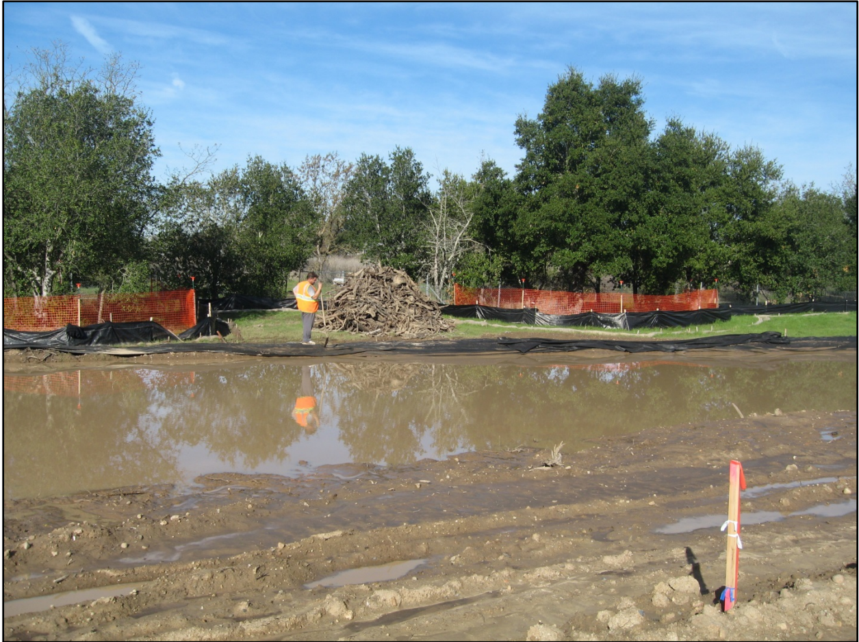
Photo 26. Storm water containment area along western boundary of Site adjacent to Peterson Creek (on the other side of the orange fencing). During the inspection, the containment area was filled near capacity with sediment-laden water. During the previous rain event, the containment area was overwhelmed by the volume of storm water runoff, and water flowed onto the adjacent vegetated area and into the creek. The containment area is not properly designed per the California Storm Water Quality Association's (CASQA) BMP standards, and therefore is not sized adequately to detain the volume of runoff expected from its drainage area, and poses a threat to discharge in future rain events. Photo was taken facing northwest at 12:07.
