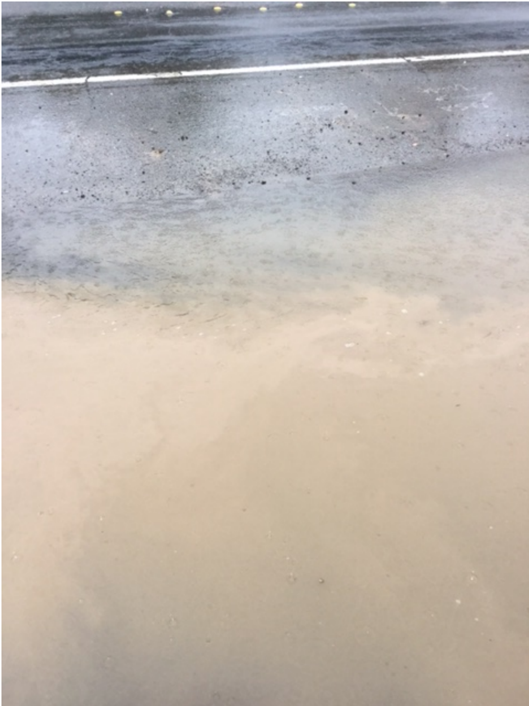
Photo 20. Sediment-laden discharge from Site's entrance to Fulton Road. Discharge occurred due to lack of adequate BMPs on construction entrance. Photo was taken by Mr. Gary Morris of LJP Construction Services during his inspection on December 15, 2016.
