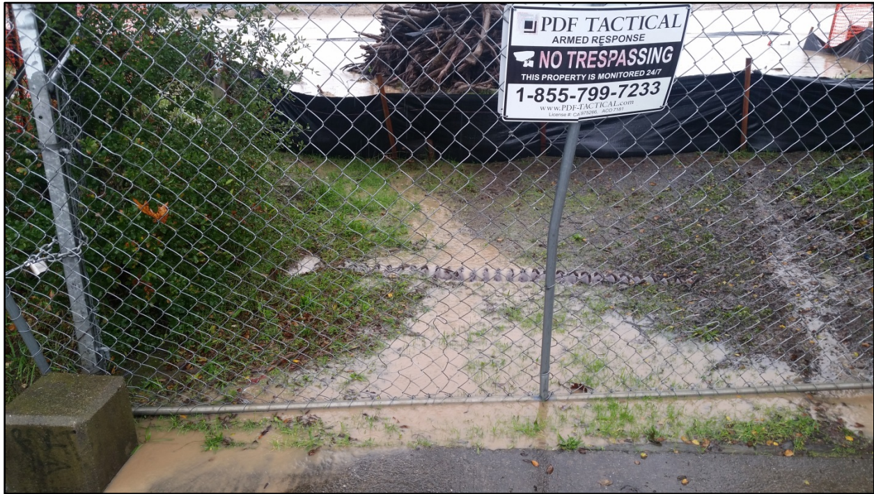
Photo 13. Sediment-laden storm water runoff discharged from the Site along the western boundary at the bridge over Peterson Creek as a result of the lack of adequate best management practices (BMPs). The runoff flowed under the bridge and into Peterson Creek. Photo was taken facing southeast at 13:24.
