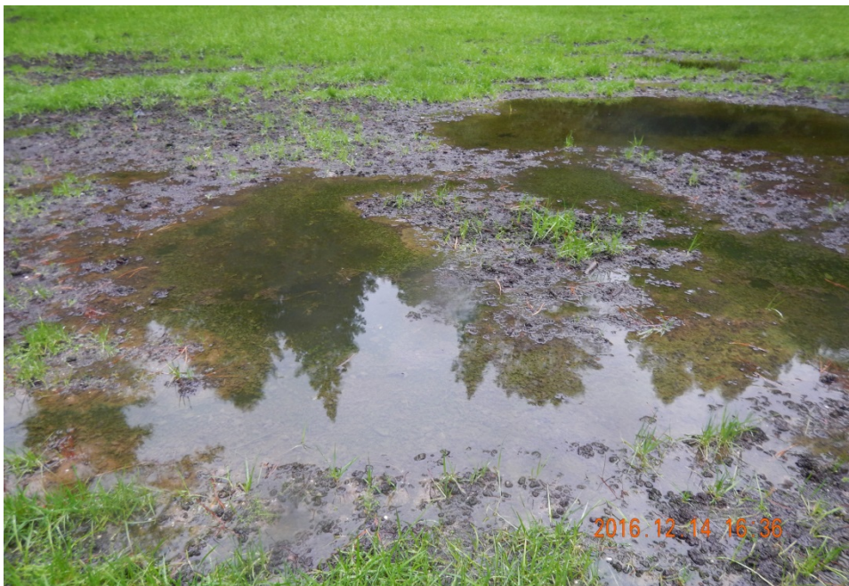
Photograph 5. Redway CSD – 12/14/16: Discoloration of water on the forested property northwest of the treatment plant. Photograph by Cathleen Goodwin, Regional Water Board staff
